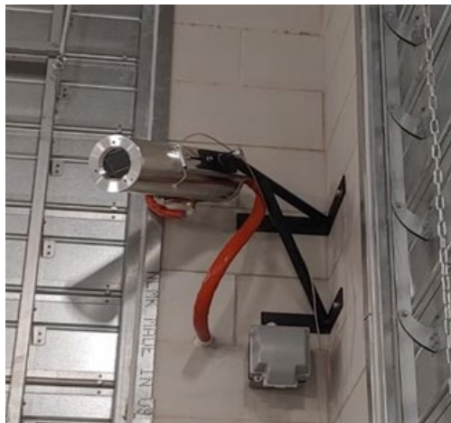
Figure 17. Thermal Imaging Camera in Enclosure
