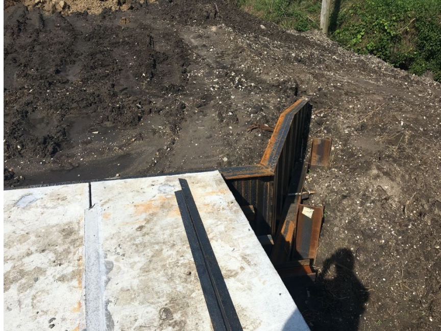
Figure 1.6 An example of a county bridge in Nebraska with solid planks and sheet pile abutments.
