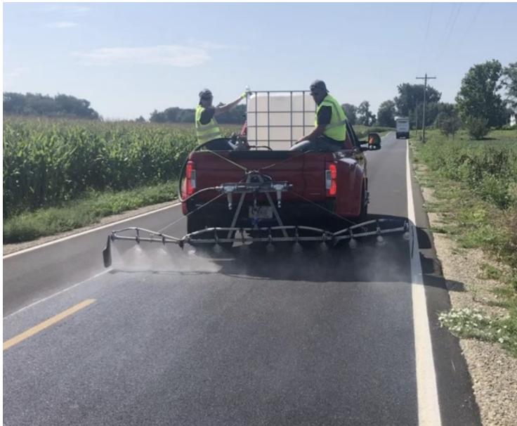
Figure 3 Bio fog seal application
