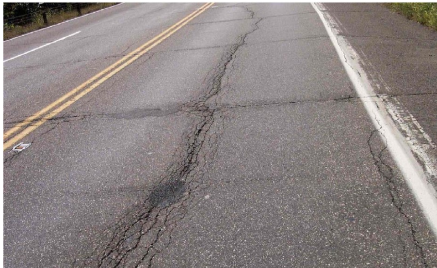
Figure A.6 High Severity Longitudinal Crack (MnDOT, 2011)
