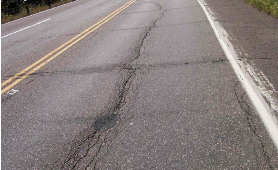
Figure A.7 High Severity Longitudinal Crack (MnDOT, 2011)
