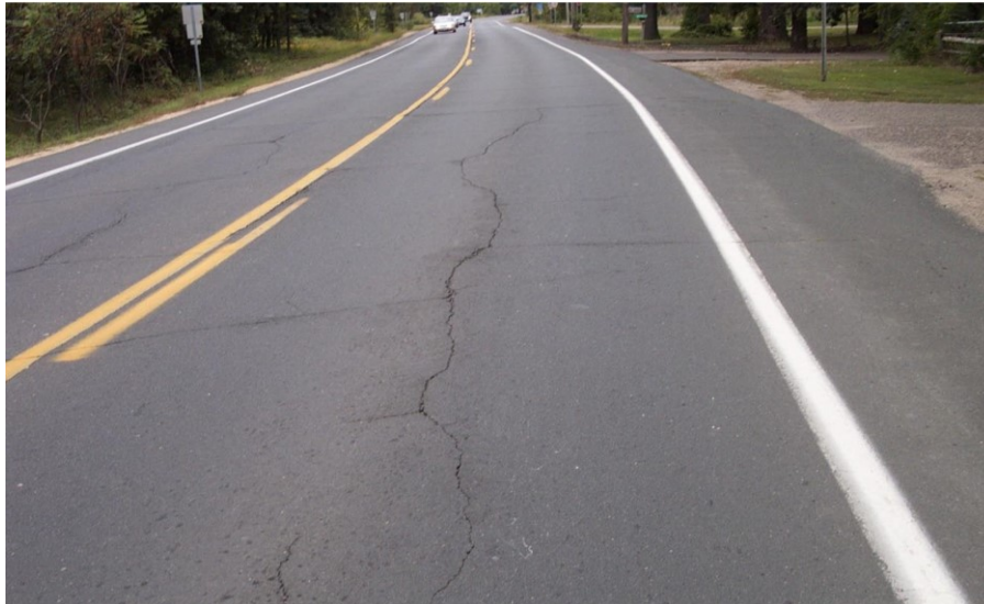
Figure A.4 Low Severity Longitudinal Crack (MnDOT, 2011)
