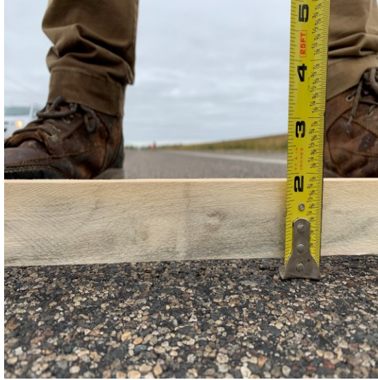
Figure 4-17 Rutting on CSAH 18 West
