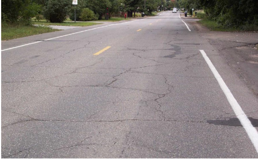
Figure A.11 Medium Severity Multiple Cracking (MnDOT, 2011)
