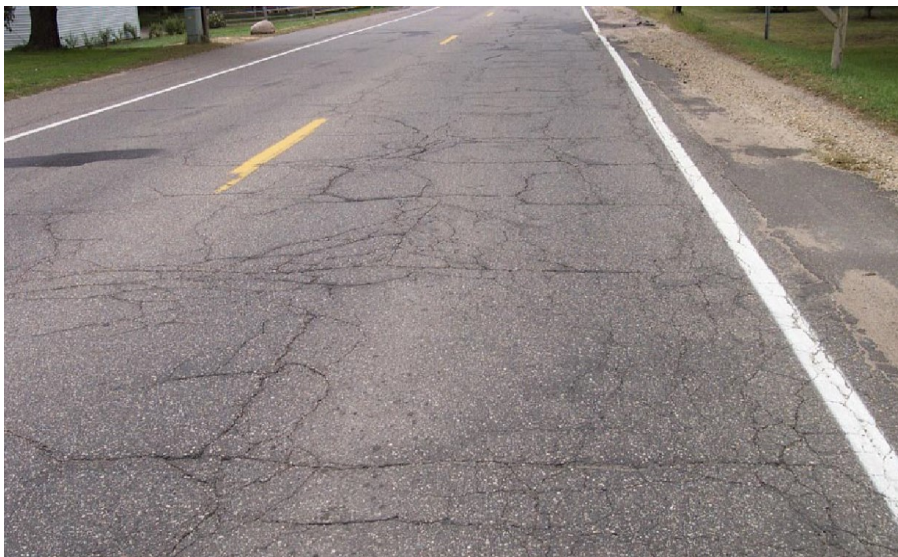
Figure A.12 High Severity Multiple Cracking (MnDOT, 2011)
