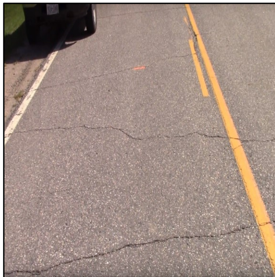
Figure 4-16 Closely spaced transverse cracks on a road in Koochiching County
