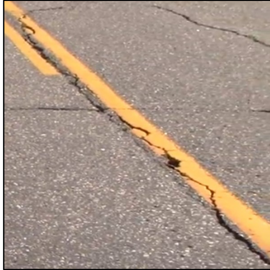
Figure 4-15 Low severity longitudinal joint cracking
