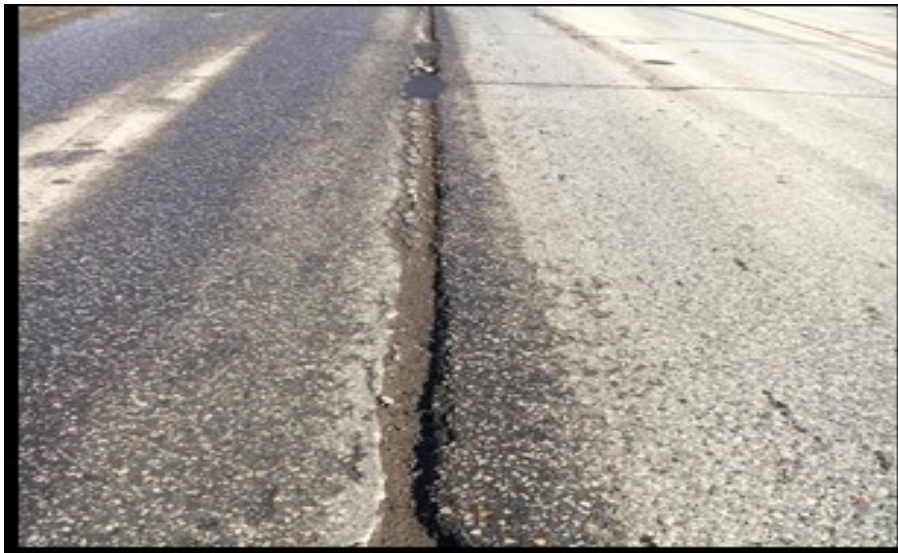
Figure A.8 High Severity Longitudinal Crack at Lane Joint (Photo Courtesy: Manik Barman)
