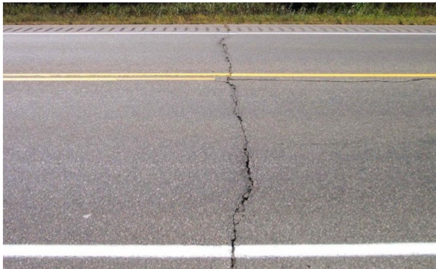
Figure A.2 Medium Severity Transverse Crack (MnDOT, 2011)
