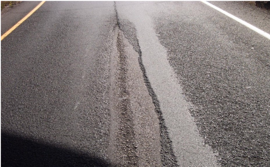
Figure A.16 Raveling in Asphalt Pavement (MnDOT, 2011)
