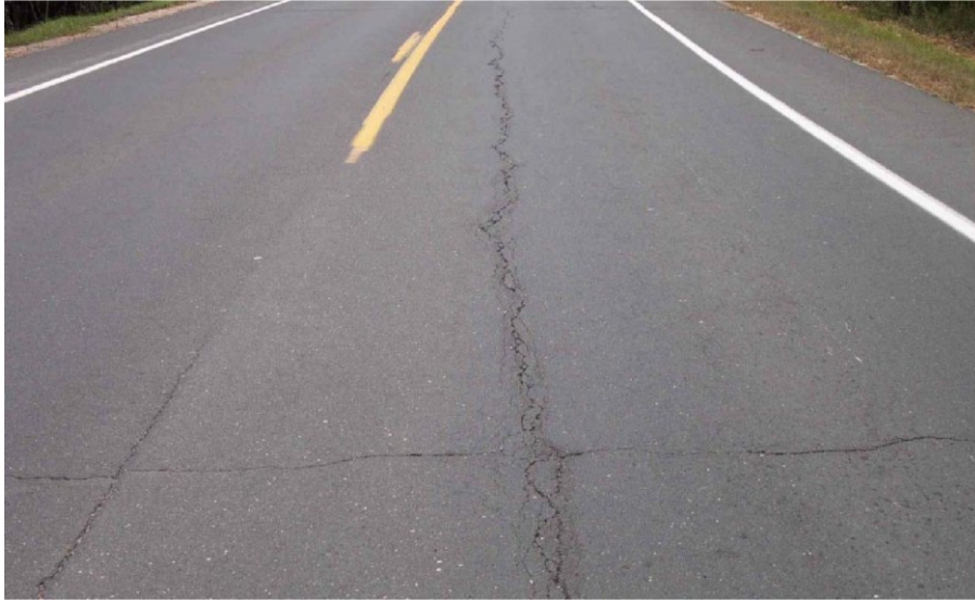
Figure A.5 Medium Severity Longitudinal Crack (MnDOT, 2011)
