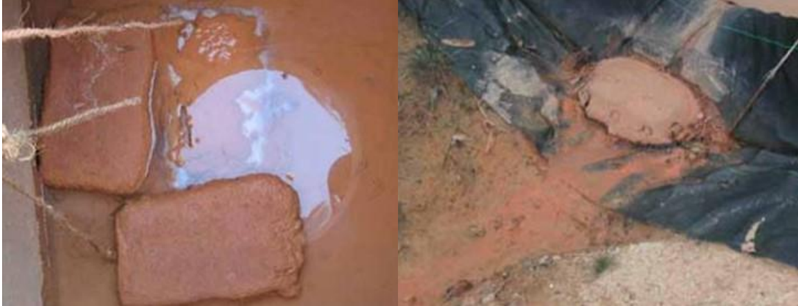
(a) improper maintenance in storm drain inlet [A]
