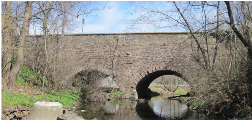
Fig. 3.10 – Photos of the BMS ID 46-4031-0314-1676 in the Montgomery County. (Figures adapted from a 2015 bridge inspection report).
