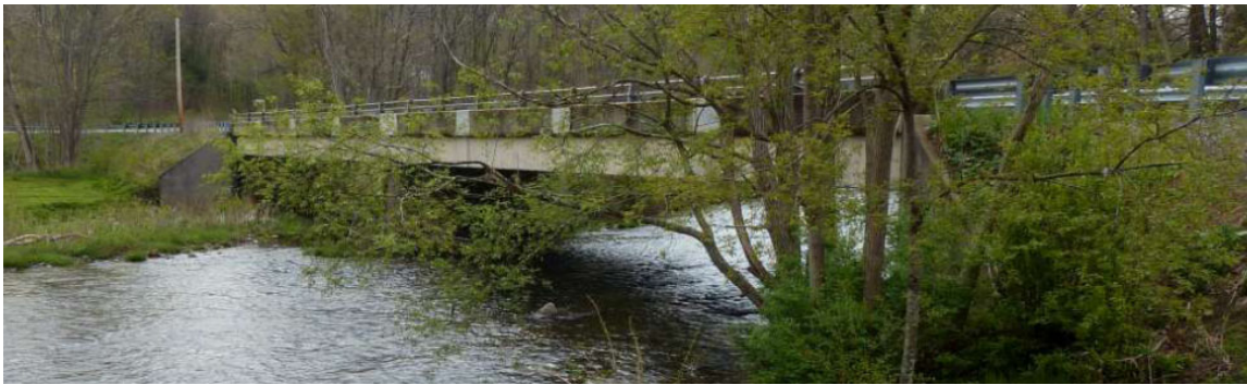
Fig. 3.7 – Photos of the 55-3014-0050-0509 bridge (Somerset Bridge). Figure adapted from PennDOT bridge inspection 2014. Upstream view.
