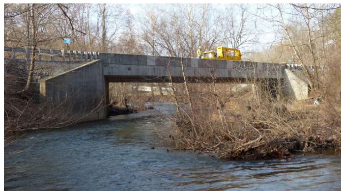
Fig. 3.8 – Photo of the single span ID 29-2004-0040-0000 bridge over little Tonoloway Creek in Fulton County.
