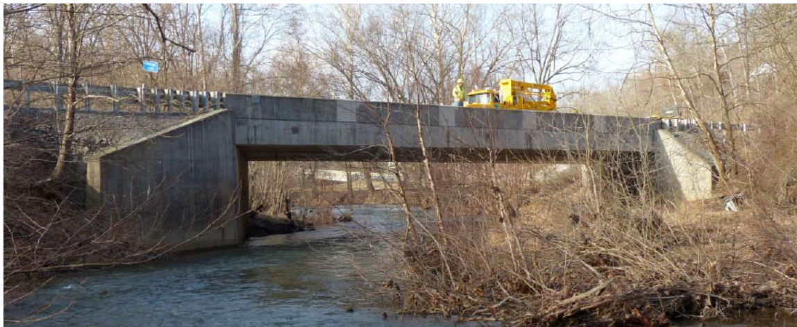
Fig. 6.1. Photos of the three bridges considered in this study. (a) Upstream view of the BMS 55-3014-0050-0509 bridge, for convenience referred here as the Somerset bridge. (b) Cooks Mill Bridge (BMS ID 05-3001-0080-0000). (c) Single span ID 29-2004-0040-0000 bridge over little Tonoloway Creek in Fulton County
