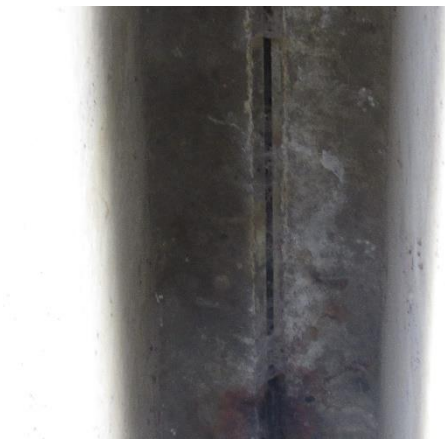
(c) Efflorescence in joint
