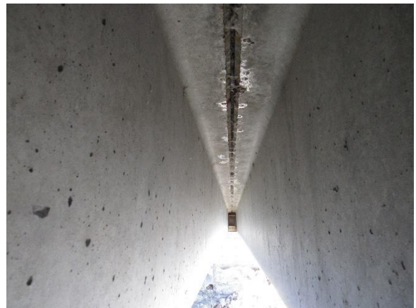
(f) Leakage from joint
