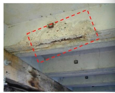
(c) Stem Cover Deterioration (CS-4)
