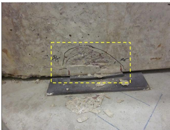
(c) Concrete Spalling at Support
