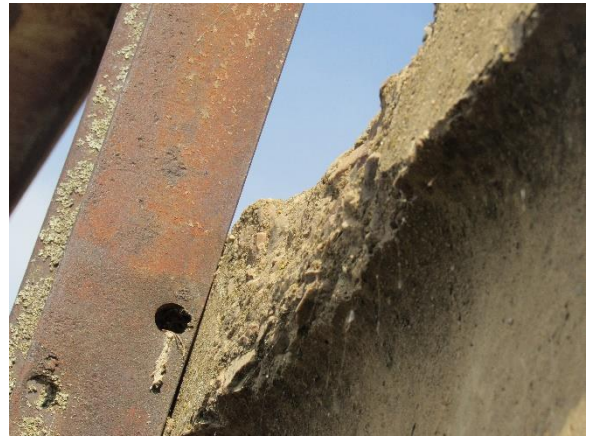
(b) Deterioration at side of bridge
