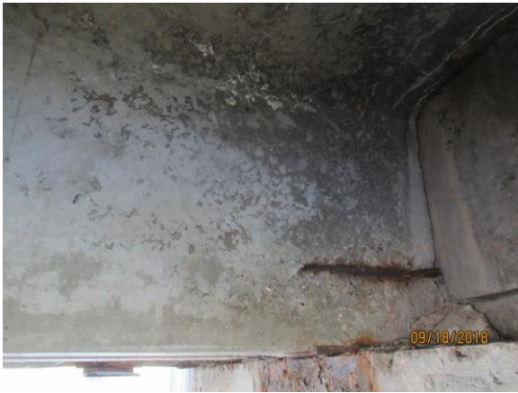
(f) Spall with Prestressing Strand Exposed – South End of East Stem of Deck Unit 6
