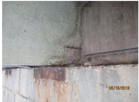
(e) Spall with Prestressing Strand Exposed – South End of East Stem of Deck Unit 3
