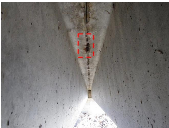
(c) Corrosion in the joint
