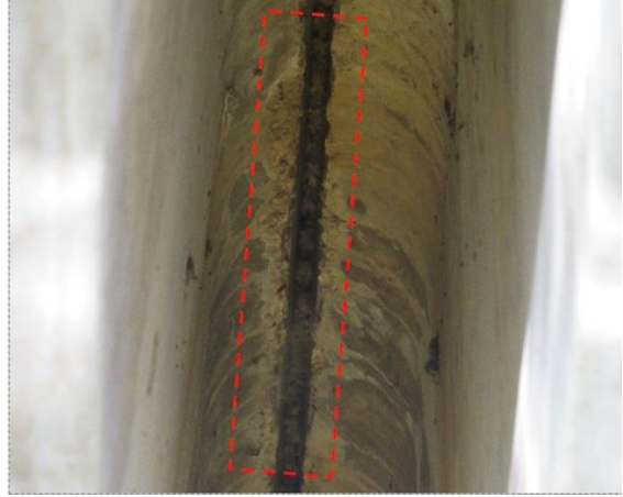
(b) Stains from Minor Corrosion of Steel Plates
