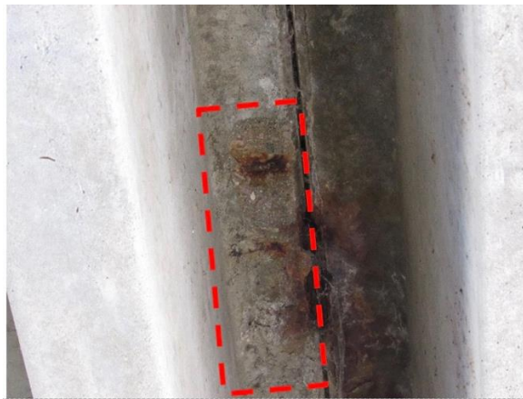
(e) Deterioration in Joint
