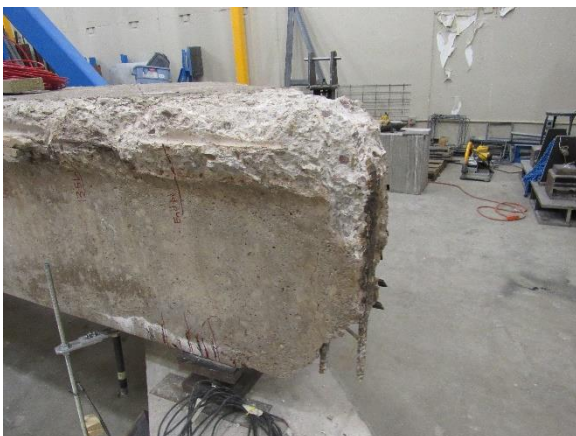
(e) Reinforcement Exposure of 30-ft (9.14-m) Girder
