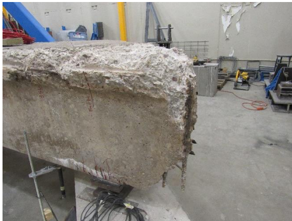
(c) Reinforcement Exposure
