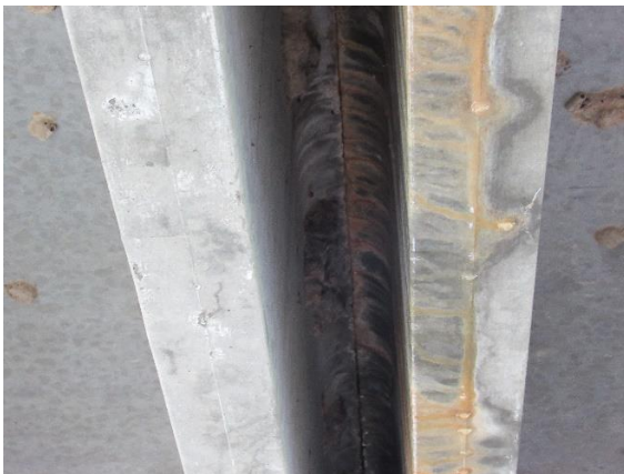
(c) Girder-to-Girder Damage
