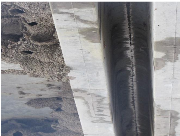
(e) Efflorescence in joint
