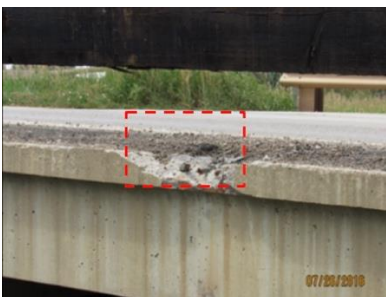
(v) Flange Exposure of Rebar (CS-1) & Flange Cover Deterioration (CS-4)
