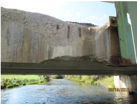
(h) Spall with Exposed Rebar Near Post 4 – Deck Unit 7
