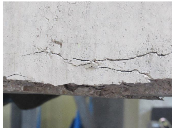
(d) Damage of 50-ft (15.24-m) Girder during Unloading
