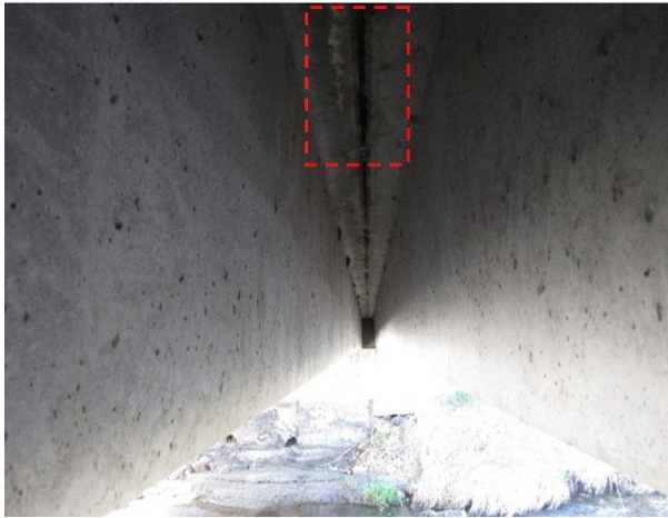
(a) Efflorescence in Joint
