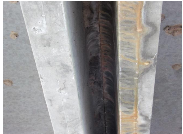
(f) Sign of corrosion
