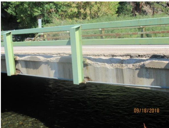
(c) Deterioration of West Side of West Deck Unit
