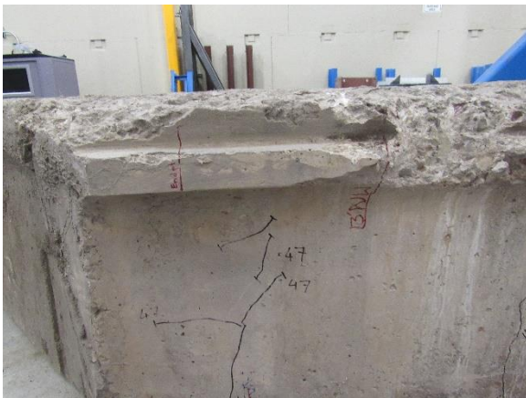
(c) Shear Crack Near North End
