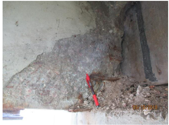
(g) Spall with Prestressing Strand Exposed – South End of East Stem of Deck Unit 7
