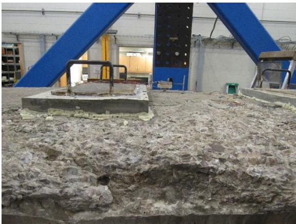
(c) Flange Cover Deterioration of 30-ft (9.14-m) Girder
