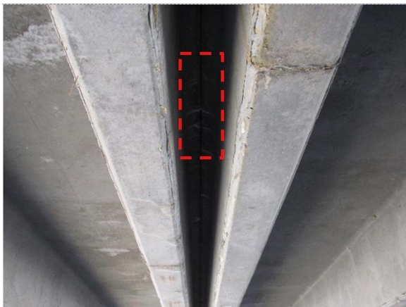
(e) Efflorescence at joint
