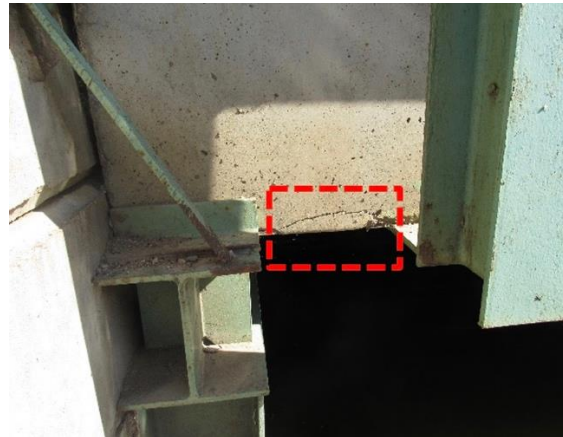
(b) Cracking at bottom of exterior girder
