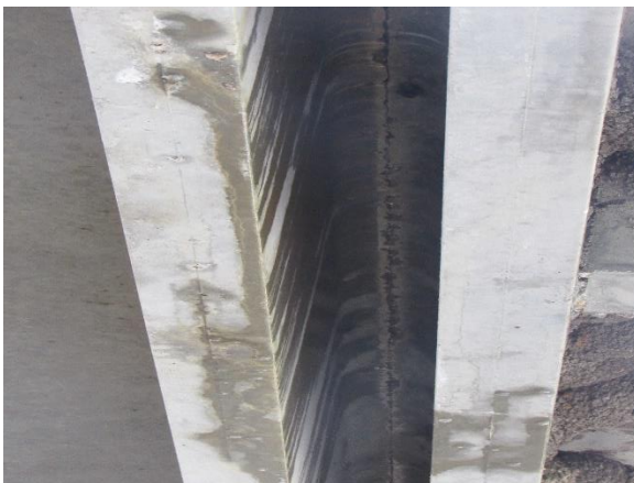
(c) Leakage from joint
