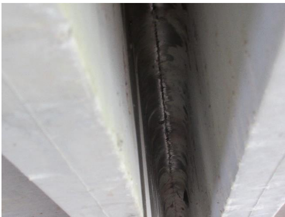
(c) Efflorescence in joint
