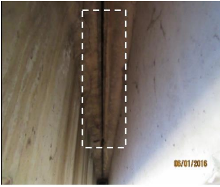
(m) Flange Girder to Girder Longitudinal Deterioration (CS-2)
