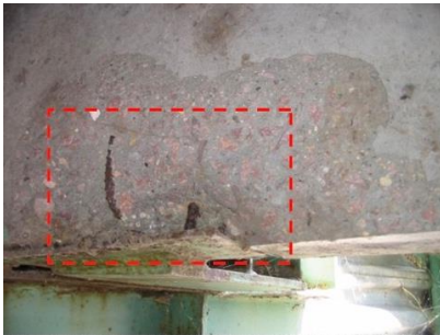
(s) Stem Exposure of Transverse Rebar (CS-1)/Stem Cover Deterioration CS (4)
