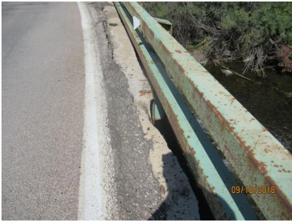
(a) Deterioration of Concrete on Top of East Deck Unit
