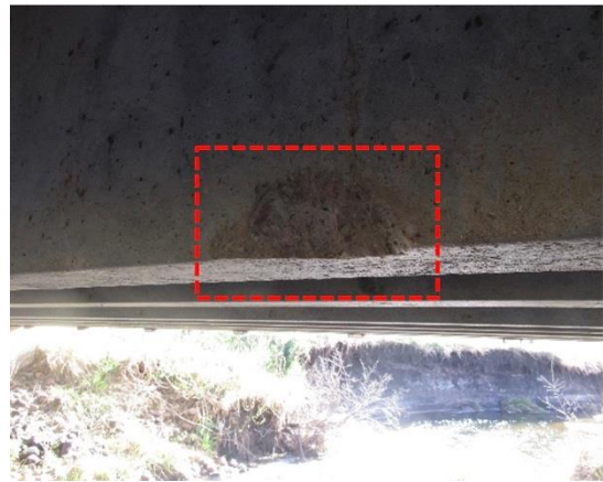
(b) Spalling at stem of bridge
