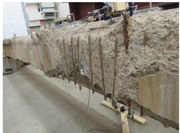
(f) Exposure of Strands and Transverse Bars on Stem of 50-ft (15.24-m) Girder
