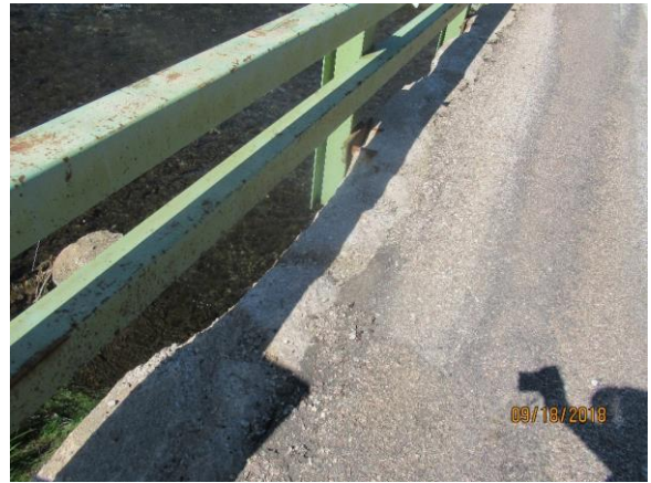
(b) Deterioration of Concrete on Top of West Deck Unit
