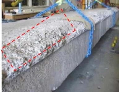
(e) Flange Cover Deterioration (CS-3)
