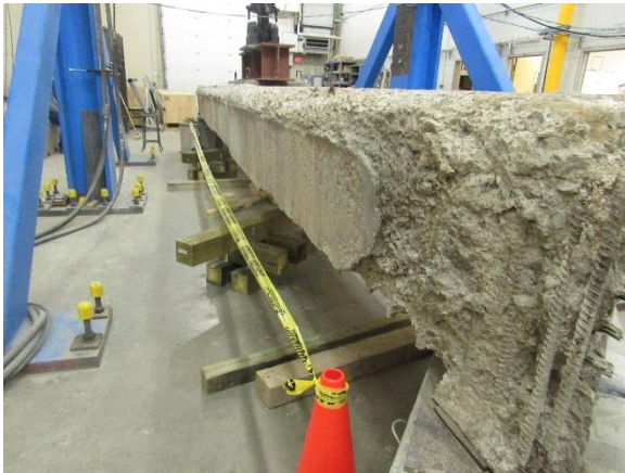
(a) Stem Cover Deterioration for 30-ft (9.14-m) Girder
