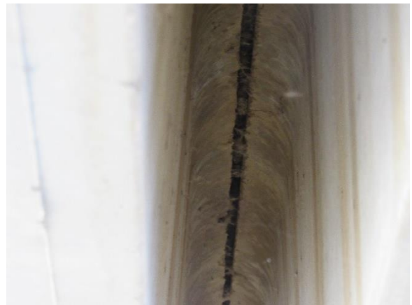
(f) Wide gap in joint
