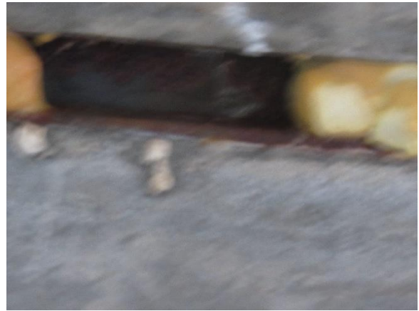
(b) Corrosion of plate of joint
