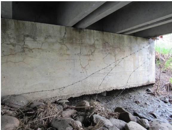
(e) Scouring from bottom of abutment
