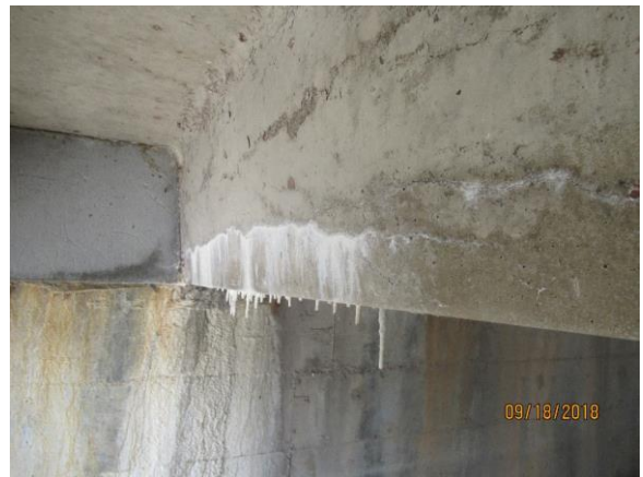
(d) Longitudinal Cracking and Severe Efflorescence- North End of Deck Unit 1
