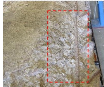
(f) Flange Cover Deterioration (CS-4)
