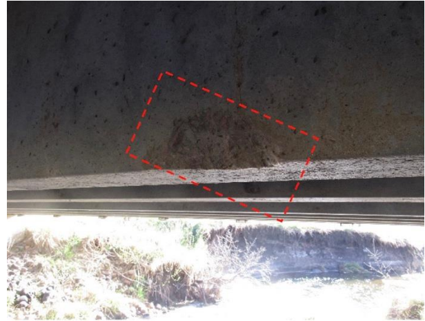
(b) Spalling at bottom of Stem, G4
