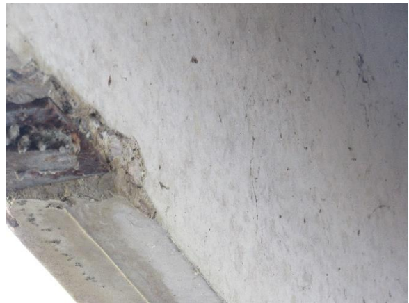
(f) Deterioration at bottom of stem
