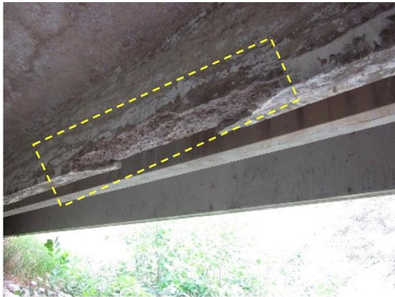
(a) Stem Cover Deterioration
