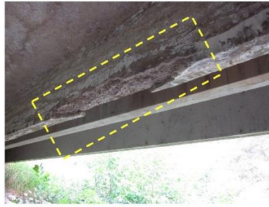
(b) Stem Cover Deterioration (CS-3)
