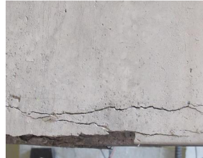
(i) Stem Cracking (CS-4)
