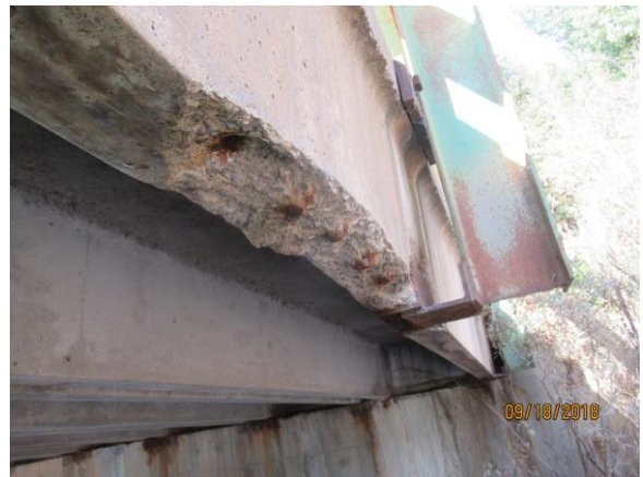
(i) Spall Near Rail Post 5 – Deck Unit 7
