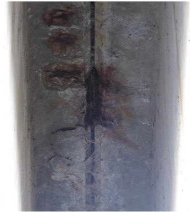
(b) Corrosion in joint
