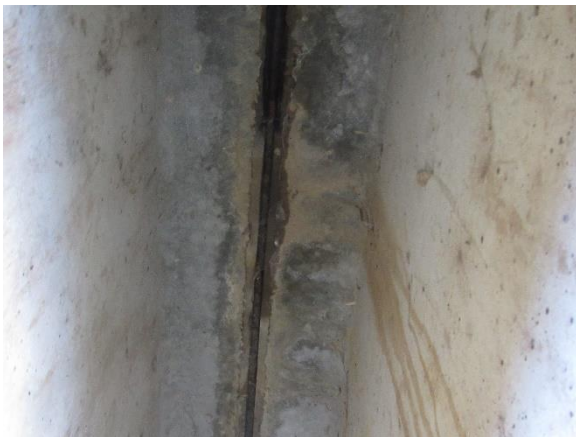
(e) Leakage from joint
