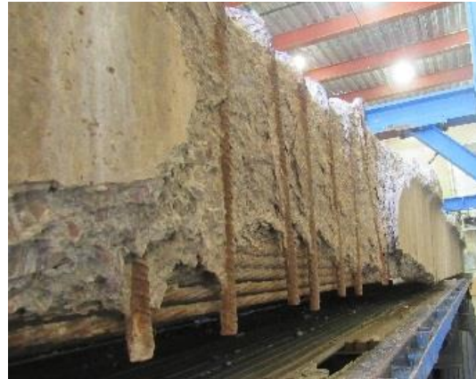
(b) Stem Reinforcement Exposure
