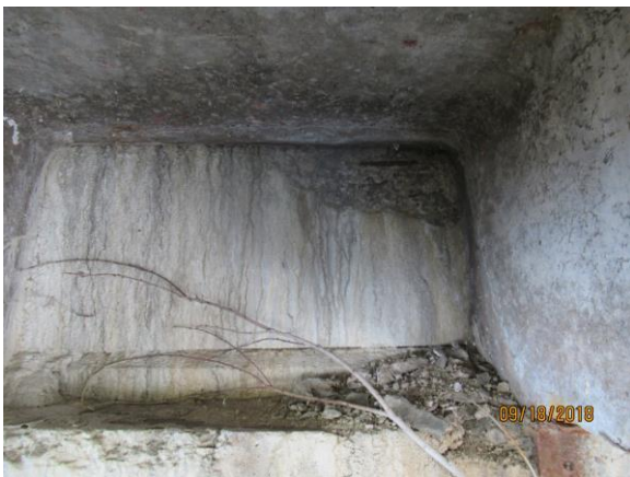
(k) Spall in North Backwall with Exposed Rebar Beneath Deck Unit 7
