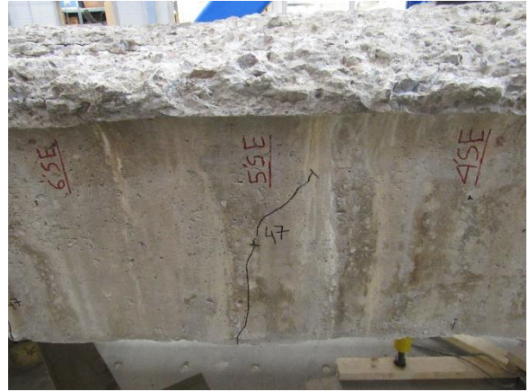
(b) Flexural Crack Near to Midspan
