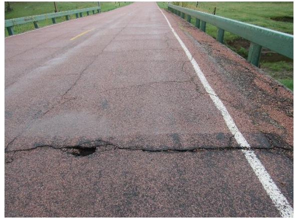
(b) Cracking on pavement over the bridge
