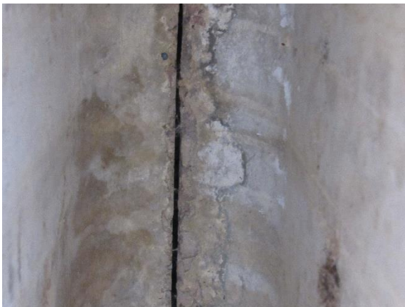
(e) Efflorescence at joint
