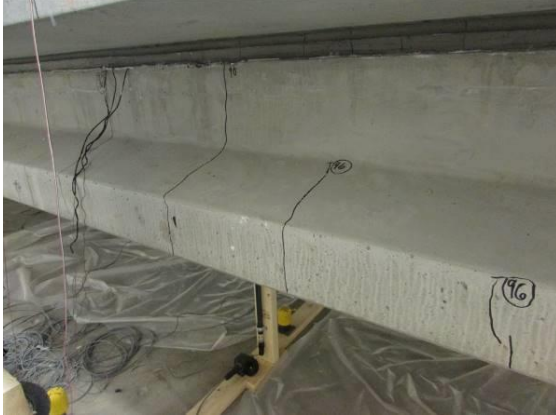
(c) Crack Pattern for Girder A at P = 263 kips
