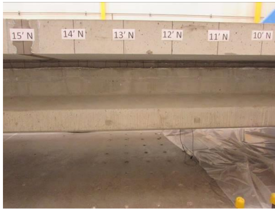
(a) Shrinkage Cracks in Haunch Region of Girder A Filled with Latex Modified Concrete
