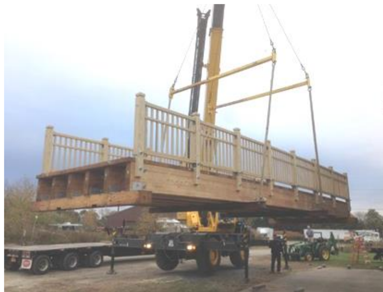
Figure 5.32: Erie Canal Bridge Being Placed in Port Byron, NY in 2014 (after laminatedconcepts.com)
