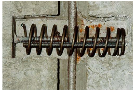
(b) Photograph of Block-out with Tied-in Lap Splice and Spiral Confinement (after Badie et al., 1998)
