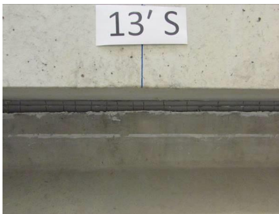
(c) Shrinkage Cracks in Haunch Region of Girder B Filled with Non-Shrink Grout
