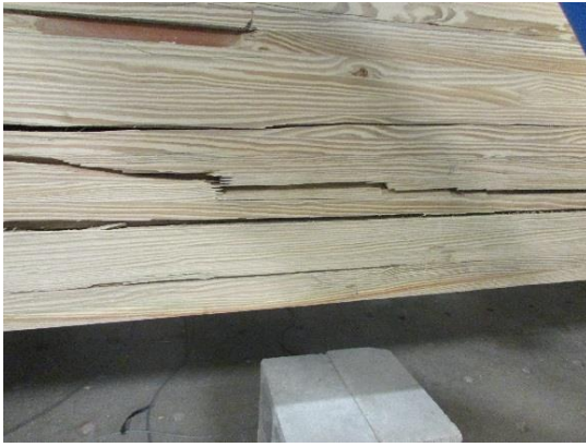
(a) Failure of West Girder
