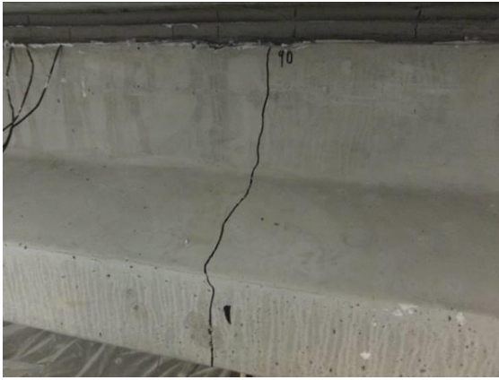
(a) First Crack, Mid-span of Girder A at P = 251 kips
