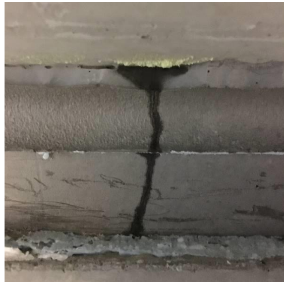
(b) Close Up of Crack
