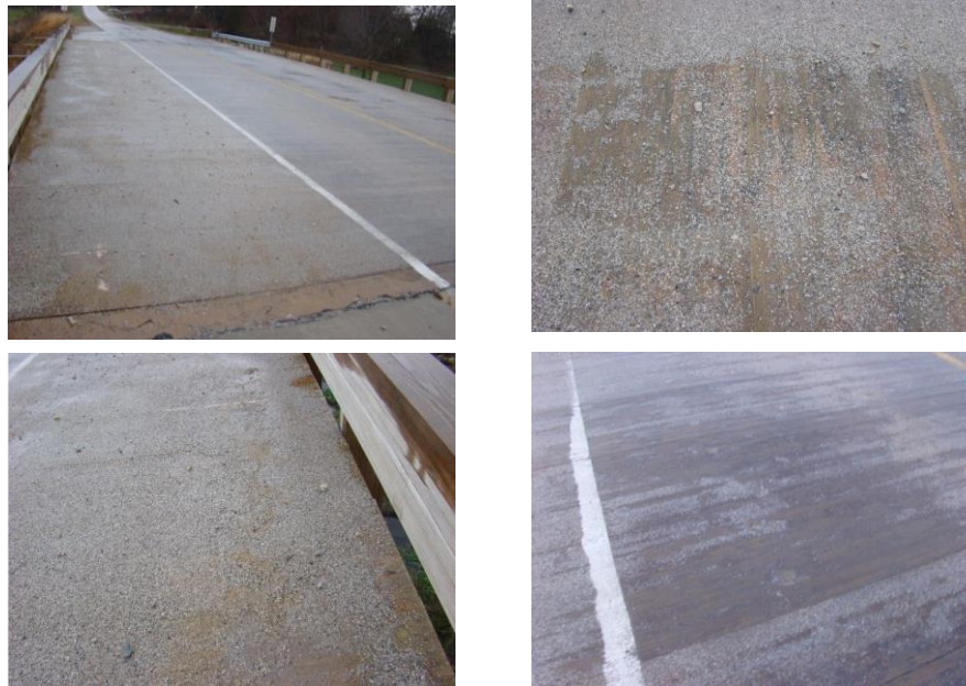
Figure 5.29: Epoxy with Embedded Grit Wearing Surface for Glulam Timber Bridge in Buchanan County, Iowa
