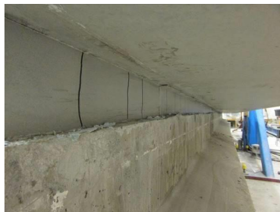
(d) Close Up of Girder B Haunch Region Filled with Non-Shrink Grout
