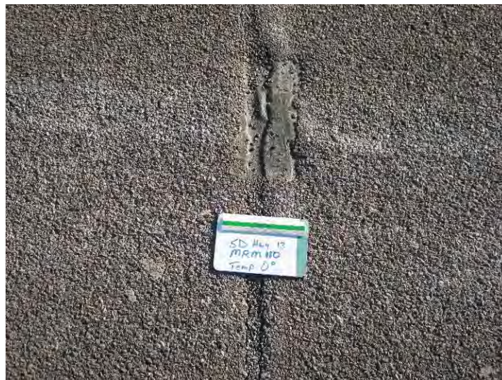
Figure 6 Exposed crack sealant on Highway 13, MRM 110 – winter 2014.
