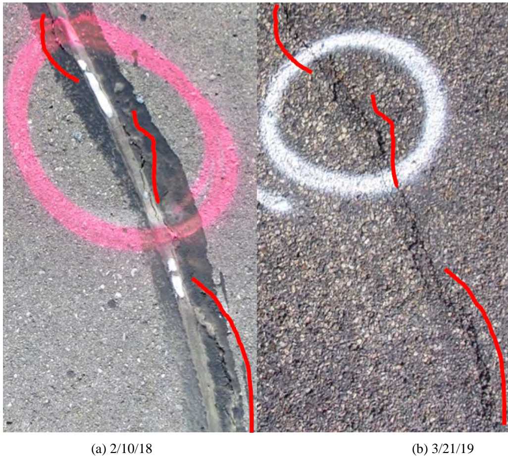
Figure 26 Sealant distress observed before (a) and after (b) chip sealing. Red lines drawn on both photographs represent the same sealant distress.
