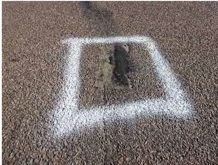
Figure 7 Exposed crack sealant on HWY 13, MRM 110 – winter 2016
