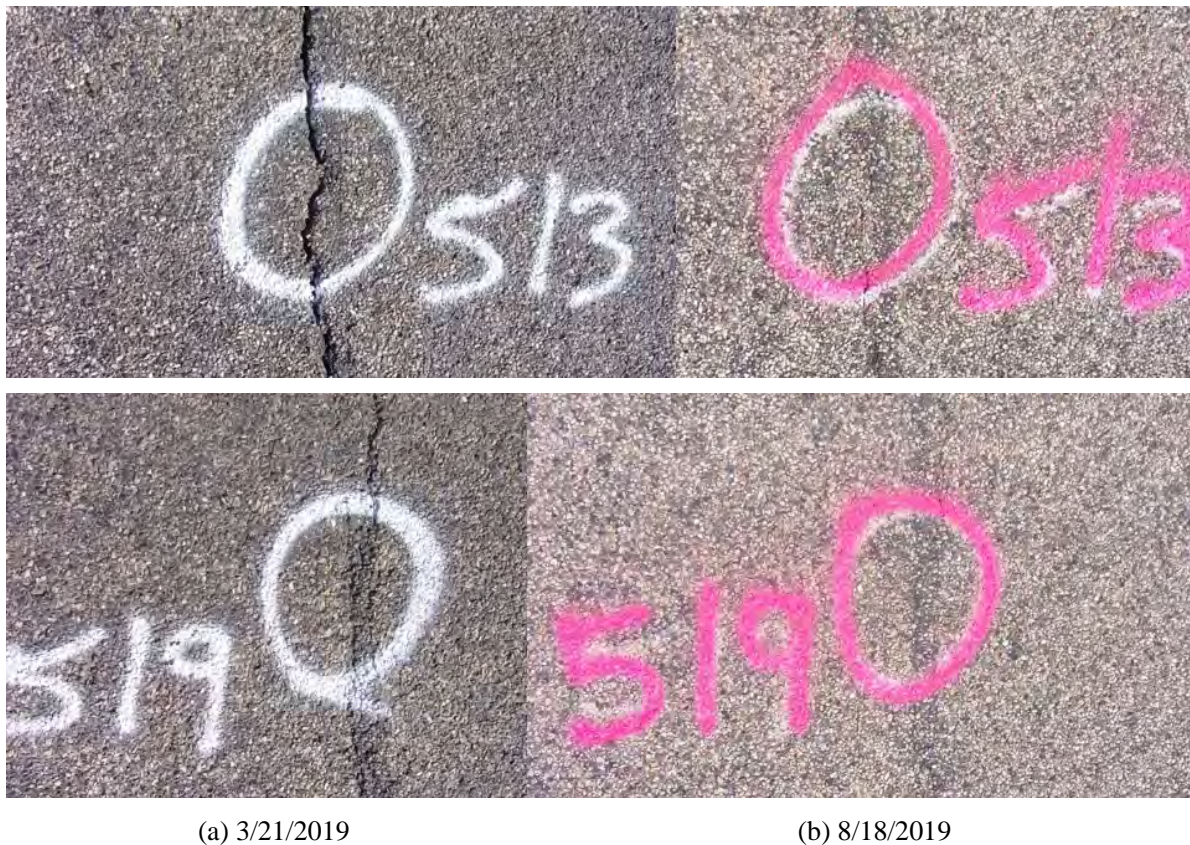
Figure 25 Observed crack sealant condition during winter (a) and summer (b) inspections.
