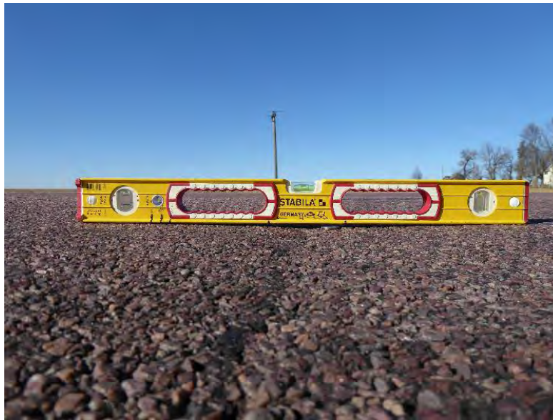
Figure 4 Evidence of subsidence near the crack, Highway 11 – winter 2016.
