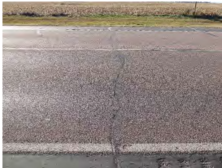
Figure 10: Crack sealant on Highway 38, post chip seal – winter 2016.
