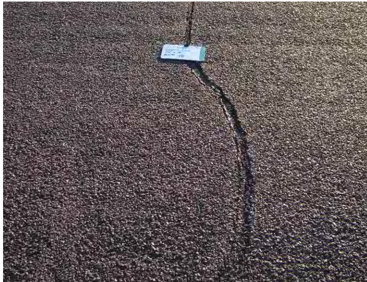
Figure 12 Recession of the crack reservoir on Highway 81, MRM 98 – winter 2013.
