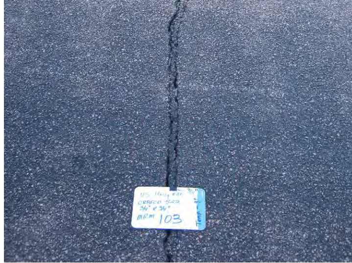
Figure 13 Typical distresses of the crack sealant on Highway 81, MRM 103 – winter 2013.
