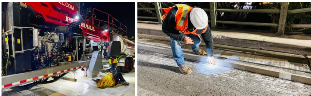
Figure 5: Diamond Grinding of the New PCC Validation of Smoothness Using a 16-ft Straight Edge
