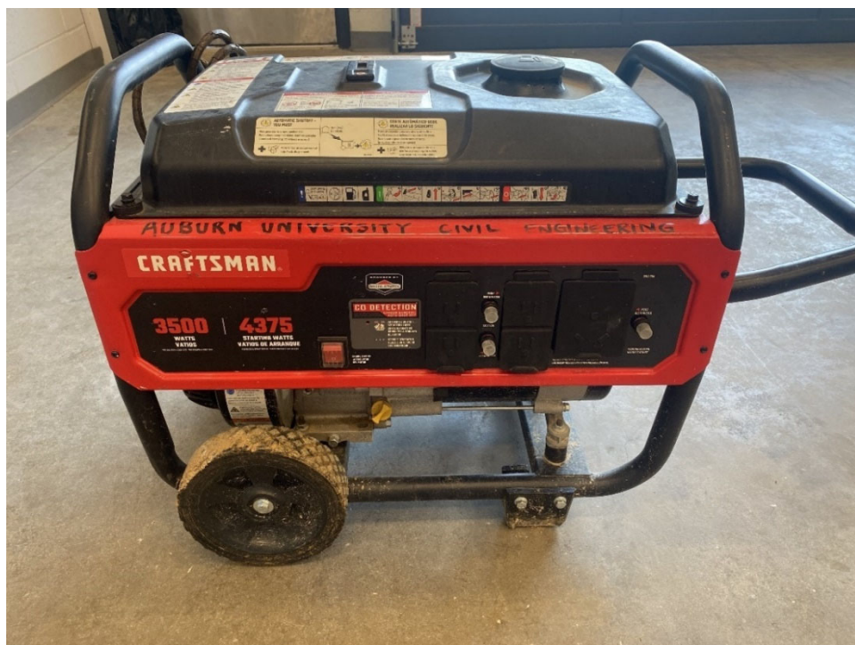
Figure 5-6: Generator used to provide power to SIC Curing Box
