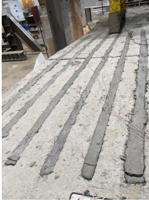
Figure 4.10 Debonding and cracking of grout
