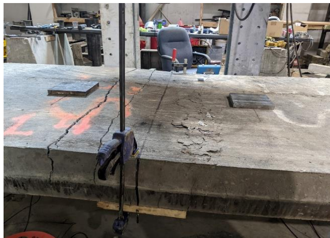
Figure 3.24 Damage slab specimen
