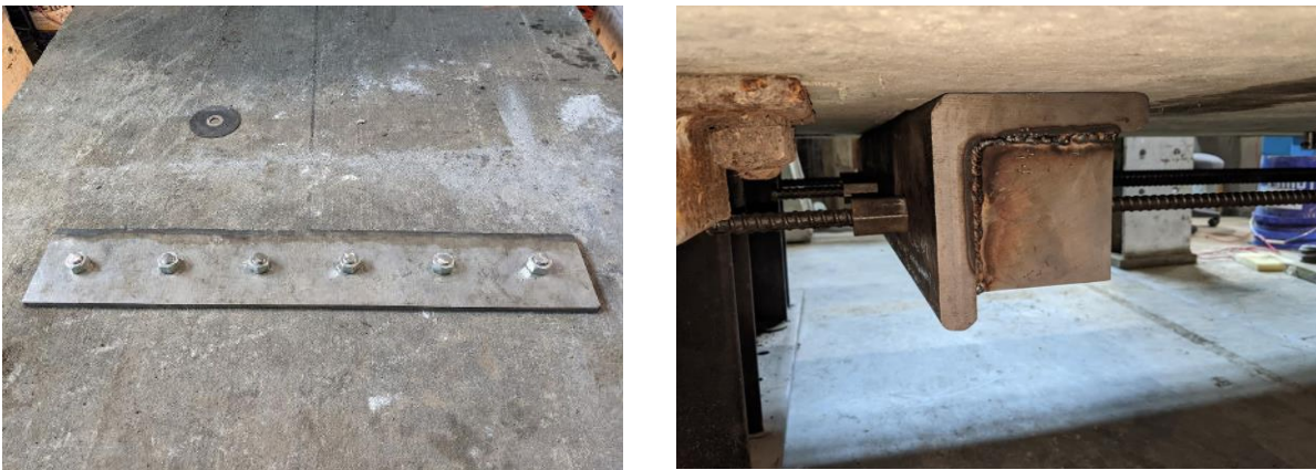
Figure 3.15 Installation of steel plates (left) and installation of steel angles and DYWIDAG threadbars (right).
