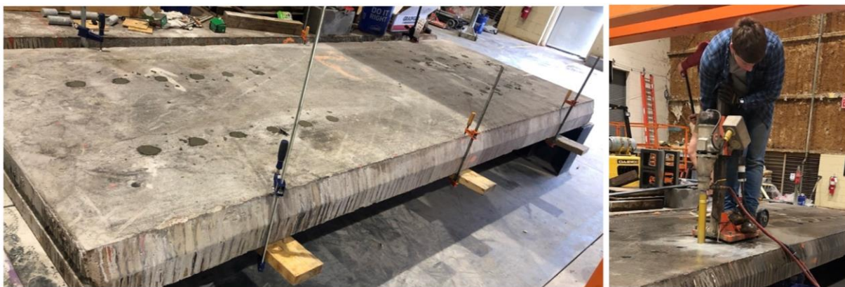
Figure 3.12 Installation of bolts and grout of the strengthened slab with steel plates from bottom. Wood planks, clamps, and grout are shown in the left photo; hole cutting is shown in the right photo.
