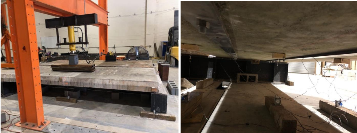
Figure 3.13 Strengthened slab test setup and ready for loading (left). Two plates installed on bottom of slab (right).
