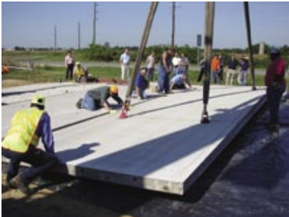
CPTP has sponsored precast concrete pavement demonstrations in Missouri and other States (see page 3).
