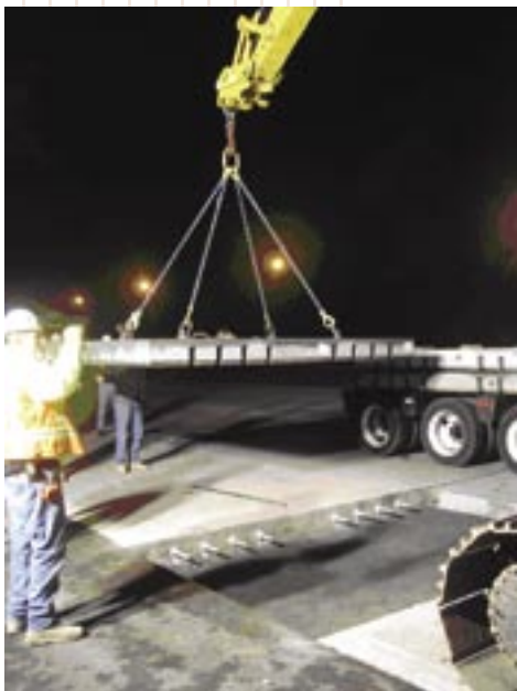
Intermittent repairs along a section of I-295 in New Jersey using the Fort Miller Super-Slab system (May 2008)..
