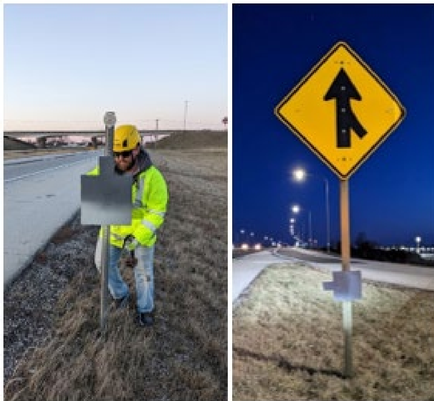
Figure 8. Photos. A target being mounted (left) and a target mounted to a signpost (right).
