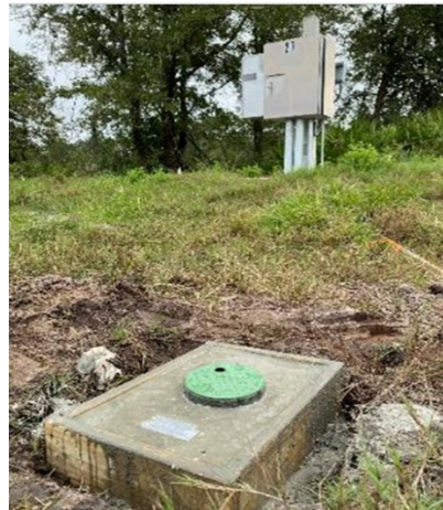
Figure 15. Monitoring well (Greene, 2020).
