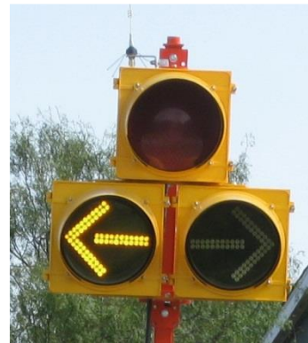
b. Flashing Proceed Indication.
