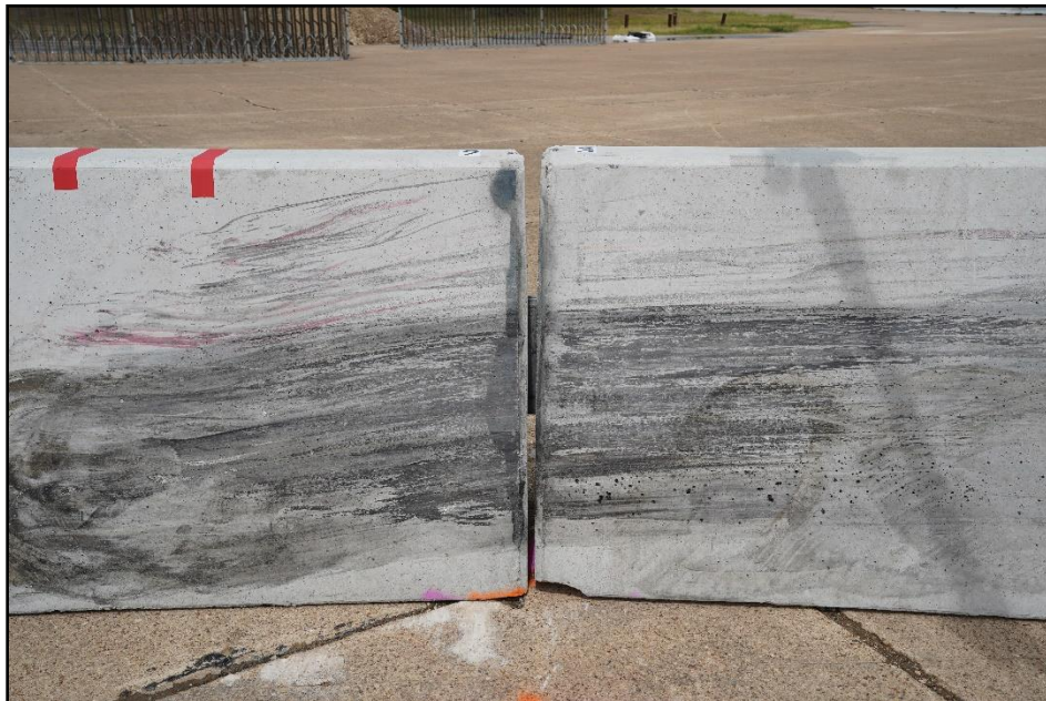
Figure 7.6. Flared Single-Slope Portable Concrete Barriers after Test at the Joint of Barriers 2 and 3, Test 440862-03-4.
