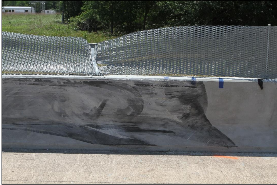
Figure 8.7. Screen-Safe® Glare Screen on F-Shape Barrier after Test at the Joint of Posts 6 and 7, Test 440822-01-4.
