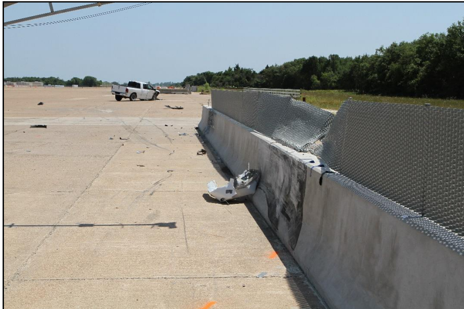
Figure 8.6. Screen-Safe ® Glare Screen on F-Shape Barrier after Test at Impact Location, Test 440822-01-4.
