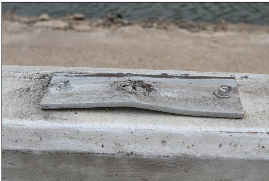
Figure 5.8. Armorcast® Gawk Screen on Single-Slope Barrier after Test at Base Plate with Missing Post, Test 440822-01-1.
