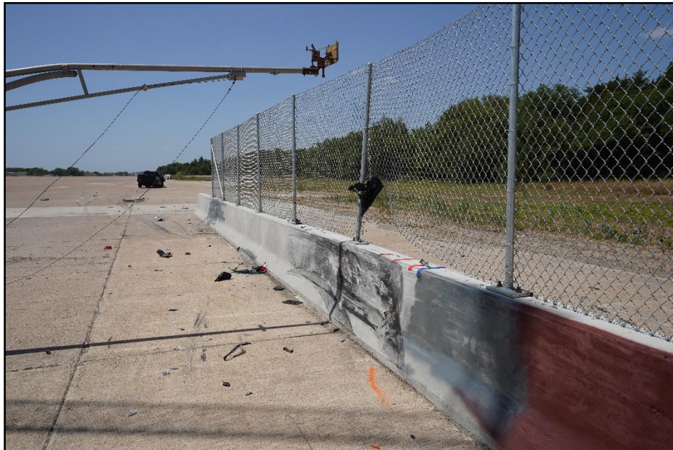
Figure 9.6. Chain-Link Fence on F-Shape Barrier after Test at Impact Location, Test 440822-01-5.
