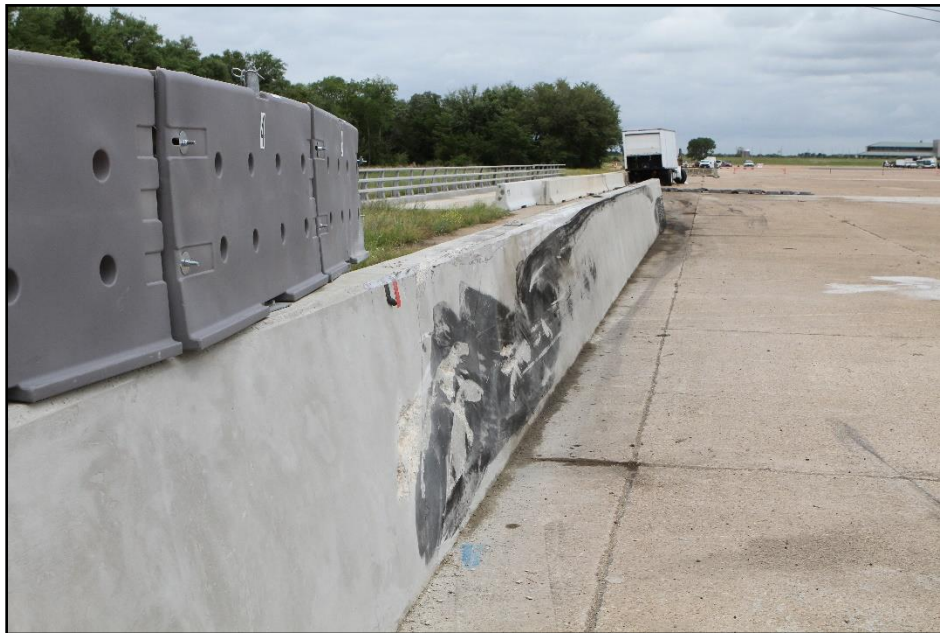
Figure 5.6. Armorcast® Gawk Screen on Single-Slope Barrier after Test at Impact Location, Test 440822-01-1.
