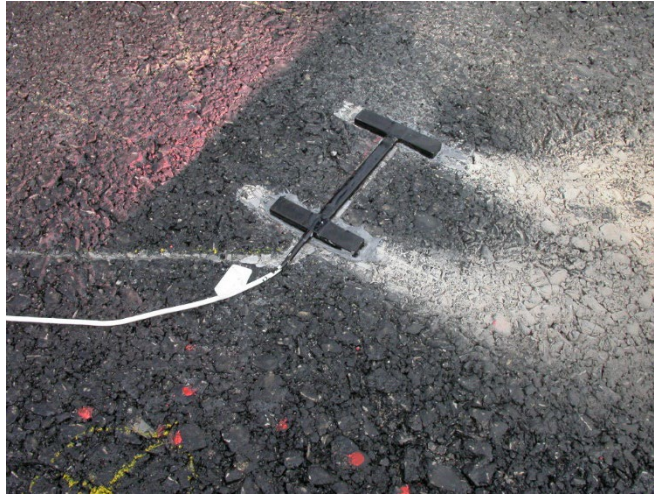
Figure 19. H-type Strain Gauge installed on the top of base course (Solaimanian et al., 2006).
