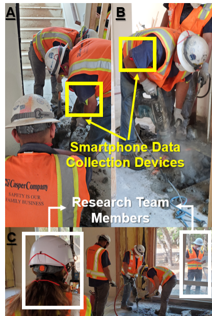
Figure 6. A) The worker using the TE 100 AVR, B) The worker using the HM1203C, C) The data collection scene with research team members.
