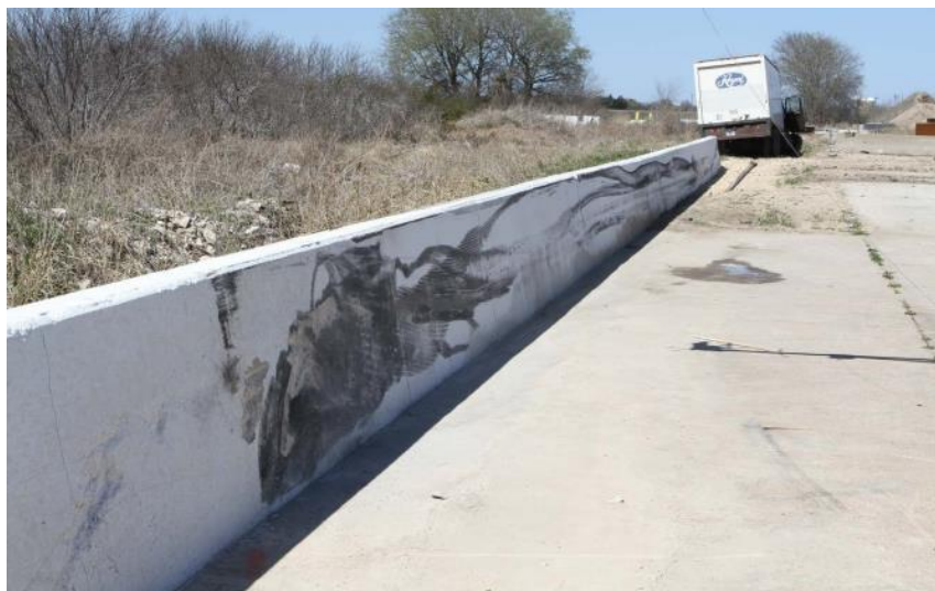
Figure 3-2. TxDOT 36-in. SSTR after MASH test 4-12 (Sheikh et al. 2011)
