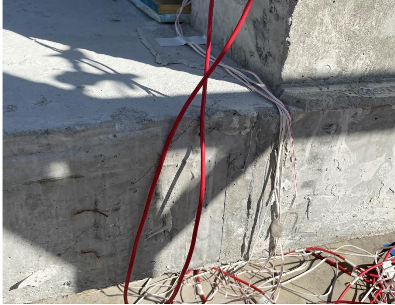
Figure 9-45 Crack in deck with no rail on top (looking towards the back face)
