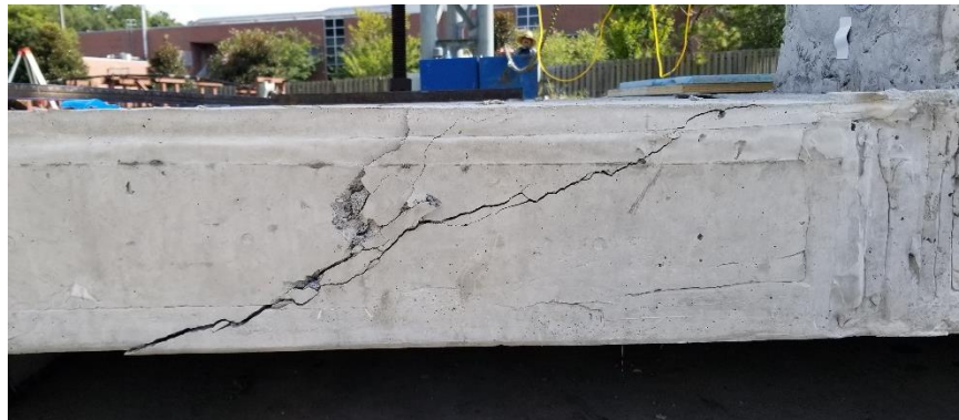
Figure 9-26 Crack in deck with no rail on top (looking towards the back face)
