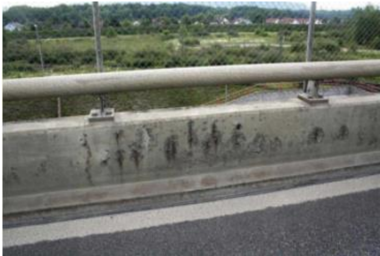
Figure 1-1. Corrosion on bridge rail
