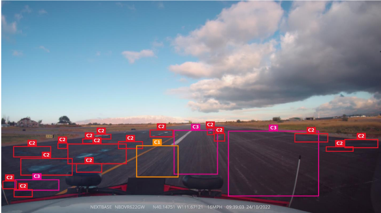
Figure 3.13: Annotated distress types on a segment of the runway. Note: To reduce cluttering, C1 refers to longitudinal and transverse cracking, C2 refers to rutting/depression, and C3 refers to weathering.
