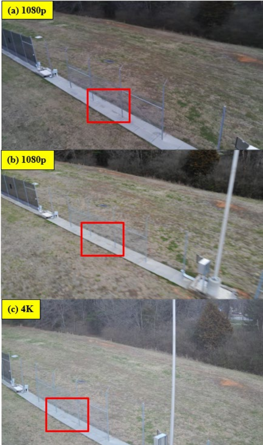
Figure 51. Twilight Recorded Visual Camera Footage of Damaged Fence from 20 ft AGL: (a) ANAFI Triple, (b) M2ED, and (c) XT2 9mm
