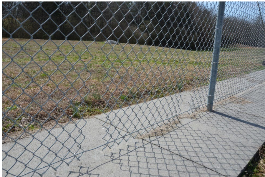
Figure 47. Damaged Test Fence at TYS
