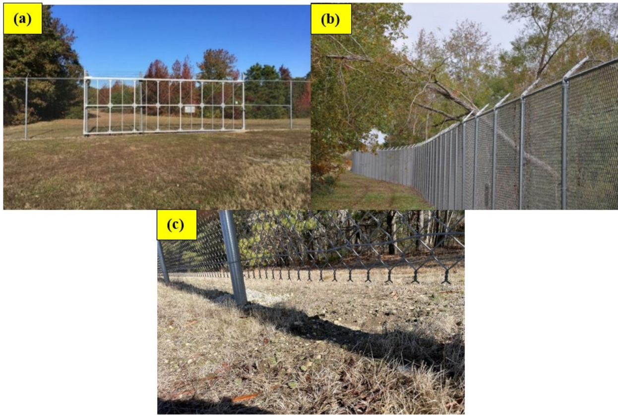
Figure 10. Existing Features: (a) AOA Access Gate, (b) Fallen Tree, and (c) Erosion Underneath Fence
