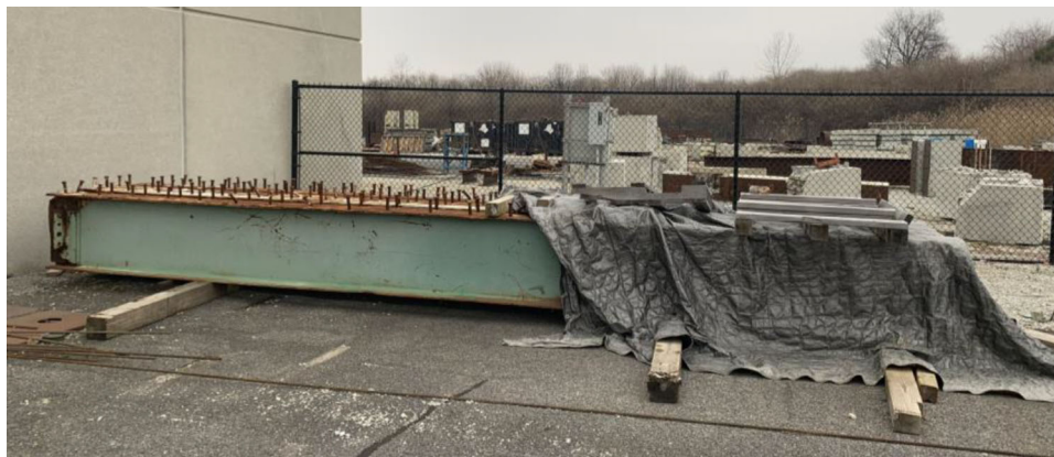
Figure 2.7 Corroded girders being stored on the north side of the Bowen Laboratory at Purdue University.
