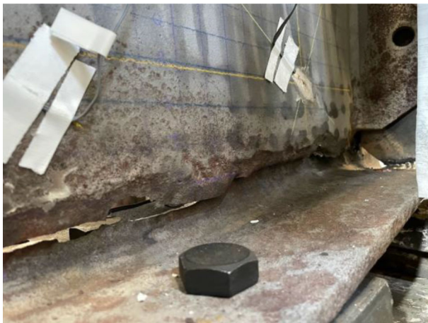
Figure 5.5 Specimen 2 shear rupture at the web bottom (East side).
