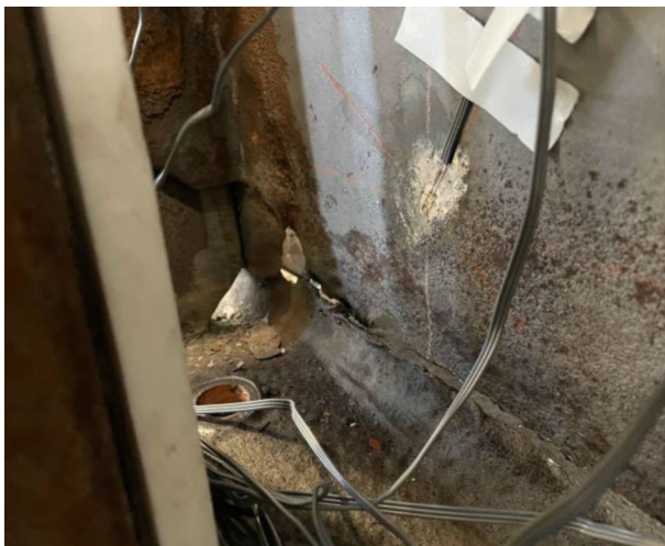
Figure 5.6 Specimen 2 shear rupture at the web bottom (West side).
