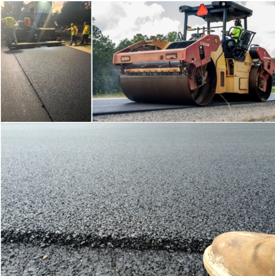
Figure 3. HPTO paving (Top left). HPTO compaction (Top right). Finished HPTO surface (Bottom). Sources: Dr. Tom Bennert, NJDOT, and West Virginia Division of Highways
