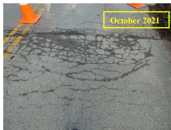
(b) Northbound lane over joint at Abutment 2
