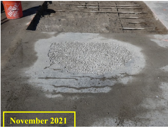
(a) Pothole filled with #8 aggregate
