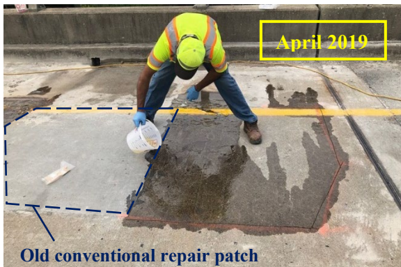
(c) Application of epoxy over cracked Area 1, west of old repair patch
