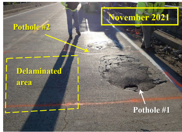
(b) Damage area (looking east)
