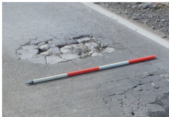
(b) Concrete spalled off from deck
