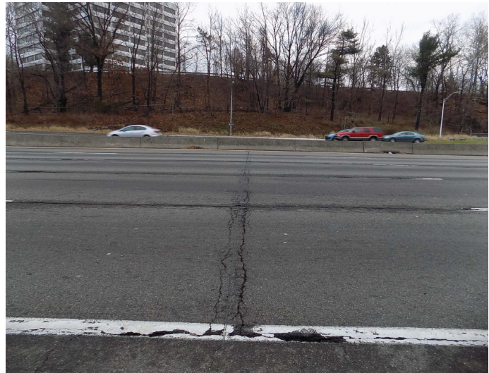
Figure 8-3. Example of pavement deterioration (NJDOT, 2019).
