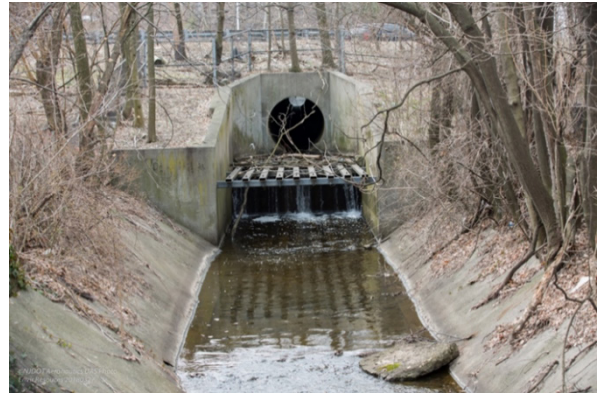
Figure 10-10: Accumulated debris on culvert rack (I-80 Milepost 57.3 Structure #1610177). (NJDOT)
