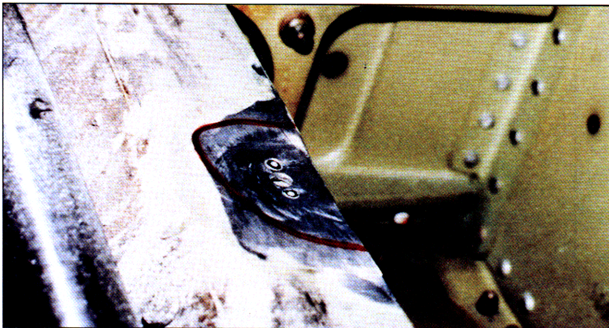
FIGURE 6-5. STEEL PARTICLES FROM FASTENERS OR NUTPLATES MAY CAUSE FUTURE CORROSION PROBLEMS IN ALUMINUM STRUCTURE
