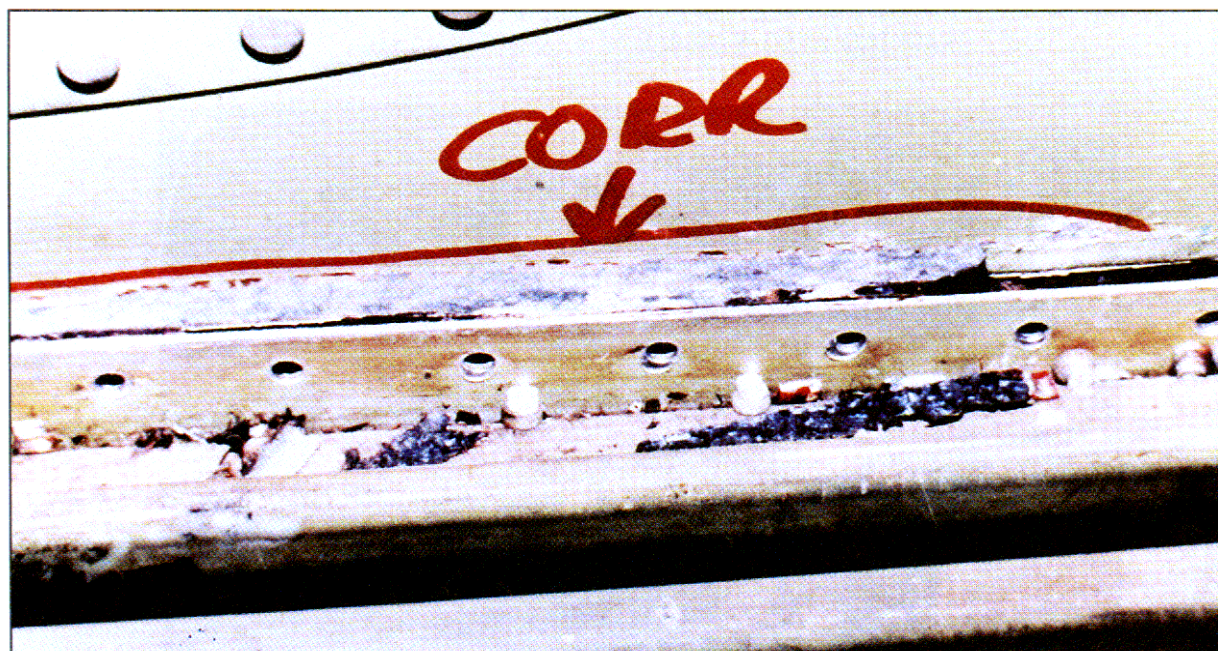
FIGURE 5-10. REMOVAL OF FILLET SEAL FROM INTERNAL EDGE OF LAP JOINT EXPOSED FULL EXTENT OF CORROSION
