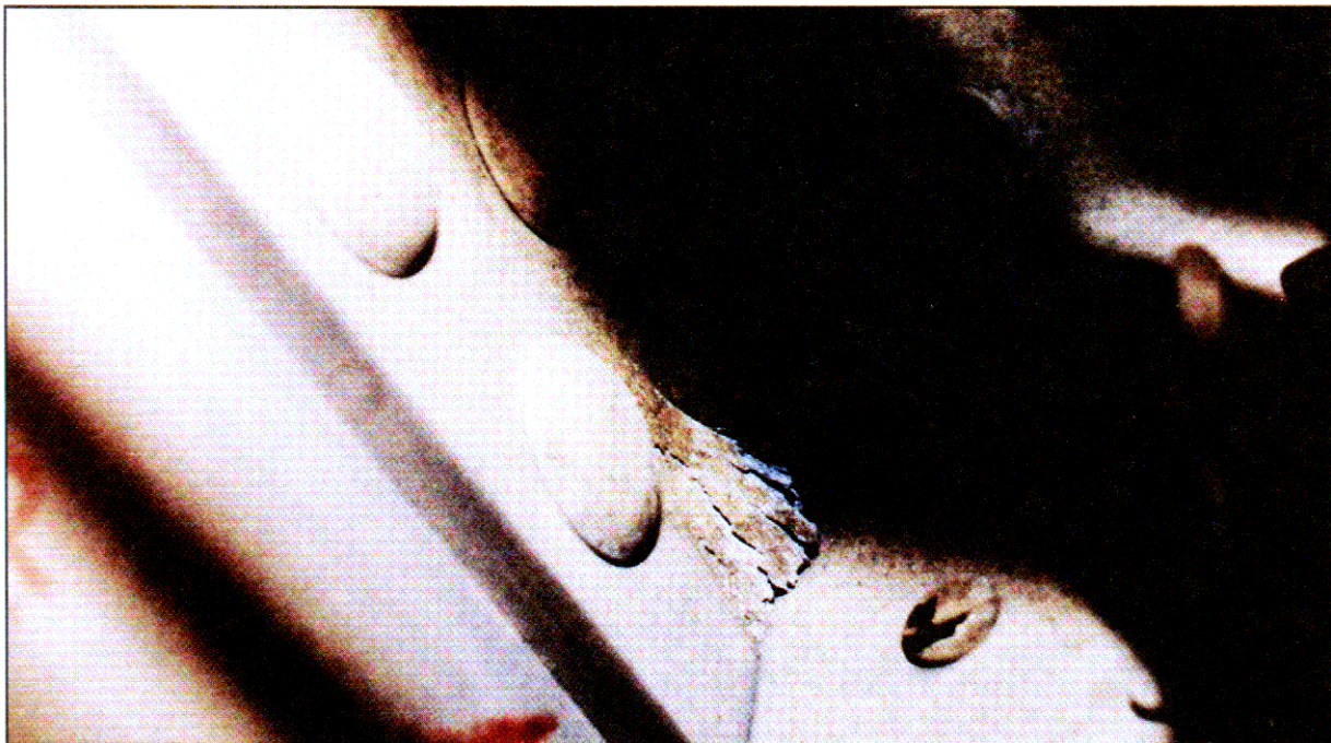
FIGURE 5-9. SPAR CHORD CORROSION
