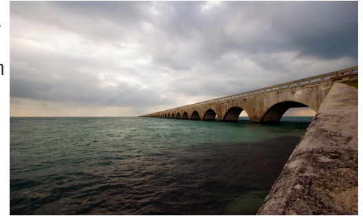
An FDOT research team is investigating the use of hot dipped galvanized steel rebar (HDGR) in the marine splash zone of Florida structures such as bridges.
