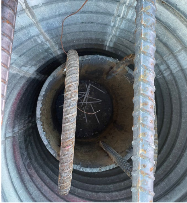
Figure 45: Pile cap void to be filled with UHPC with thermo-coupling wires installed
