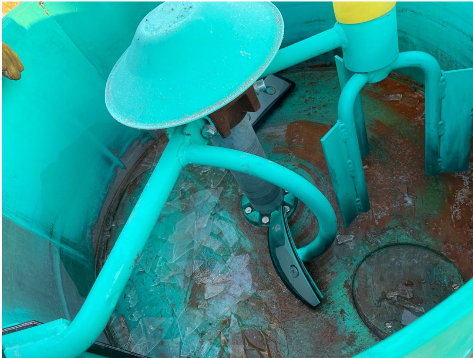
Figure 49: Ice formed in the bottom of the mixer prior to the start of construction
