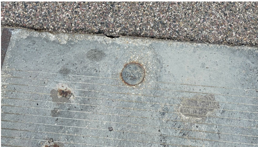
Figure 75: Rusting of embedded pipe on deck-to-cap connection
