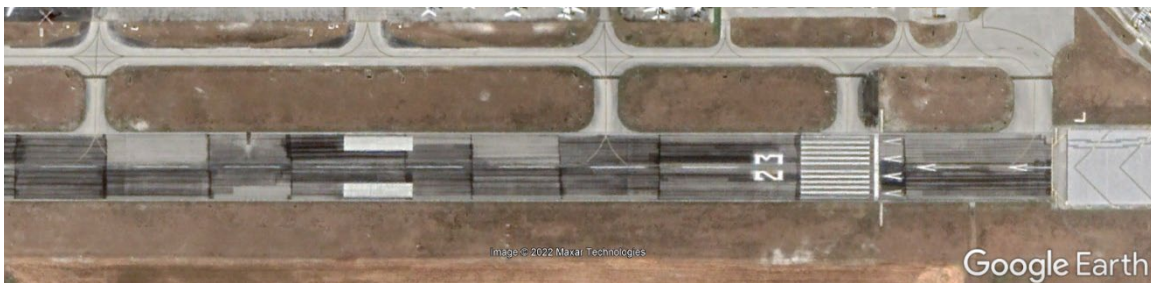
Figure 3. Checkerboard Appearance of P-608-R on BCT Runway 05/23 Approximately 28 Months After Application
