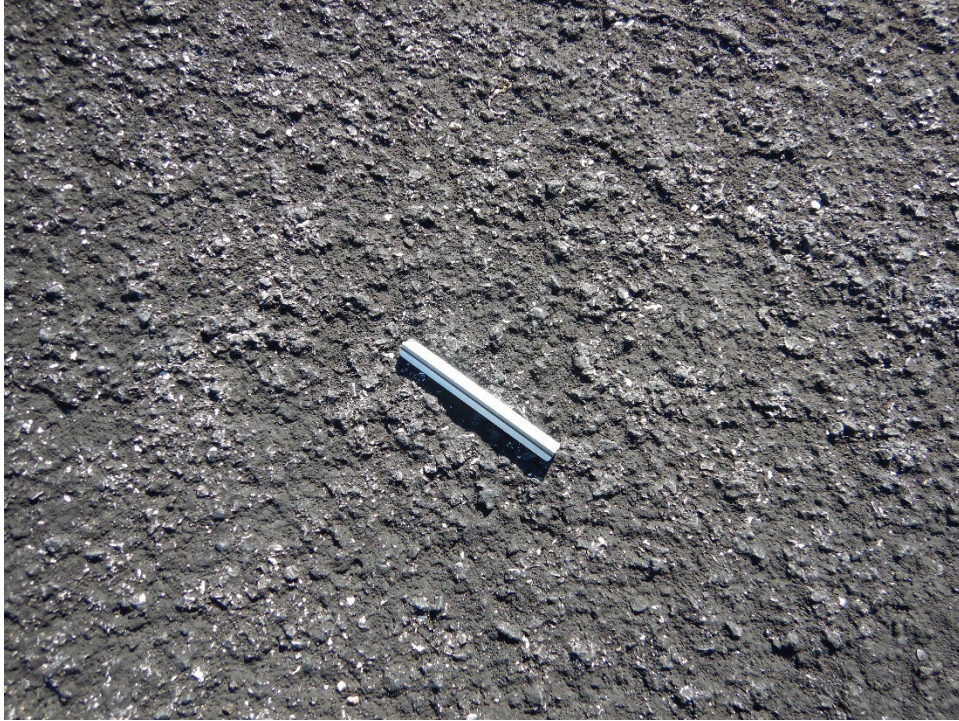
Figure LUG-20. Texture of Taxiway A in High Age Area
