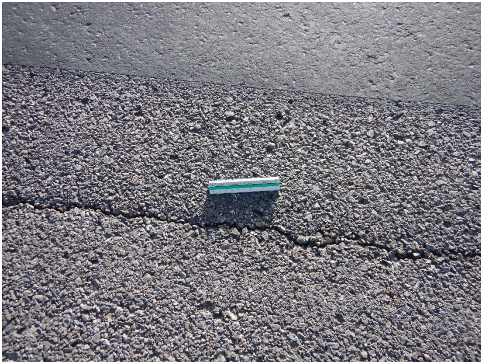
Figure UDOT-12. Sandblasted Area on BTF Runway 17/35
