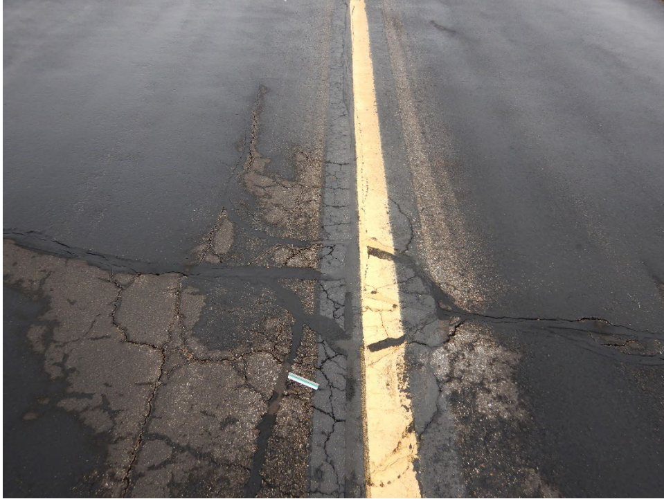
Figure EKO-30. Fatigue Cracking on Taxiway B
