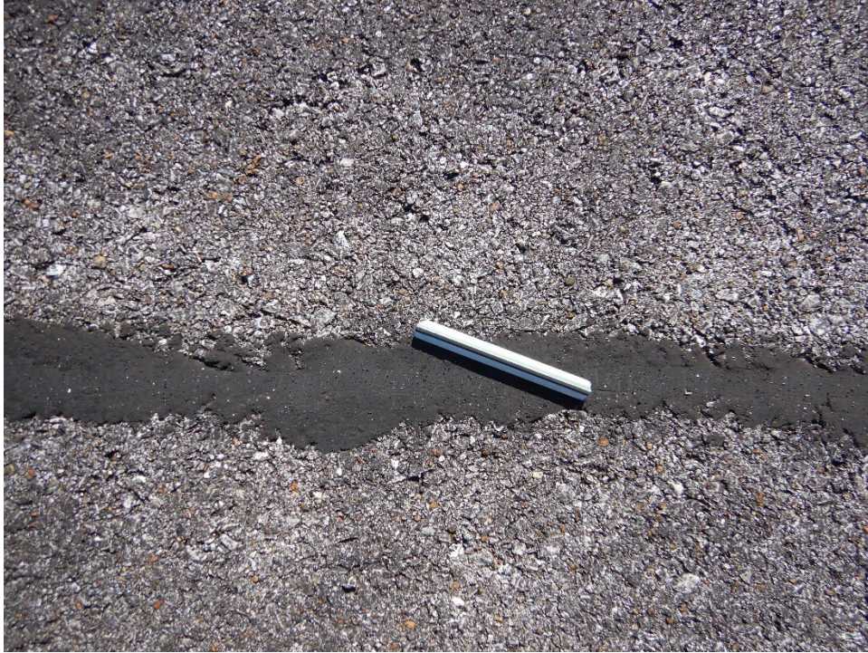
Figure LUG-4. Crack Sealant on Runway 02/20
