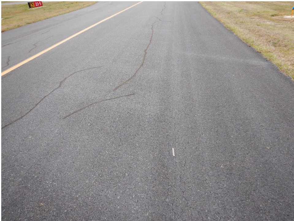
Figure EQY-23. Fatigue Cracking on High Age Taxiway
