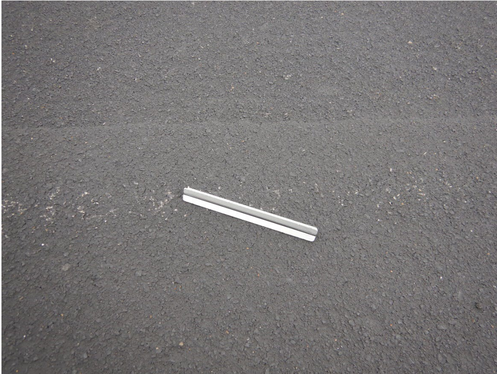
Figure 9. P-629 Texture on M17 Taxiway
