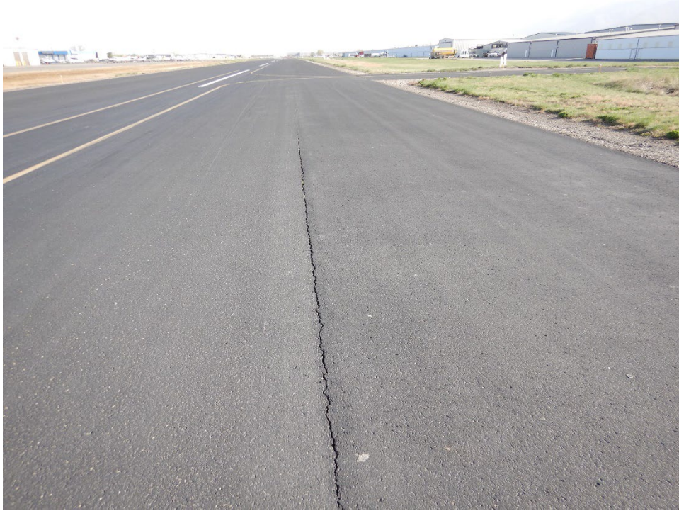
Figure UDOT-9. Opened Longitudinal Paving Joint on BTF Runway 17/35
