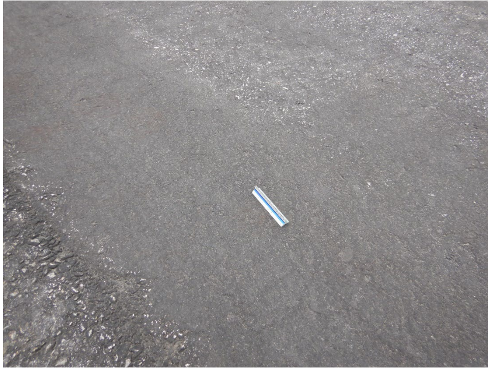
Figure UDOT-39. Thick Coal Tar Fog Seal Application on BMC Taxiway (Rehabilitated in 2006)
