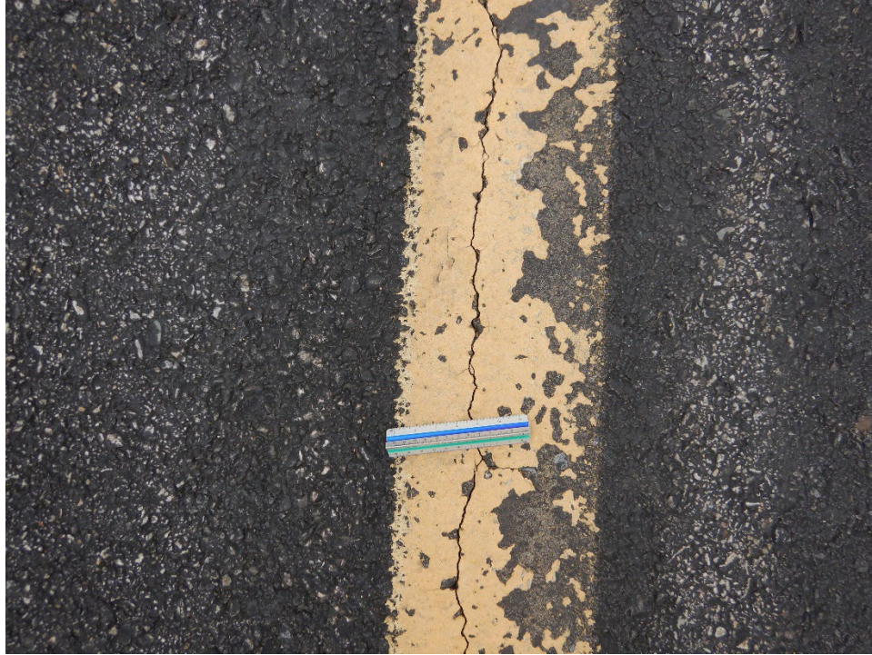
Figure UDOT-31. BMC Taxiway (Rehabilitated in 2008) Longitudinal Paving Joint
