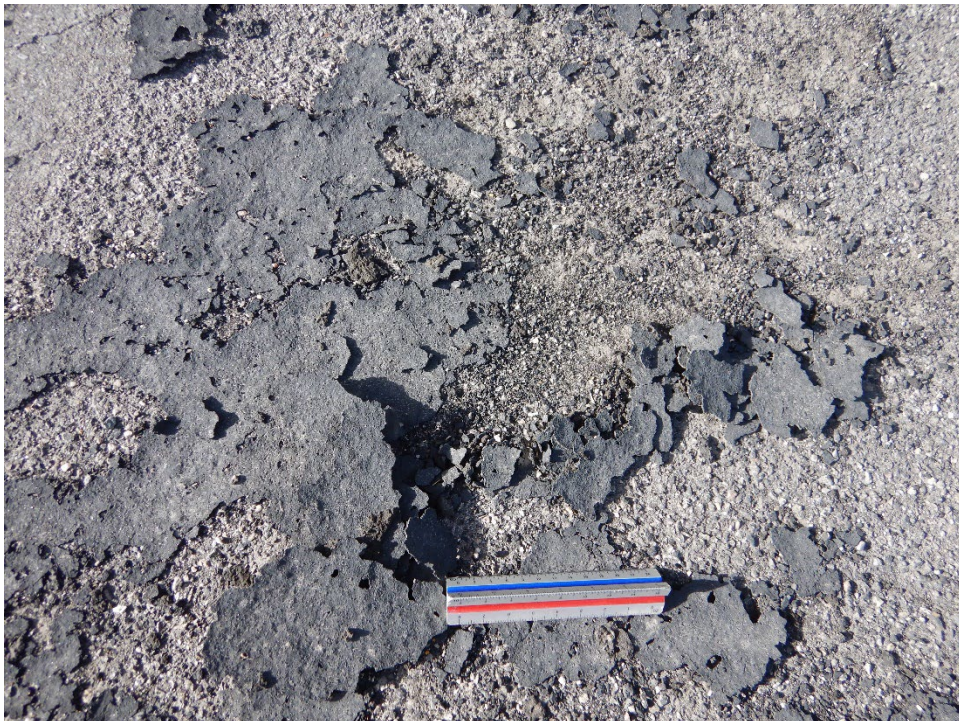
Figure UDOT-14. Debonding on BTF Apron
