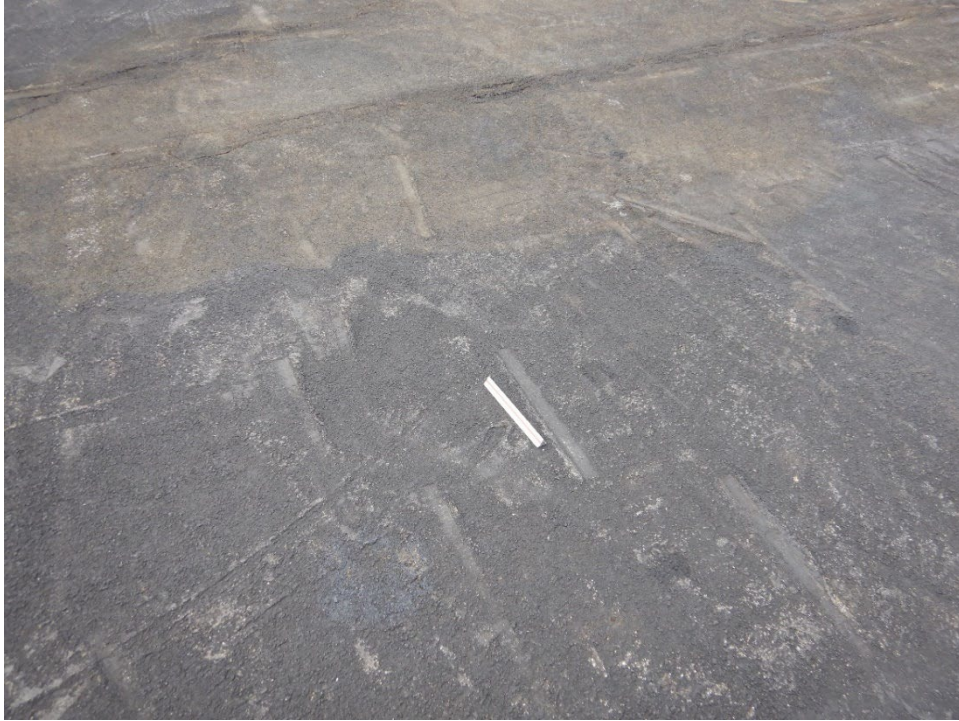
Figure MoDOT-7. Helicopter Skid Indentation on P-629
