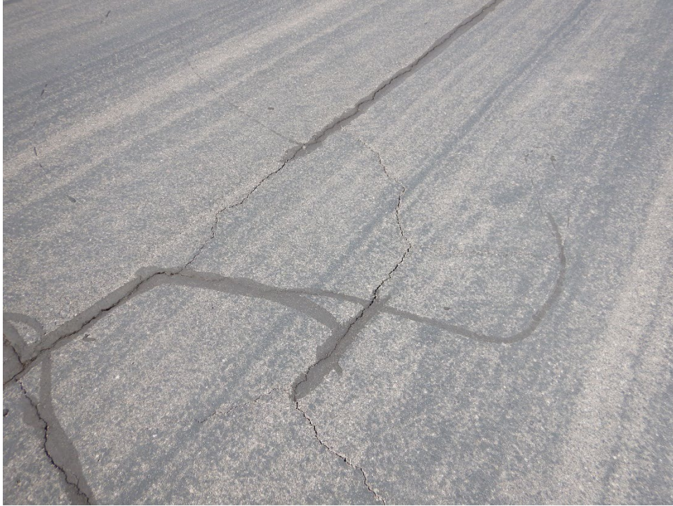
Figure PHX-12. Crack Development on East Cargo Apron
