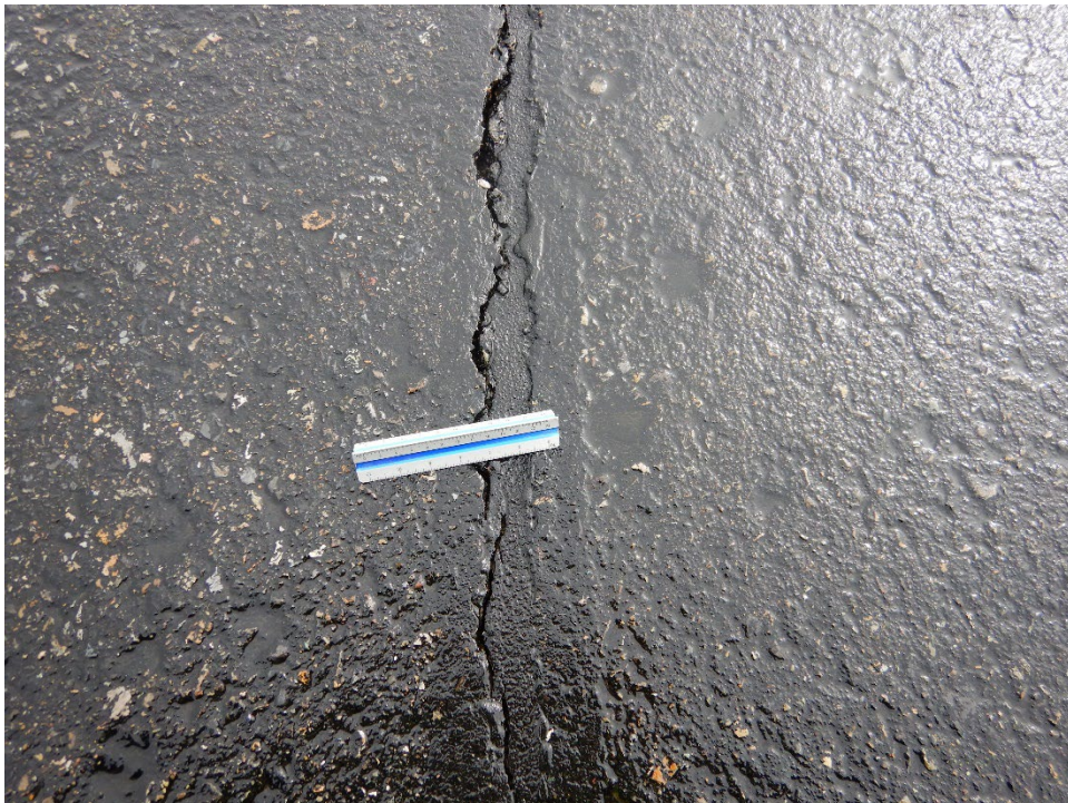
Figure EKO-13. Failed Crack Sealant on Taxiway A
