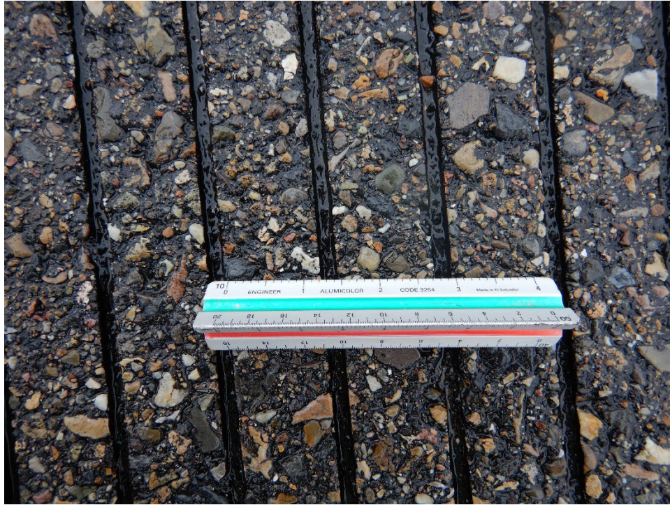
Figure EKO-3. P-608 Condition Between and Within Runway 06/24 Grooves
