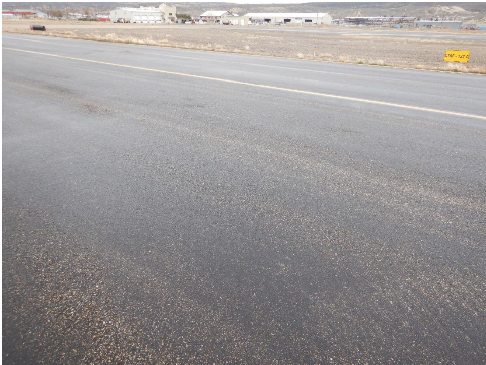
Figure EKO-19. P-608 Streaking on Apron
