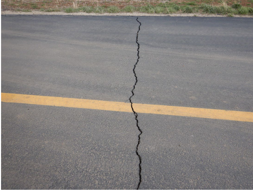
Figure UDOT-25. Transverse Crack on 42U Taxiway
