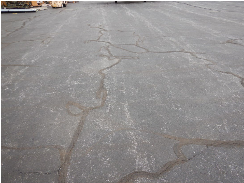
Figure UDOT-43. Block Cracking on BMC Apron
