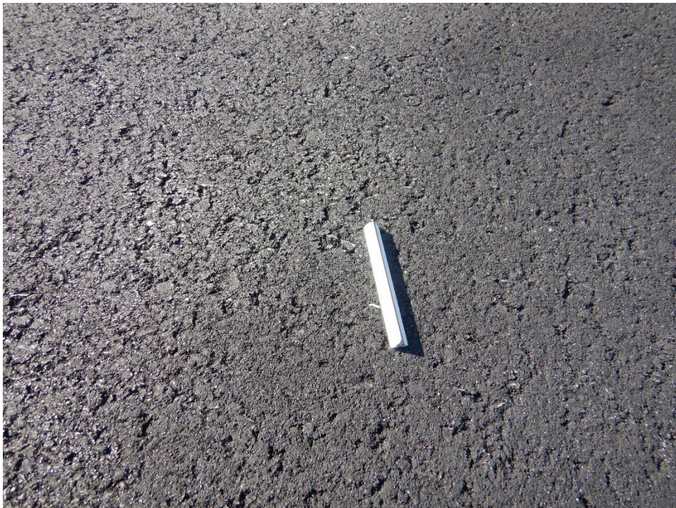
Figure LUG-9. P-608 Texture on T-Hangar Pavement
