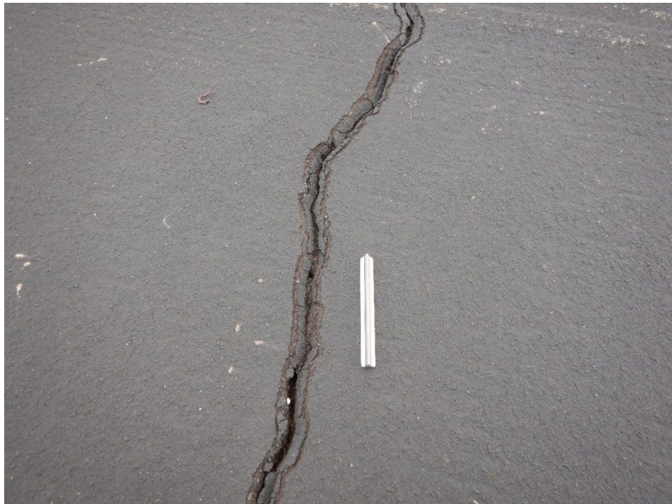
Figure MoDOT-10. M17 Taxiway Cracking With Failed Sealant
