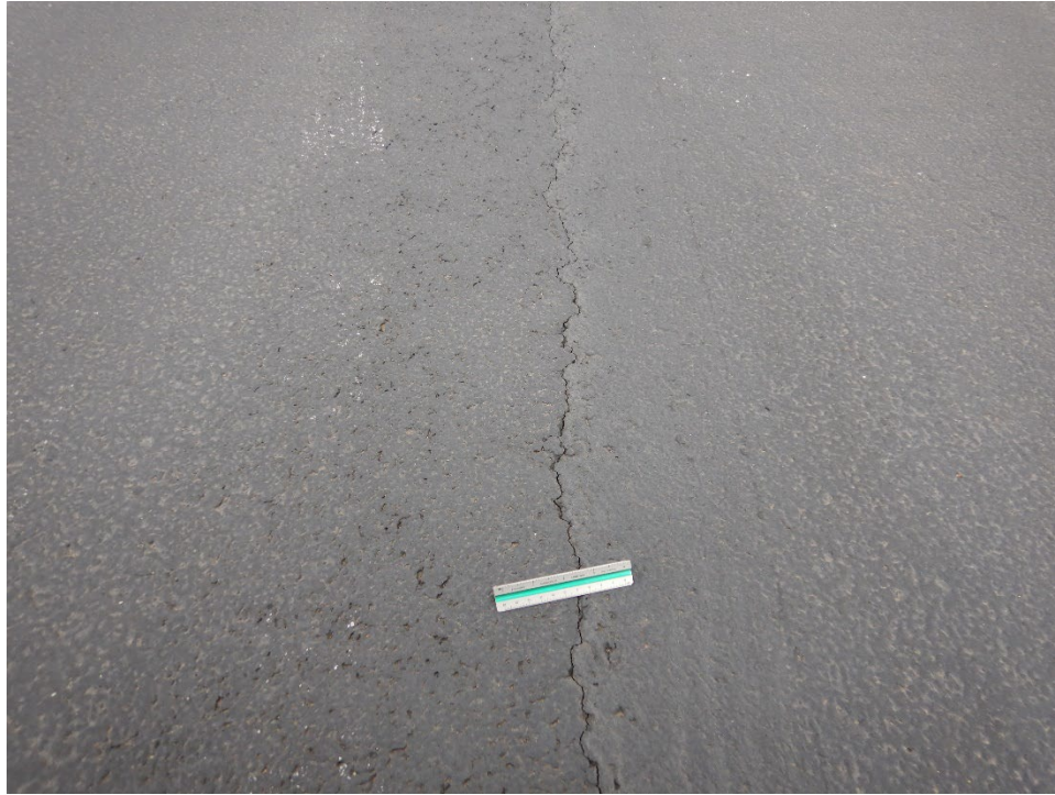
Figure UDOT-21. Closeup of Longitudinal Paving Joint on 42U Runway 03/21
