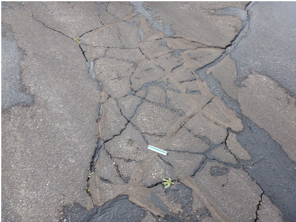
Figure EKO-25. Fatigue Cracking on Runway 12/30
