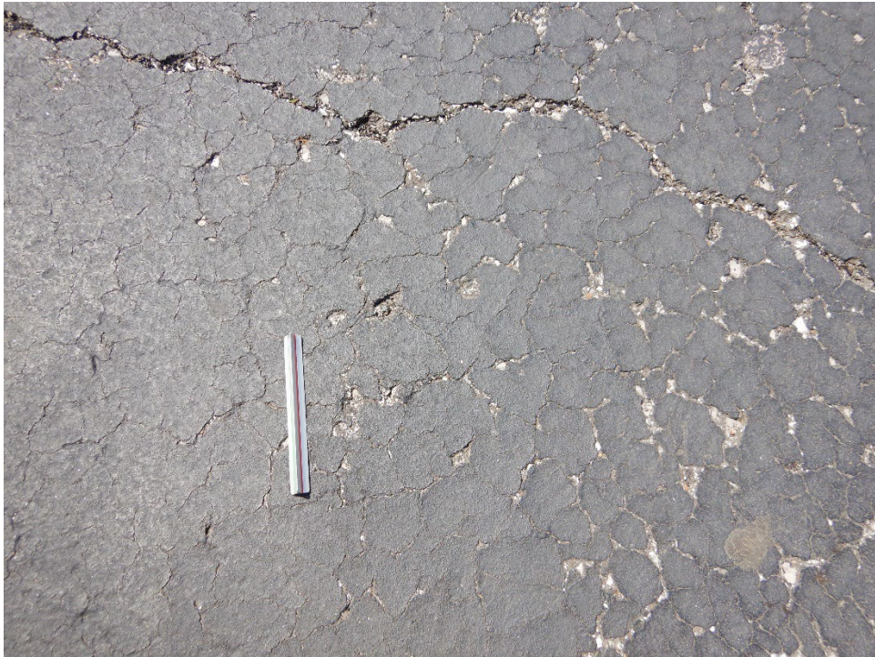
Figure GZS-13. Raveling on Apron
