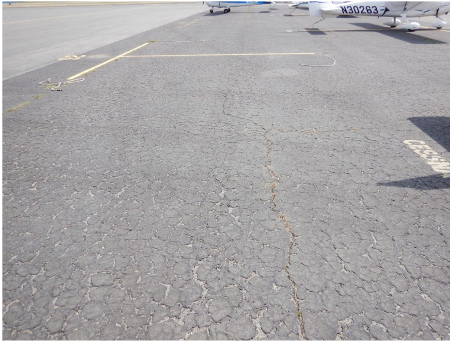
Figure EQY-1. Apron Overview with Coal Tar Slurry
