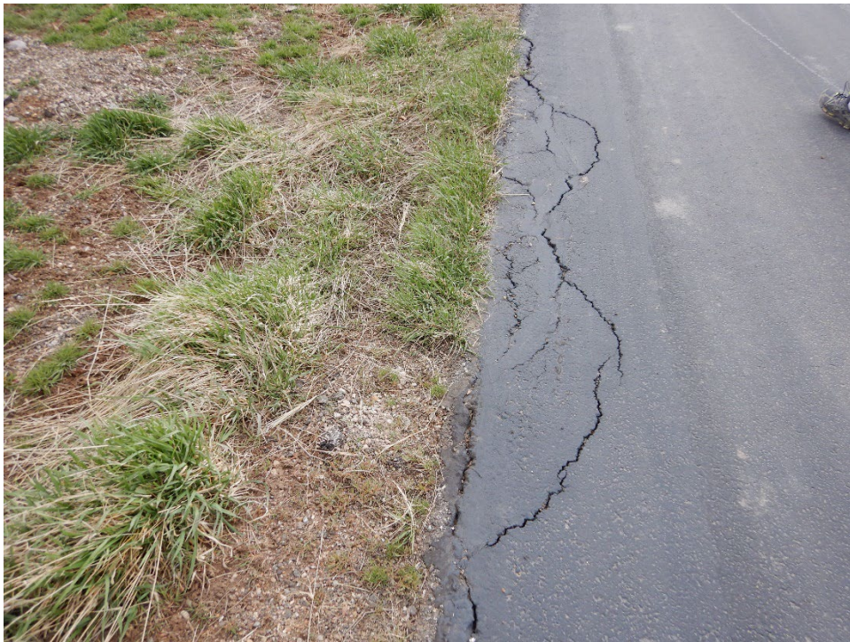
Figure UDOT-26. Edge Cracking on 42U Taxiway
