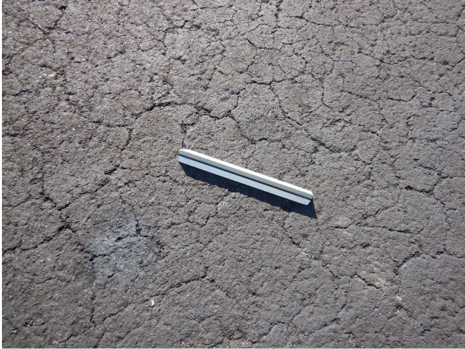
Figure LUG-15. Map Cracking on Apron
