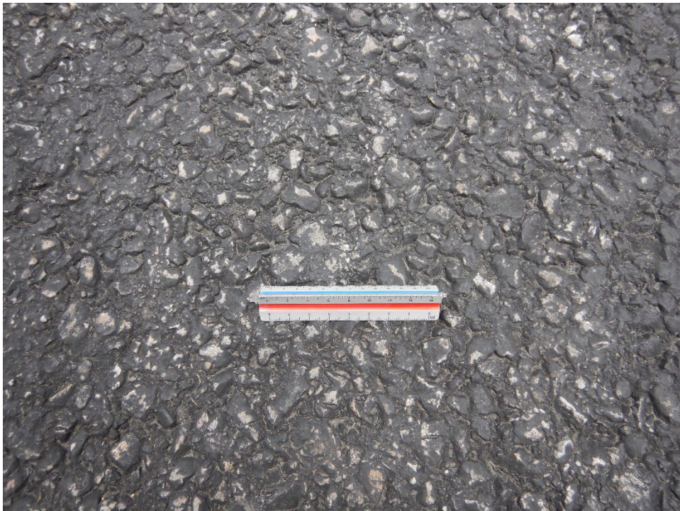
Figure UDOT-38. Snowplow Wear on BMC Taxiway (Rehabilitated in 2006)
