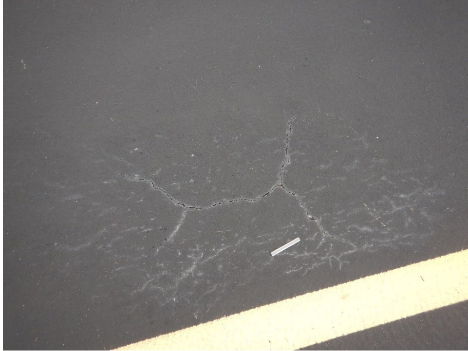
Figure MoDOT-9. Possible Fatigue Cracking on P-629
