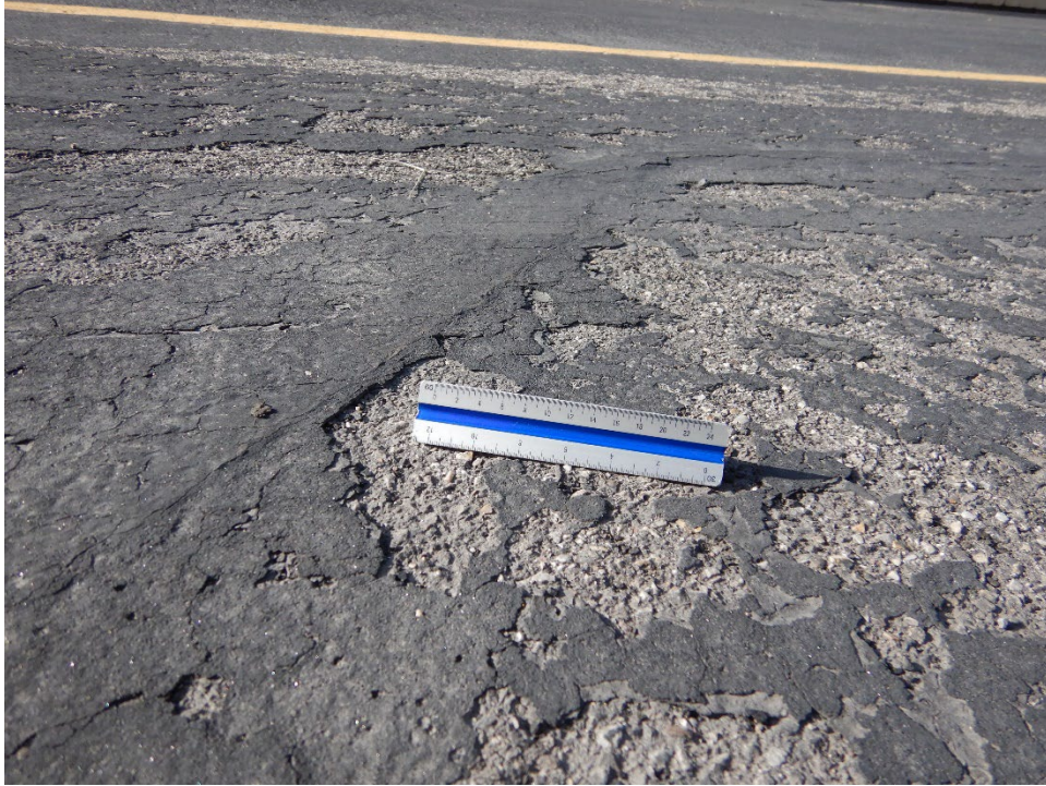
Figure UDOT-15. Raveling on BTF Apron
