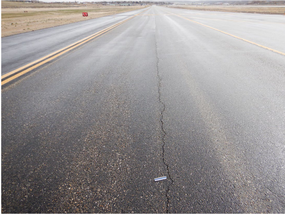
Figure EKO-12. Opened Longitudinal Joint on Taxiway A
