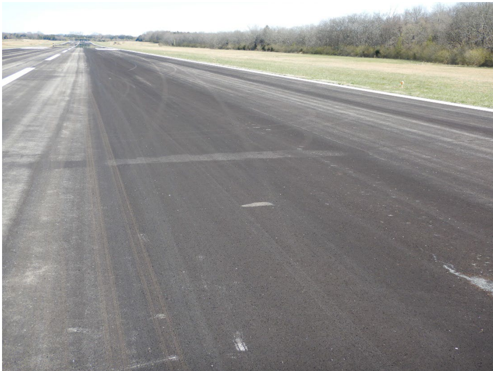
Figure LUG-5. Tire Tracks on Runway 02/20
