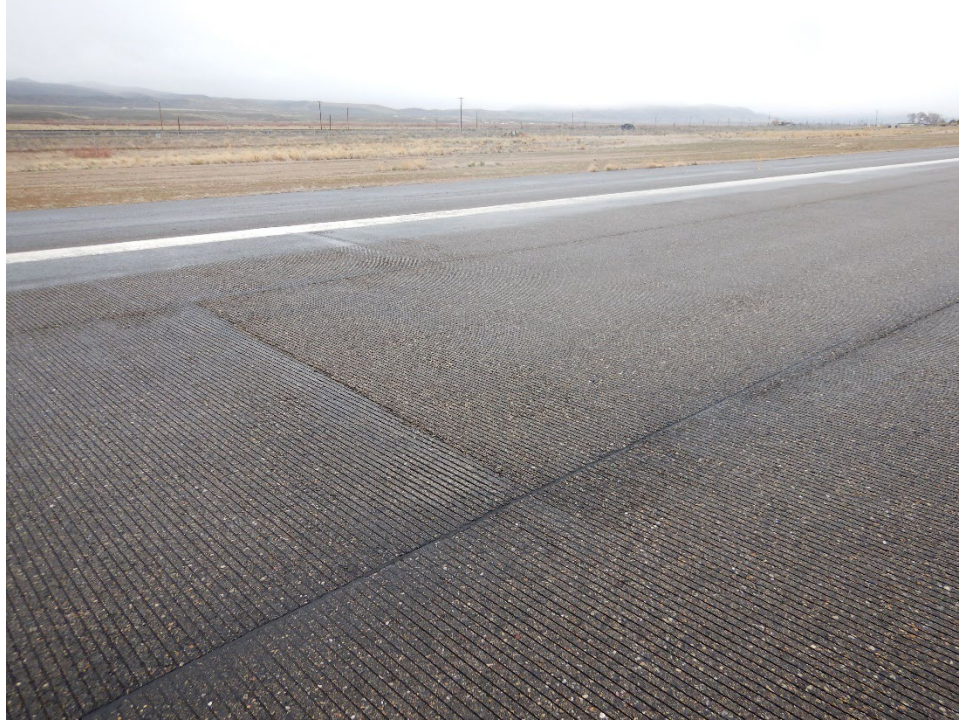
Figure EKO-7. Transverse Construction Joint on Runway 06/24
