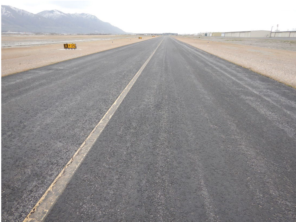
Figure UDOT-34. Overview of BMC Taxiway (Rehabilitated in 2006) With Coal Tar Fog Seal
