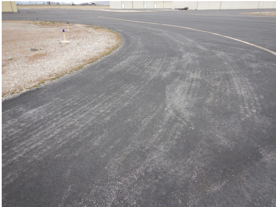
Figure UDOT-32. BMC Taxiway (Rehabilitated in 2008) Showing Uneven Coverage of Coal Tar Fog Seal
