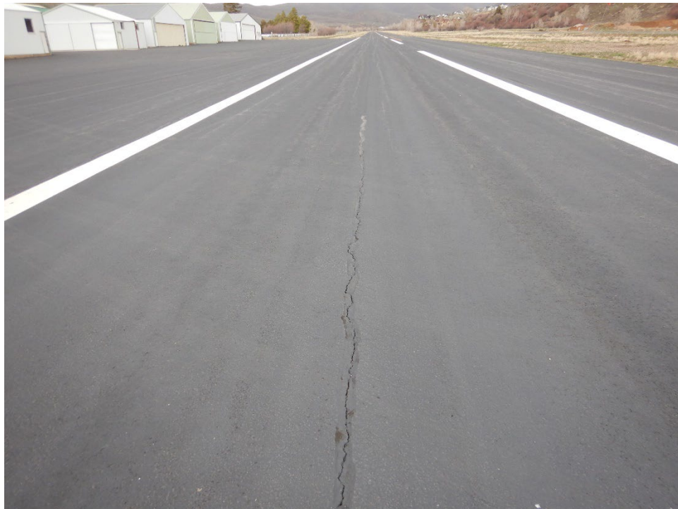
Figure UDOT-20. 42U Runway 03/21 Longitudinal Paving Joint
