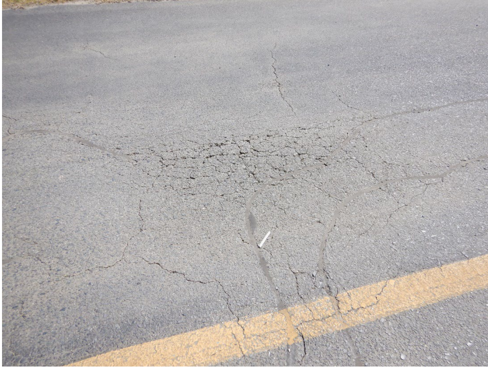
Figure EQY-22. Depression and Fatigue Cracking on High Age Taxiway
