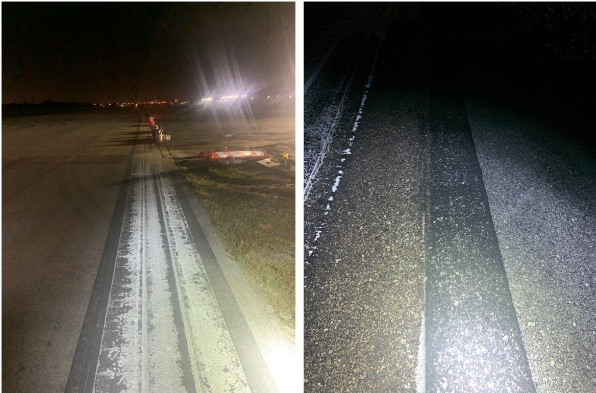
Figure BCT-3. Runway 05/23 Peeling Pavement Marking
