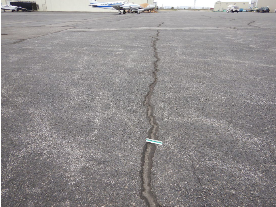
Figure UDOT-42. L&T Cracking on BMC Apron
