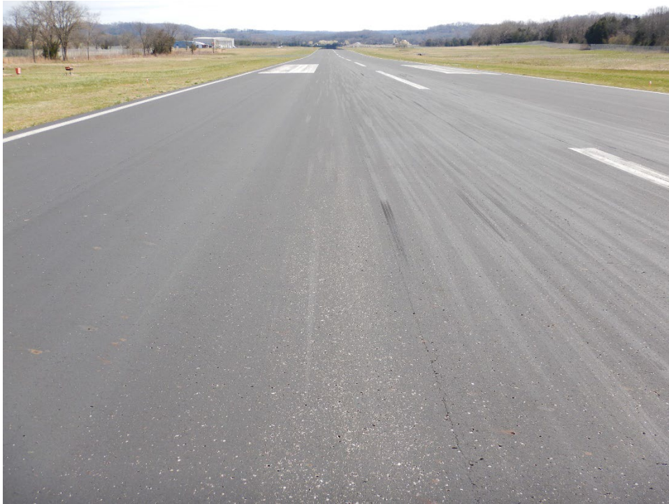
Figure 2. Tire Wear Pattern on GZS Runway
