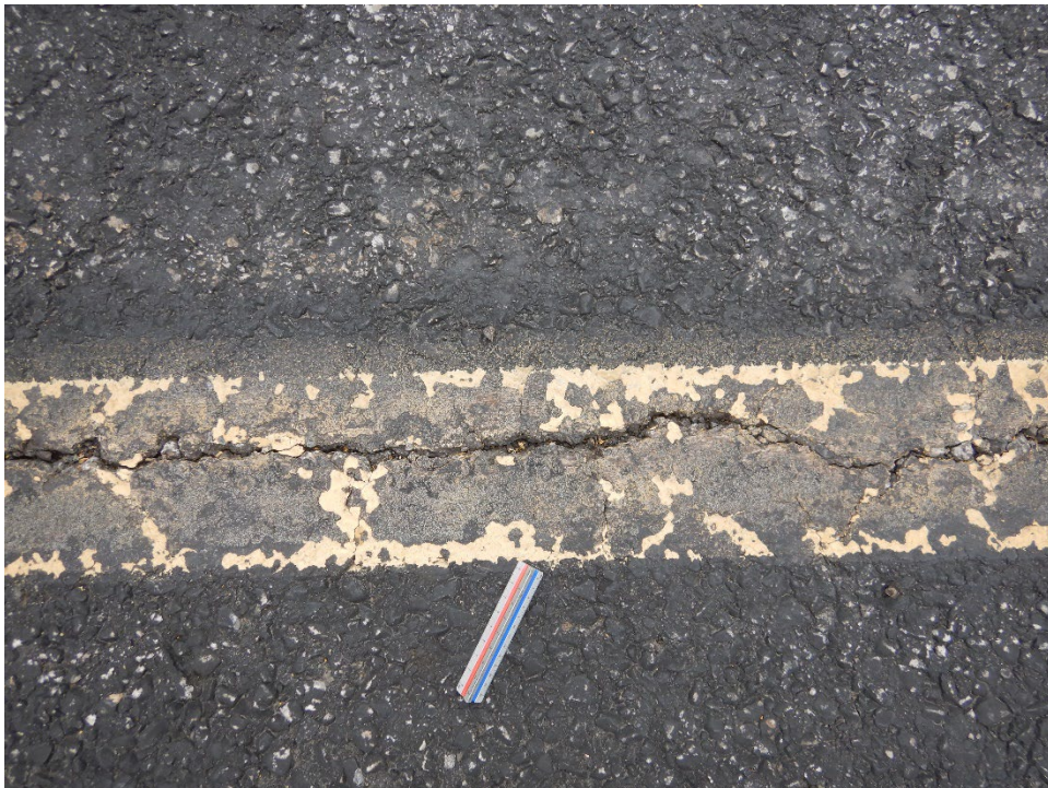
Figure UDOT-36. BMC Taxiway (Rehabilitated in 2006) Longitudinal Paving Joint
