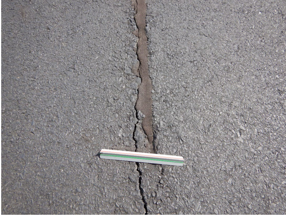
Figure EQY-14. Cracking on Medium Age Taxiway
