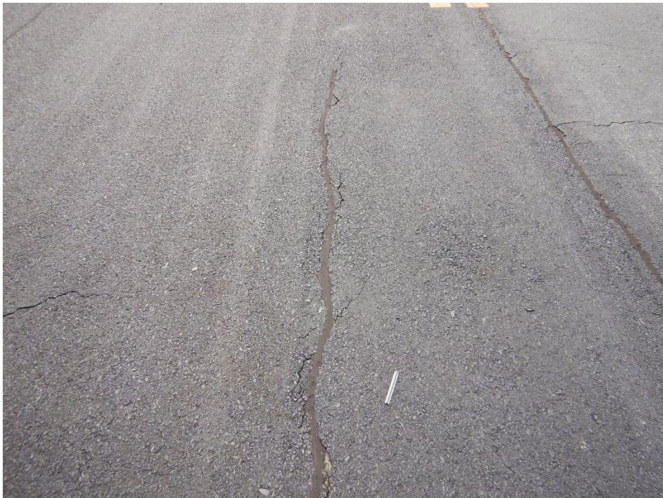
Figure EQY-21. Cracking on High Age Taxiway
