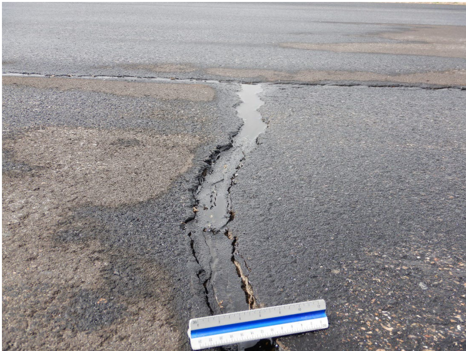
Figure EKO-23. Crack Sealant Condition on Runway 12/30
