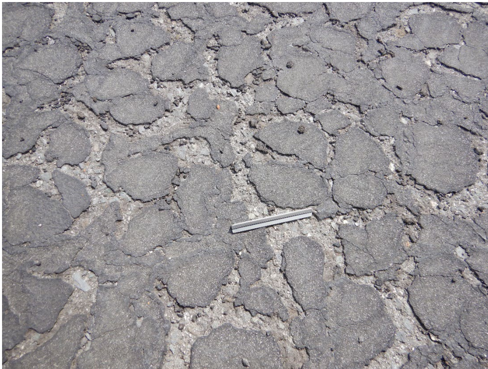
Figure EQY-4. Severe Map Cracking with Coal Tar Slurry
