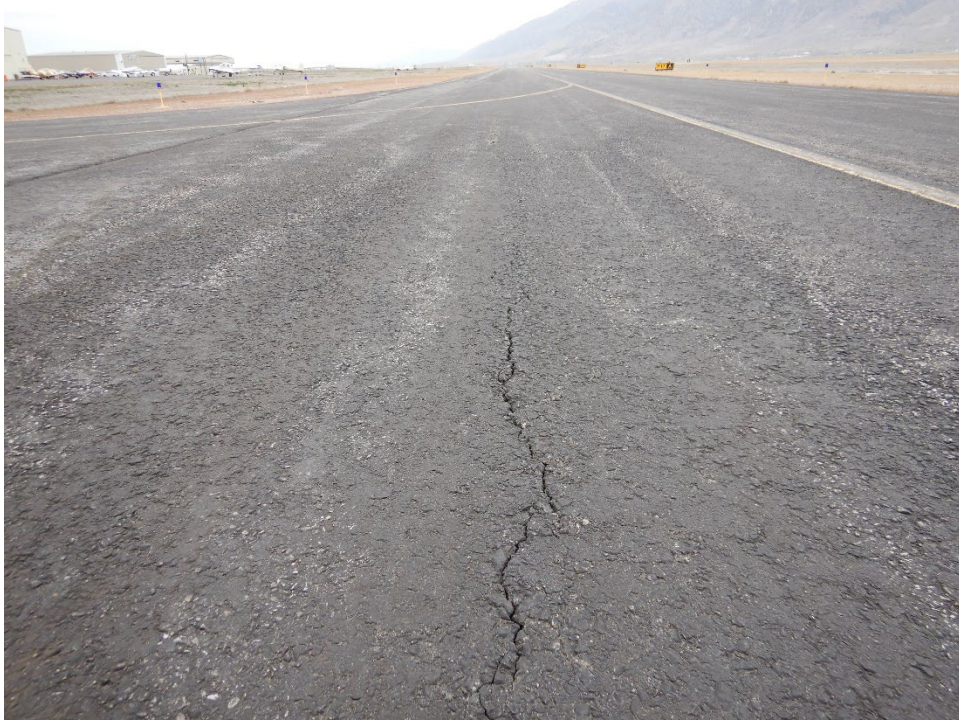
Figure UDOT-37. Wheelpath Cracking on BMC Taxiway (Rehabilitated in 2006)
