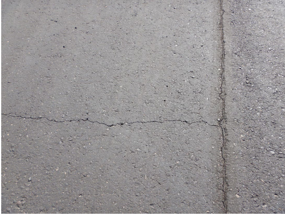
Figure PHX-8. New Cracking on Taxiway A
