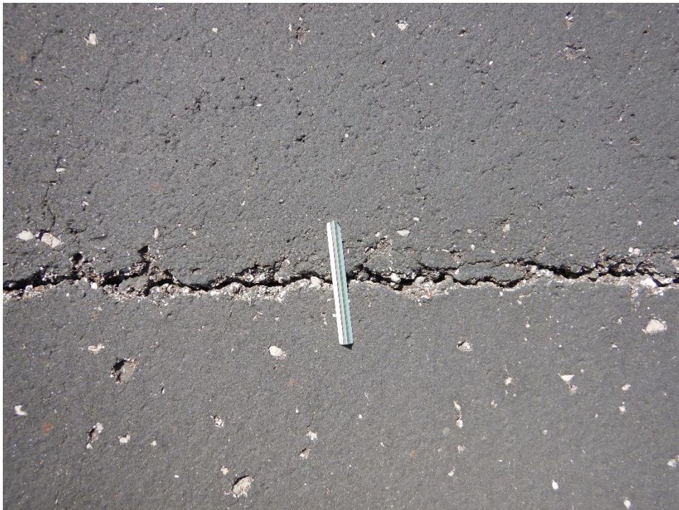
Figure GZS-5. Cracking on Runway 16/34
