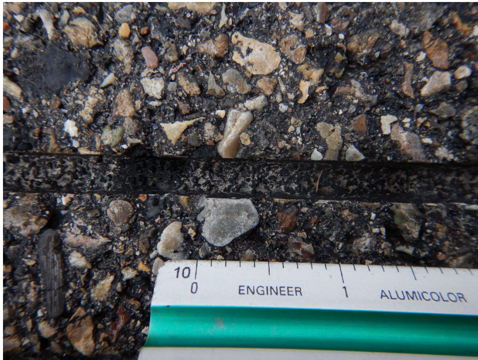
Figure 5. P-608 Material Visible in EKO Runway 06/24 Groove
