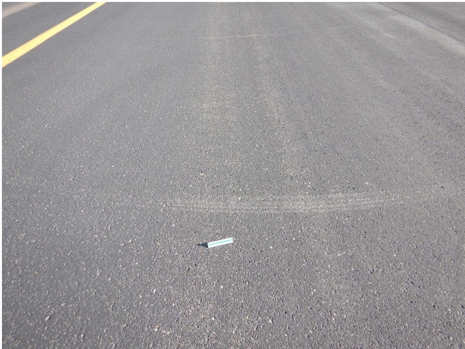
Figure UDOT-6. Slight Wear of Onyx on BTF Runway 17/35
