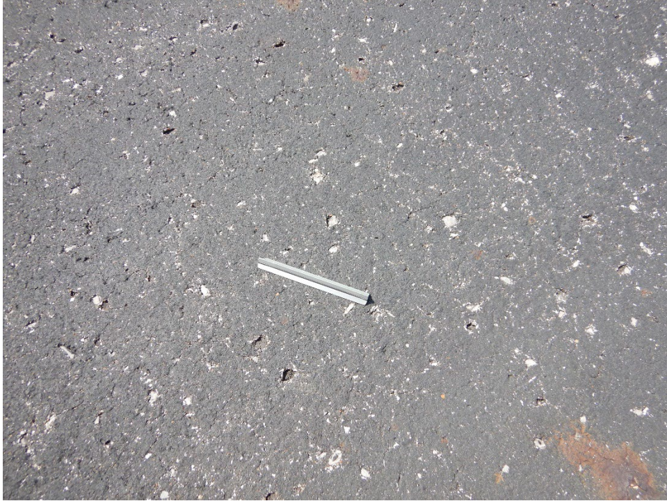
Figure GZS-6. Raveling on Runway 16/34
