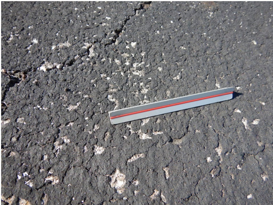
Figure MoDOT-20. LLU Runway 03/21 Raveling
