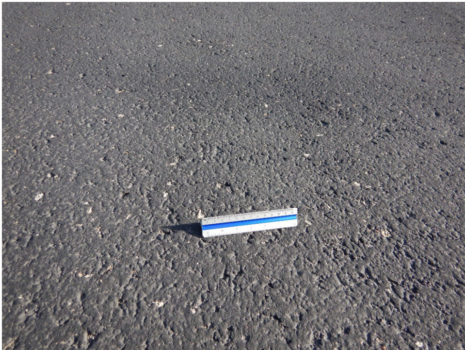
Figure UDOT-8. Exposed Coarse Aggregate on BTF Runway 17/35
