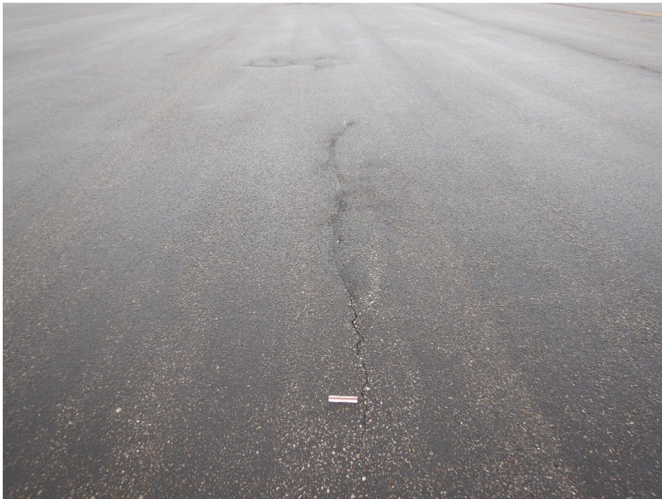
Figure EKO-17. Cracking Development on Apron
