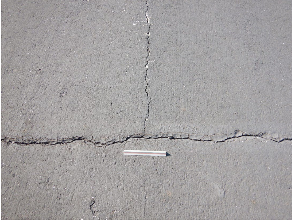
Figure MoDOT-19. LLU Runway 03/21 Cracking
