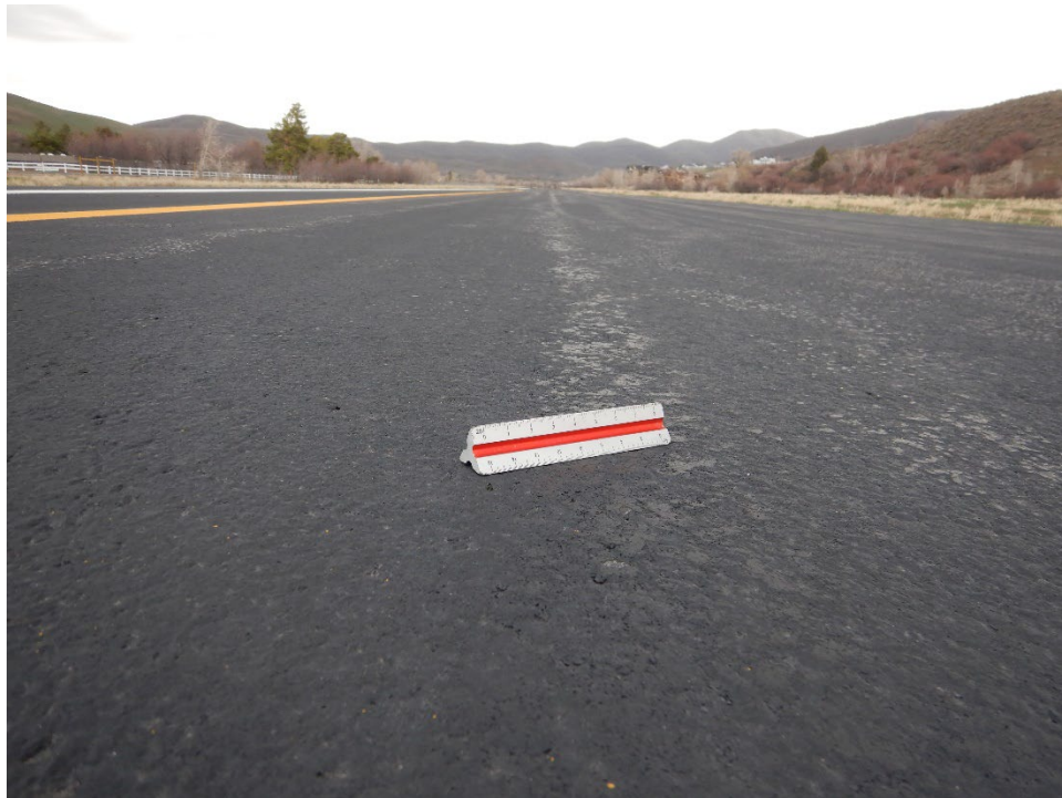
Figure UDOT-22. Surface Smoothing Due to Snowplowing on 42U Runway 03/21
