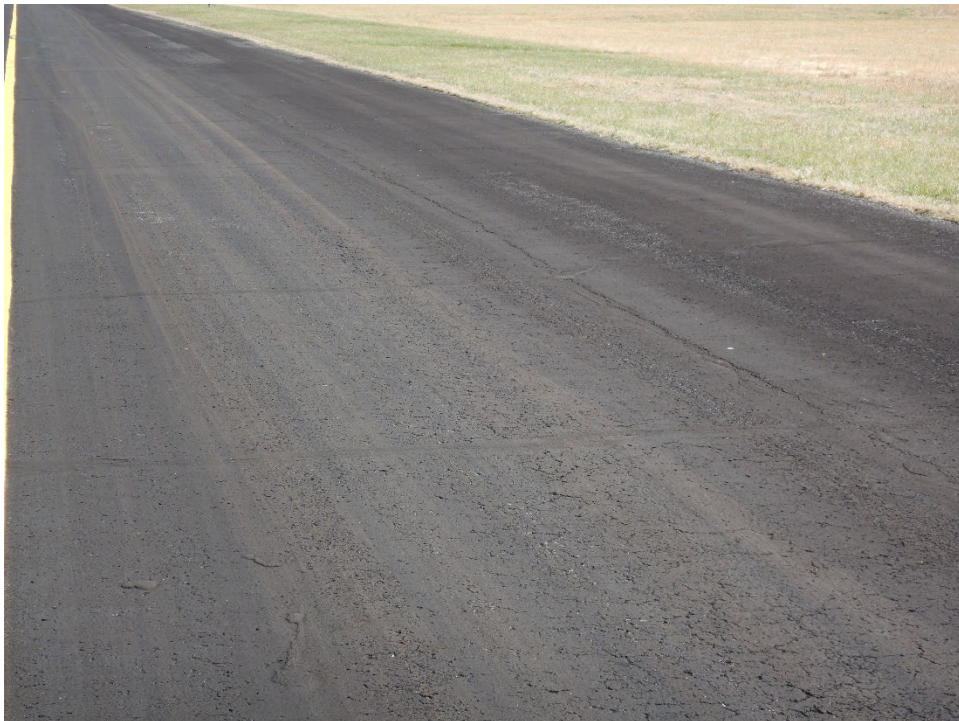
Figure LUG-21. Tire Tracks on Taxiway A in High Age Area
