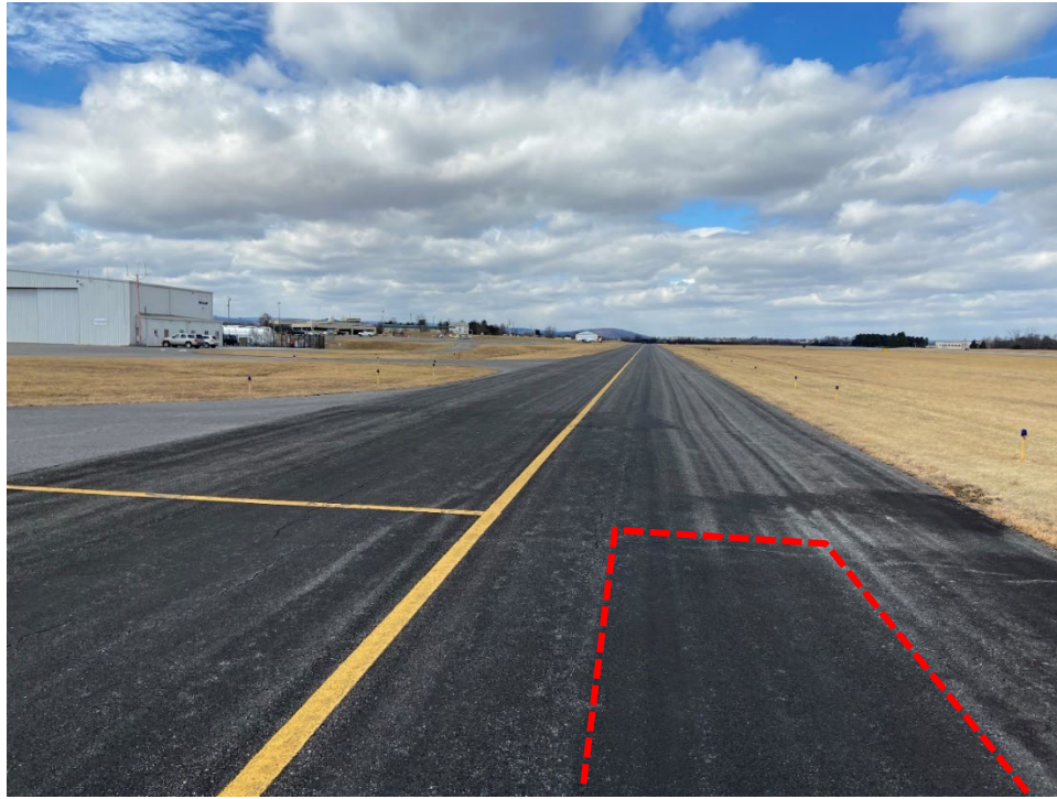
Figure OKV-1. Typical P-608 Application and Overlap (Red Dashed Rectangle) on Taxiway A—February 2022
