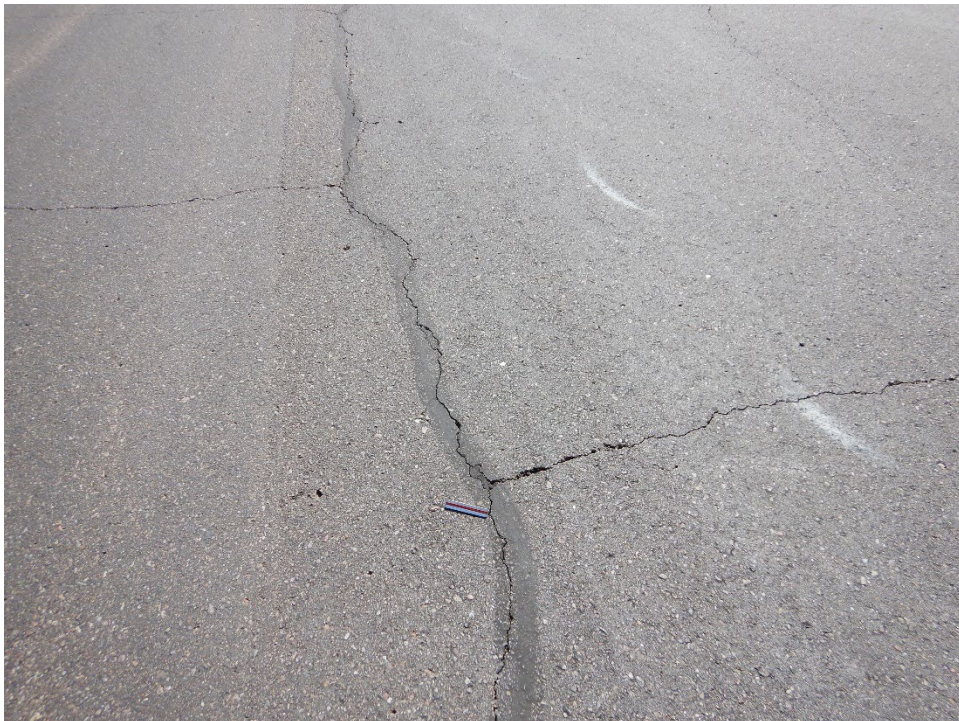
Figure PHX-4. New Crack Formation on West Cargo Apron
