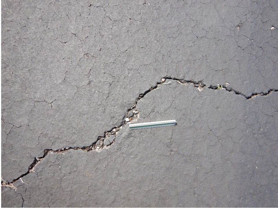
Figure GZS-12. Cracking on Apron
