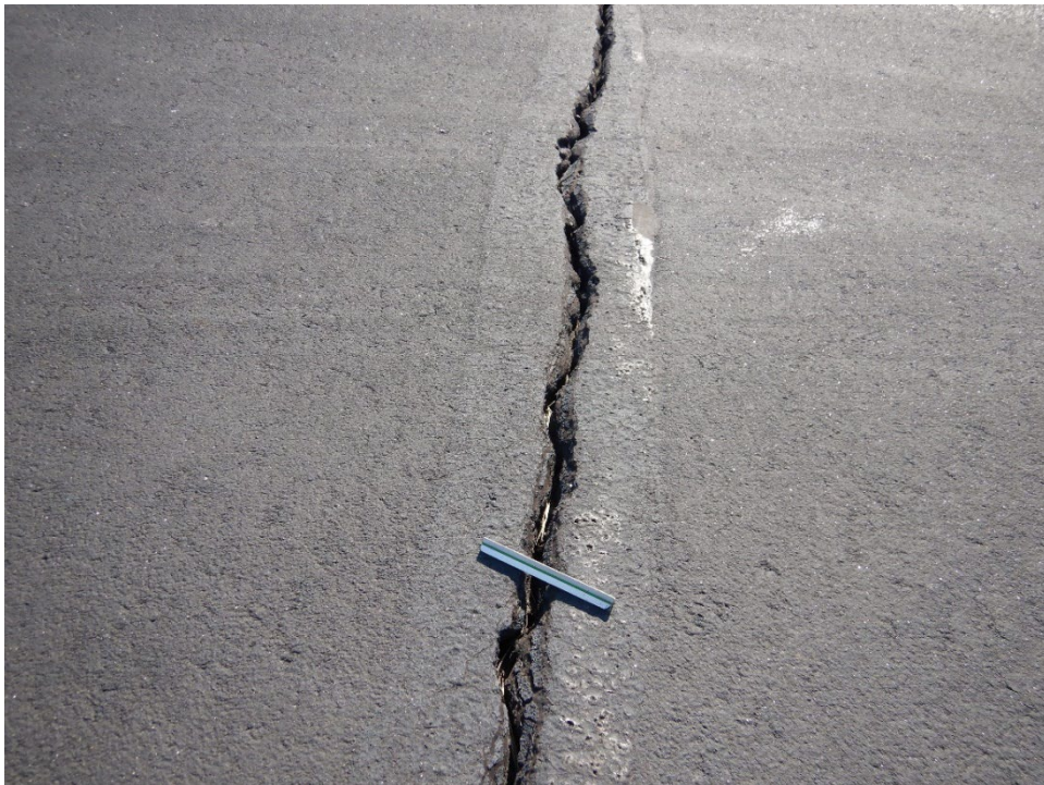
Figure MoDOT-18. LLU Runway 03/21 Cracking With Failed Sealant
