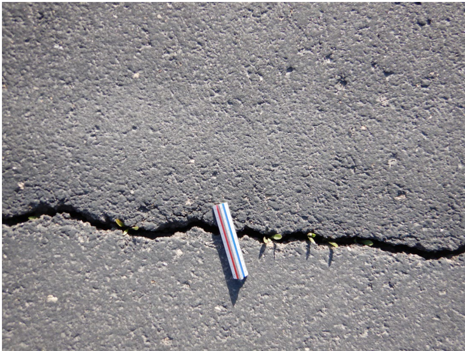
Figure UDOT-10. Closeup of Opened Longitudinal Paving Joint
