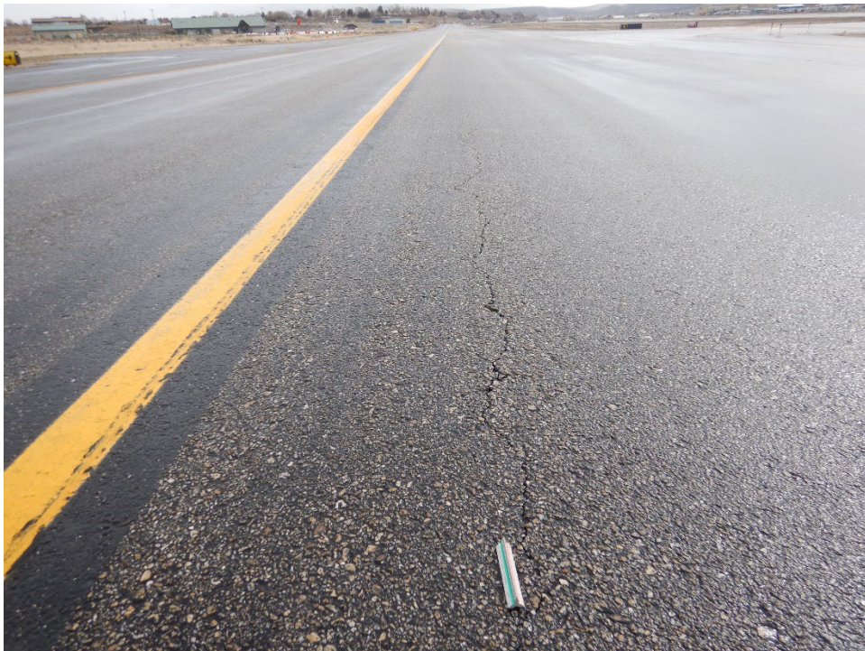
Figure EKO-11. Wheelpath Cracking on Taxiway A
