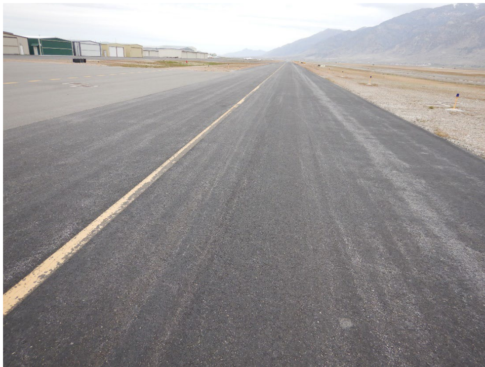
Figure UDOT-28. Overview of BMC Taxiway (Rehabilitated in 2008) With Coal Tar Fog Seal
