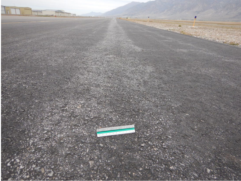
Figure UDOT-33. Snowplow Wear on BMC Taxiway (Rehabilitated in 2008)
