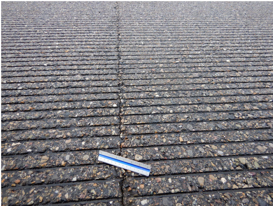
Figure EKO-6. Cracked Longitudinal Paving Joint on Runway 06/24
