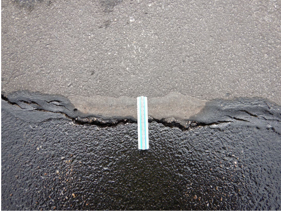
Figure EKO-24. Failed Crack Sealant on Runway 12/30
