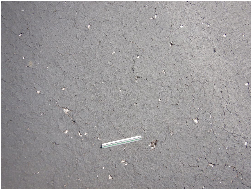
Figure GZS-11. Map Cracking on Apron
