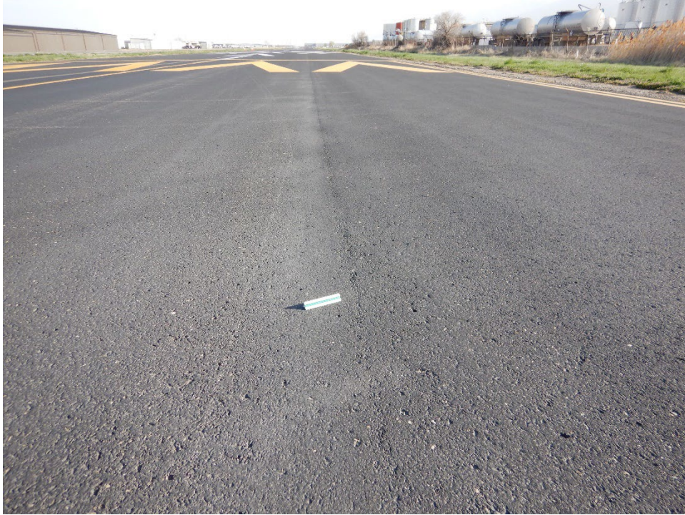
Figure UDOT-11. Closed Longitudinal Paving Joint on BTF Runway 17/35
