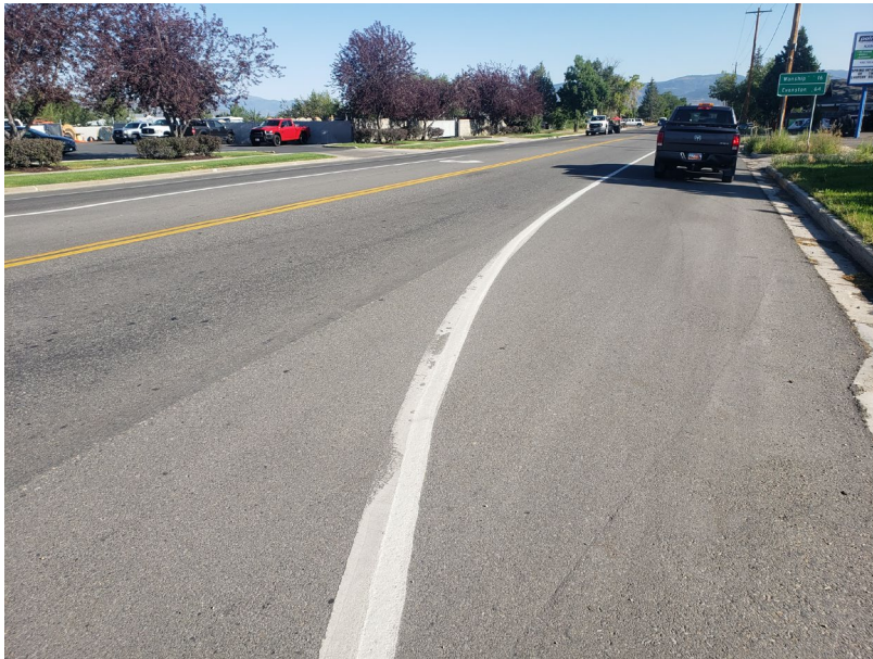
Figure 3.3 Section UT-04 Showing some joint opening
