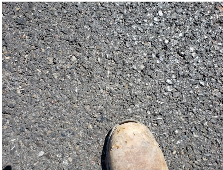
Figure 3.1 Section UT-02 showing fatigue cracking and raveling
