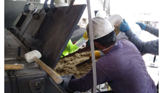
Fibers are added after mortar is mixed to give the concrete more strength, ductility, and tensile capacity.
