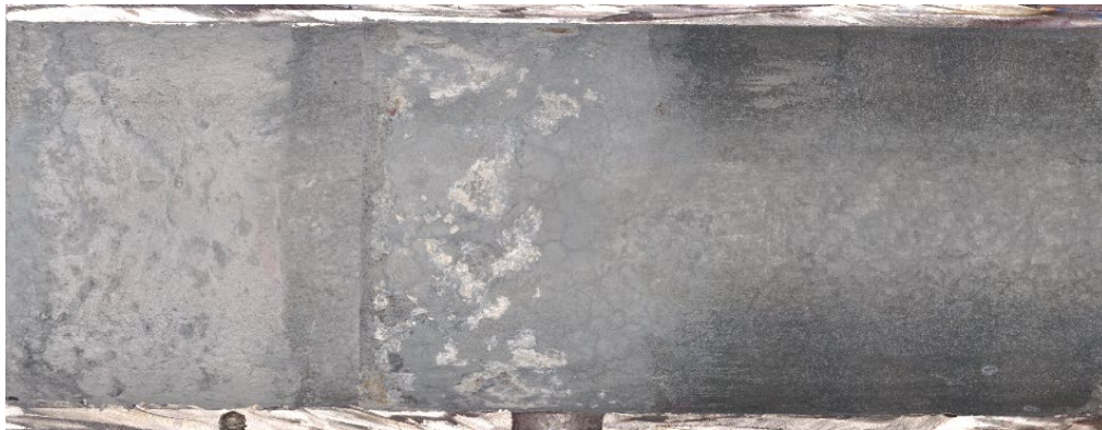
Figure 5-5. Inside view of the galvanized duct from Tendon 5 with very soft grout ( w/c = 0.5 ).
