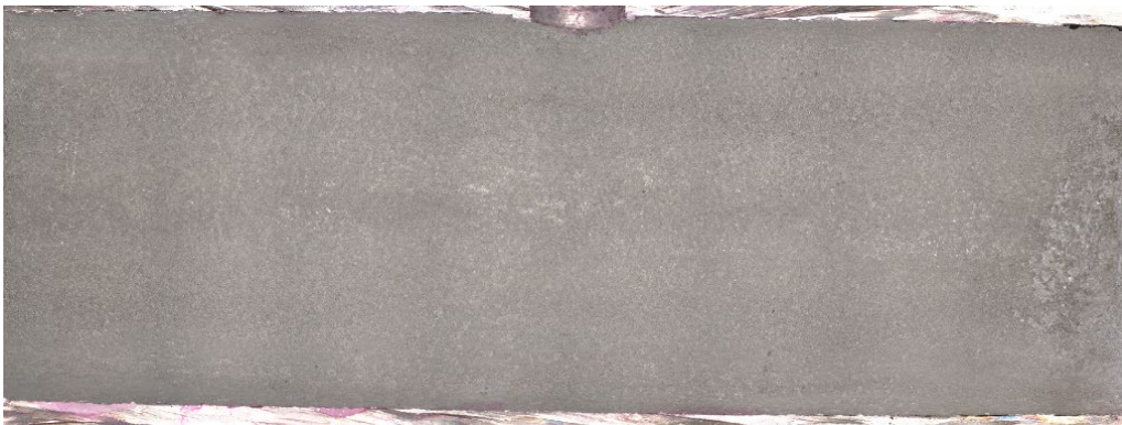
Figure 5-3. Inside view of the galvanized duct from Tendon 1 with good grout ( w/c = 0.28 ).
