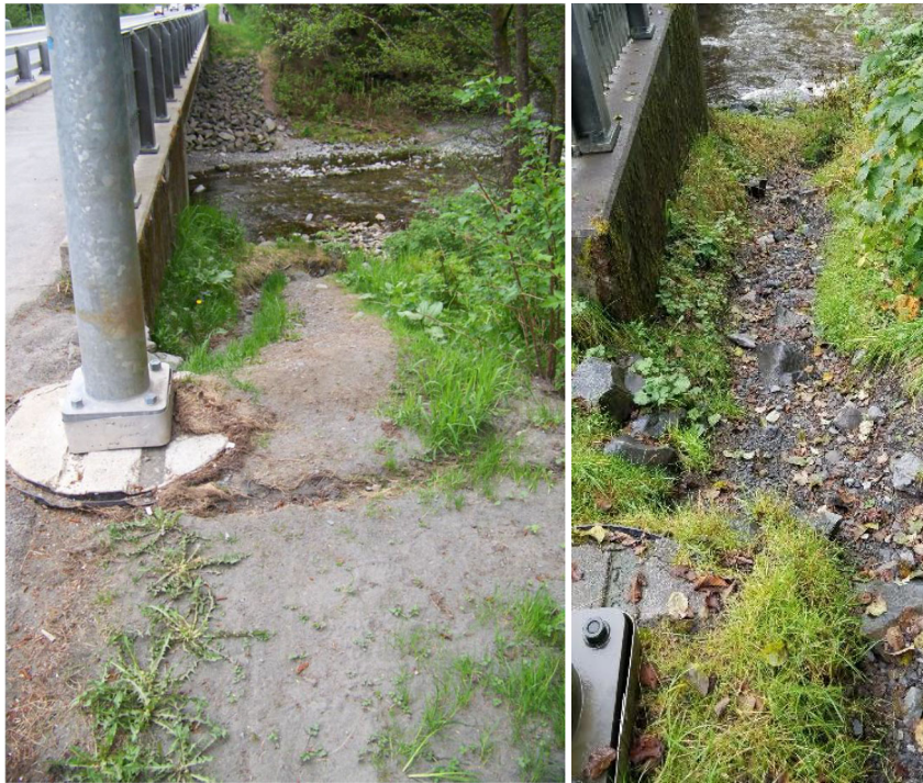
Figure 8 - (L) Trail connection in 2014. Water started to wear channels into the soil. Figure 9 - (R) Trail connection in 2018. Trail surface has continued to deteriorate and large rocks are starting to show through. The surface is very loose with uneven footing.
