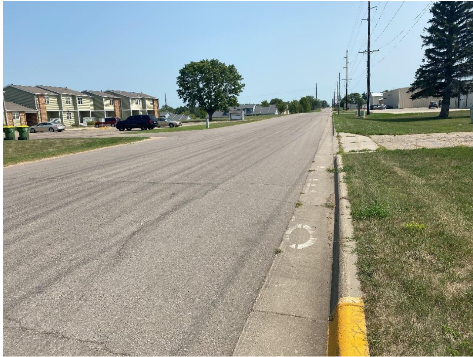
Figure 42. Paved over bike lane in Pipestone, Minnesota.
