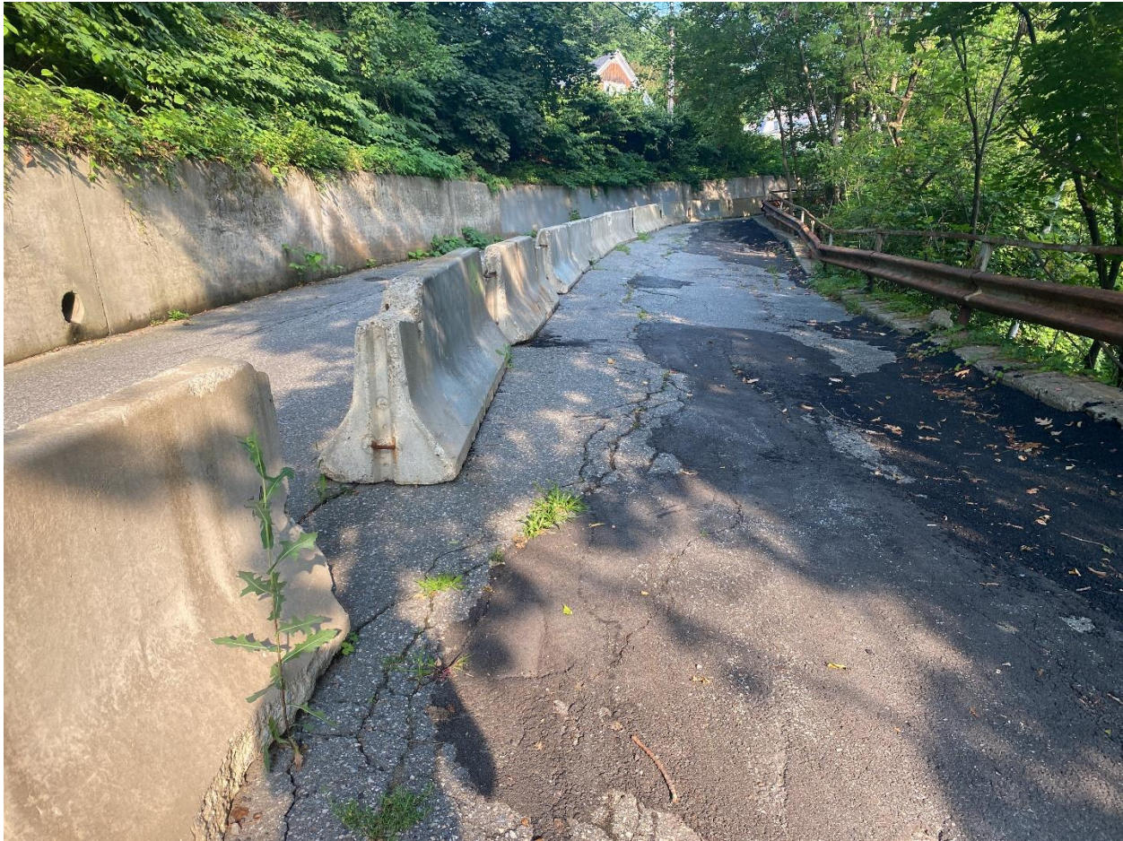
Figure 33. Aging infrastructure, Town of Hartford, Vermont.
