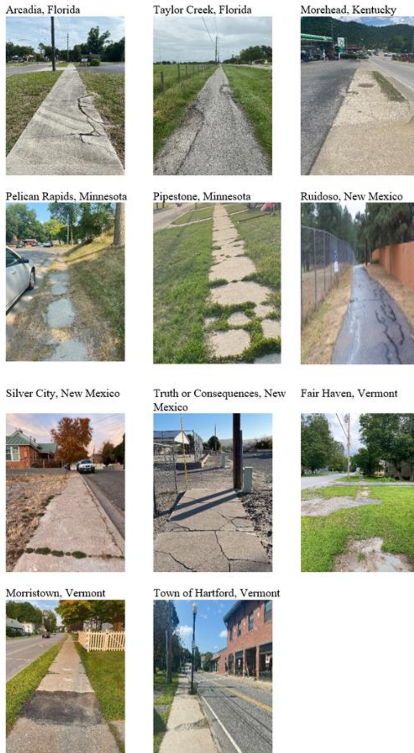
Figure 34. Examples of sidewalks in the case study areas in need of repair.
