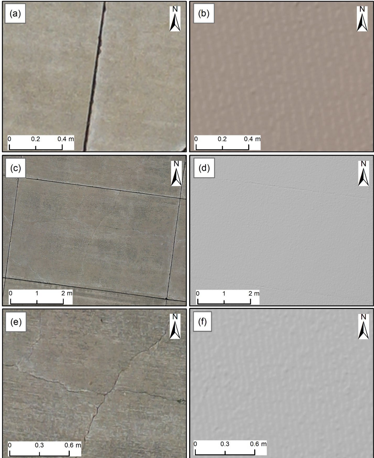
Figure 59. Faulting (L) in (a) 2.5-mm/pix Orthophoto and (b) 10-mm/pix DEM; and Shattered Slabs (M) in (c, e) 2.5-mm/pix Orthophoto and (d, f) 10-mm/pix DEM
