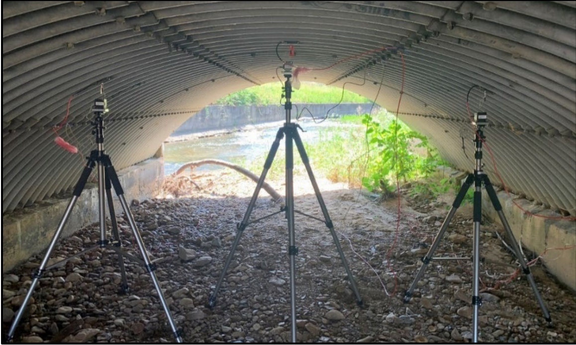
Figure 5.28. Potentiometers installed at \frac{1}{4} , crown and \frac{3}{4} locations at Bain's Gap Road culvert.
