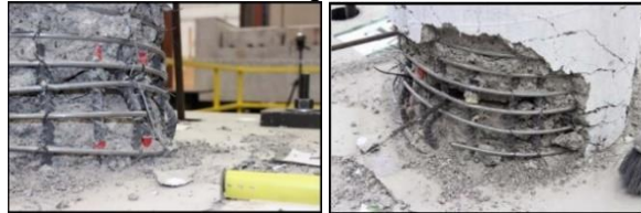
Damage State III
