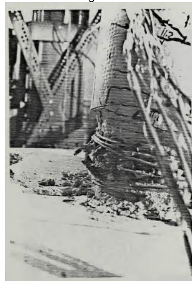
Damage State VI (8.95%)
