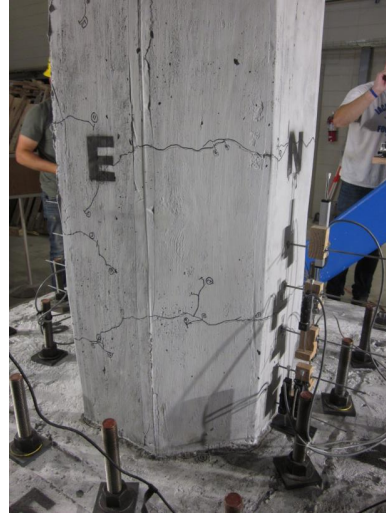
(b) Damage State 2 (DS2)
