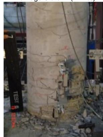
Damage State VI (6.97%)
