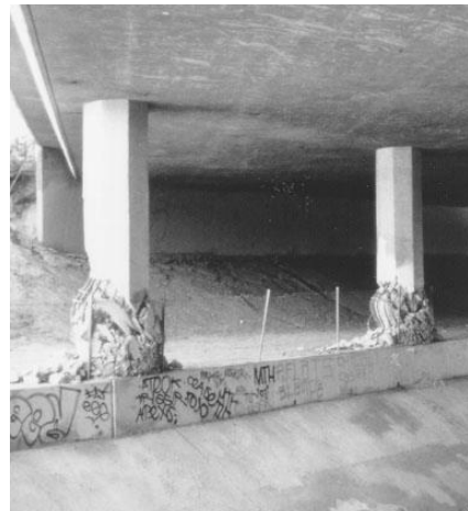
(b) Bull Creek Canyon Channel Bridge Damage in the 1994 Northridge EQ. (Moehle & Eberhard, 2000)
