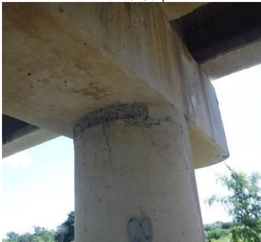
(g) Bridge 2401 Damage at Column Top in the Jan. 2020 Puerto Rico EQ, Built in 1996 (Photo by Dr. Manuel Coll)
