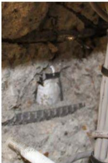
Damage State IV (4.3%)
