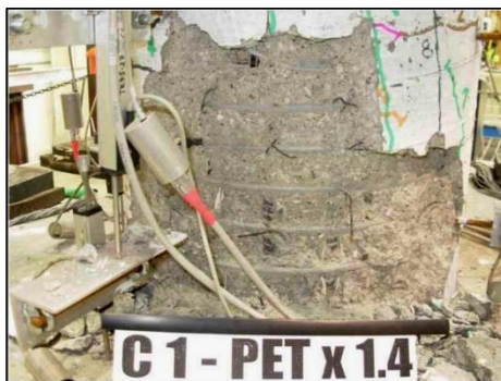
Damage State IV (9.15%)
