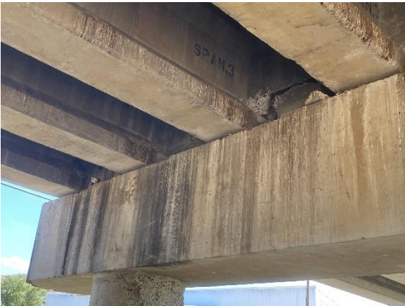
(d) Bridge 2401 Damage at Bent Top in the Jan-March 2020 Puerto Rico EQs, Built in 1996 (Photo by Dr. Manuel Coll)
