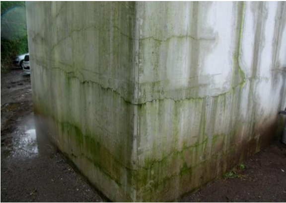
(b) Okirihata Oh-hashii Bridge Damage in the 2016 Kumamoto EQ., Built in 2001 (Istrati, 2016)
