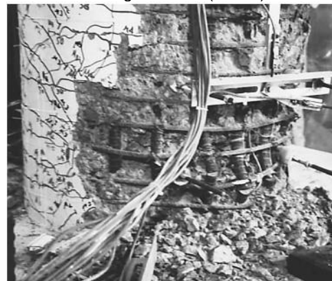
Damage State V-VI (8.7%)
