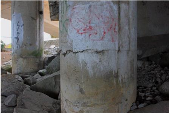
(a) Llacolen Bridge Damage in the 2010 Maule EQ, Built in 2000 (Yen et al., 2011)
