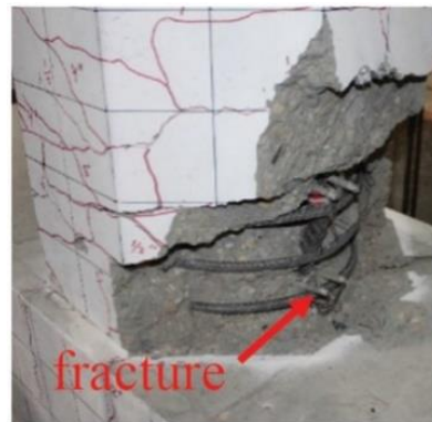
Damage State III
