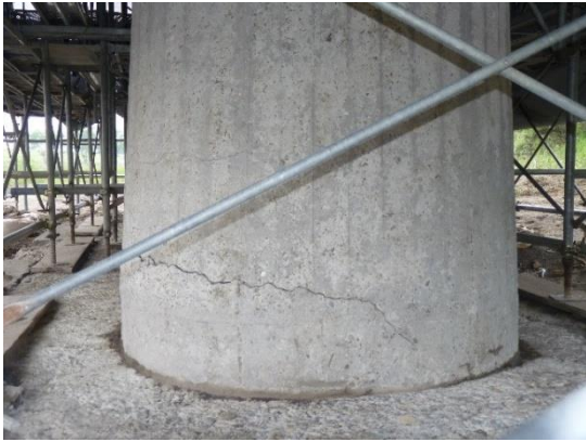
(e) Shida Hashi Bridge Cracks at Column Base in the 2011 Tohoku EQ, Built in 1957 (EERI, 2011)
