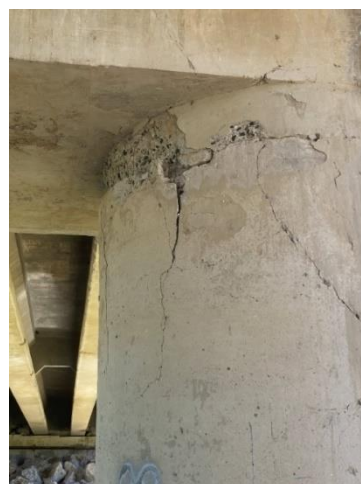
(h) Bridge 2401 Damage at Column Top in the March 2020 Puerto Rico EQ Built in 1996 (Photo by Dr. Manuel Coll)
