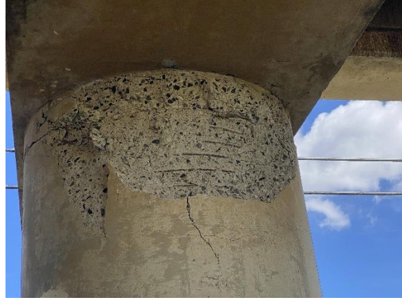
(f) Bridge 2401 Damage at Column Top in the March 2020 Puerto Rico EQ, Built in 1996 (Photo by Dr. Manuel Coll)
