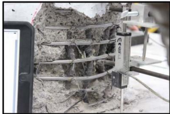
Damage State VI (6.92%)
