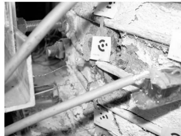
Damage State III
