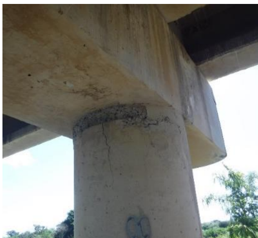
(g) Bridge 2401 Damage at Column Top in the Jan. 2020 Puerto Rico EQ, Built in 1996 (Photo by Dr. Manuel Coll)
