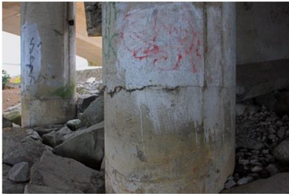
(a) Llacolen Bridge Damage in the 2010 Maule EQ, Built in 2000 (Yen et al., 2011)
