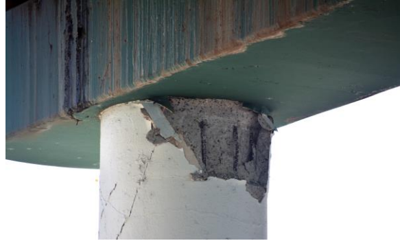
(l) Bridge PR-2 Mayagüez Damage at Column Top in the Jan. 2020 Puerto Rico EQ, Built before 1980 (Photo by Wallace J. de la Vega)
