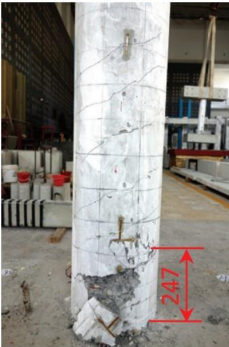
Damage State IV (2.79%)
