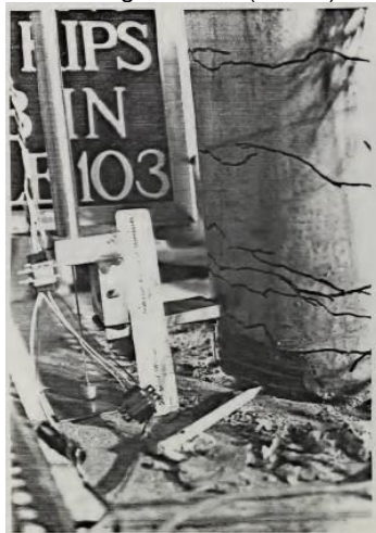
Damage State IV (6.44%)
