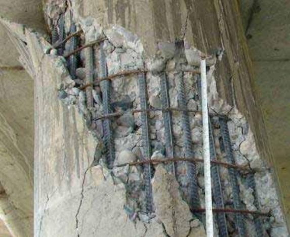
(c) Mianyang Airport Viaduct, Short Column Damage in the 2008 Wenchuan EQ, Built in 2001 (Yen et al., 2011)
