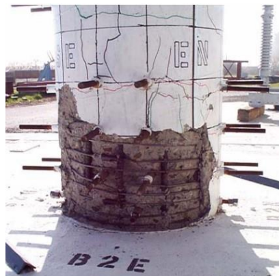
Damage State VI (Both later runs to 5.82%)
