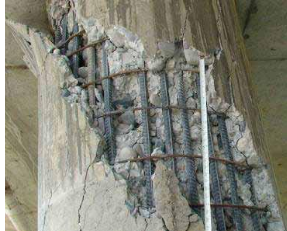
(b) Mianyang Airport Viaduct, Short Column Damage in the 2008 Wenchuan EQ, Built in 2001 (Yen et al., 2011)
