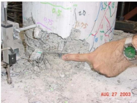
Damage State IV (5.52%)
