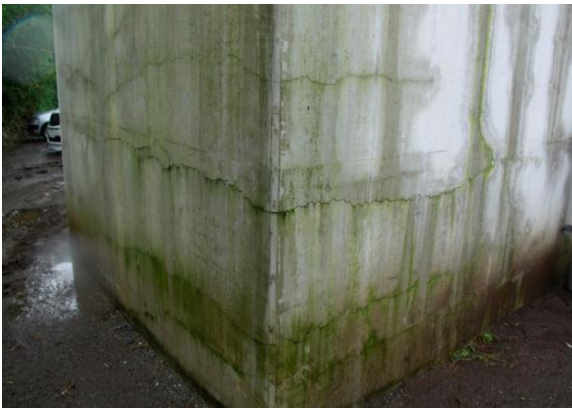
(c) Okirihata Oh-hashii Bridge Damage in the 2016 Kumamoto EQ., Built in 2001 (Istrati, 2016)
