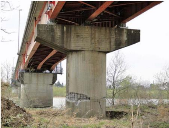
(g) Fuji Bridge Damage with Insufficient Development in the 2011 Tohoku EQ, Built before 1990 (Kawashima and Buckle, 2013)
