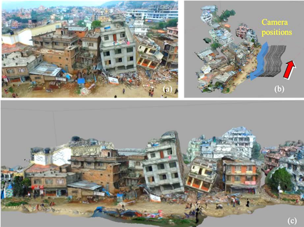
(a) Snapshot of Video Footage, (b) Estimated Camera Positions, (c) 3D model of the district Figure 2.30 – 3D Reconstruction of a District in Sitapaila, Kathmandu, Nepal (Yamazaki et al., 2015)
