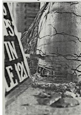
Damage State VI (7.73%)
