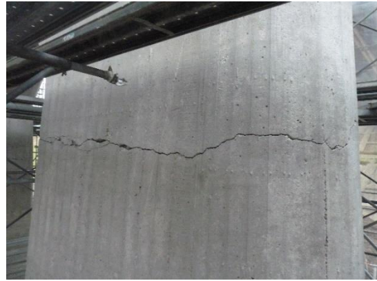
(f) Shida Hashi Bridge Cracks at Column Top in the 2011 Tohoku EQ, Built in 1957 (EERI, 2011)
