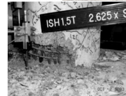
Damage State V (5.16%) & VI (5.8%, 6.03%)
