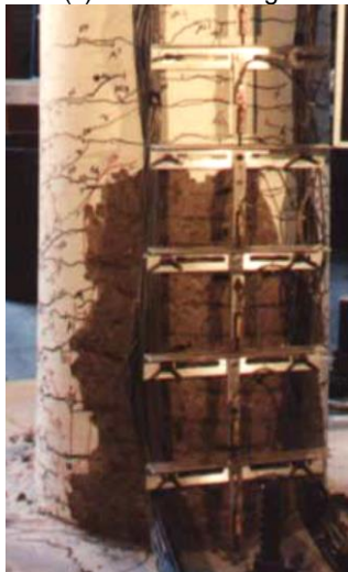
(e) Level IV Damage
