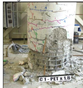
Damage State V & VI (14.89%)
