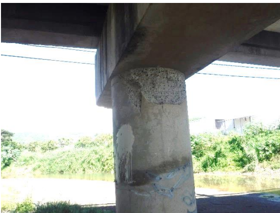
(e) Bridge 2401 Damage at Column Top in the Jan. 2020 Puerto Rico EQ, Built in 1996 (Photo by Dr. Manuel Coll)
