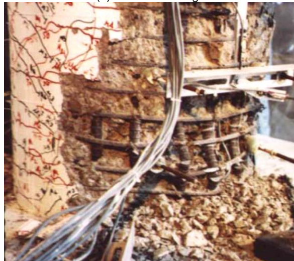
(f) Level V Damage
