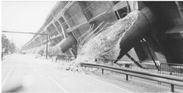
(a) Higashi-Nada Viaduct Collapse in the 1995 Hyogo-Ken Nanbu EQ (Chung et al., 1996)
