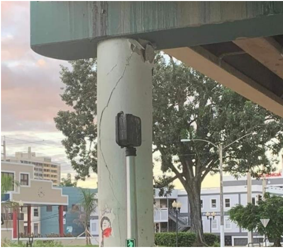
(k) Bridge PR-2 Mayagüez Damage at Bent Top in the Jan. 2020 Puerto Rico EQ, Built before 1980 (Miranda et al., 2020)
