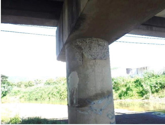
(e) Bridge 2401 Damage at Column Top in the Jan. 2020 Puerto Rico EQ, Built in 1996 (Photo by Dr. Manuel Coll)
