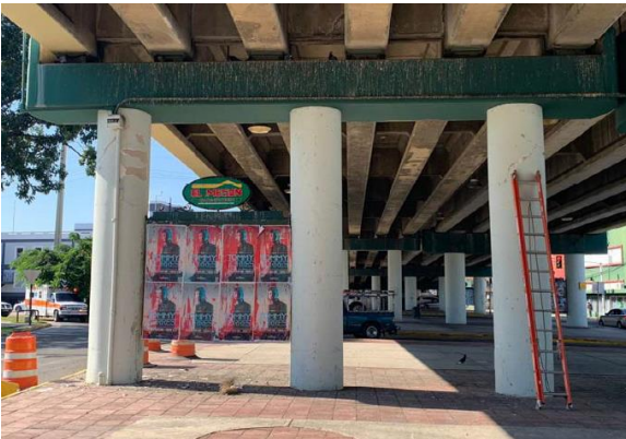
(i) Bridge 0729 Damage at Bent Top in the Feb. 2020 Puerto Rico EQ, Built in 1961 (Photo by Dr. Manuel Coll)
