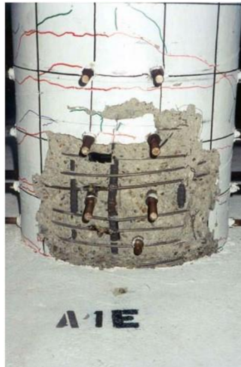
Damage State V-VI (7.8%)
