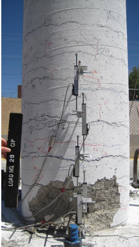
Cast-in-Place Column by Haber et al. (2013) Photo at Drift Ratio: 4.0% Column Height = 108 in. Diameter = 24 in.
