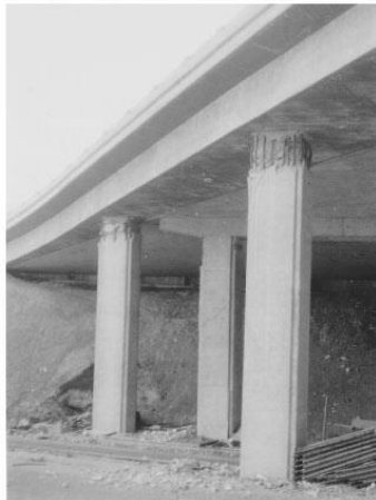
(c) San Fernando Road Overhead Damage in the 1971 San Fernando EQ (Moehle & Eberhard, 2000)
