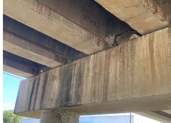
(d) Bridge 2401 Damage at Bent Top in the Jan-March 2020 Puerto Rico EQs, Built in 1996 (Photo by Dr. Manuel Coll)
