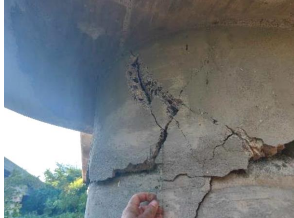
(n) Bridge 2417 Damage at Column Top in the Jan. 2020 Puerto Rico EQ, Built in 1961 (Miranda et al., 2020)
