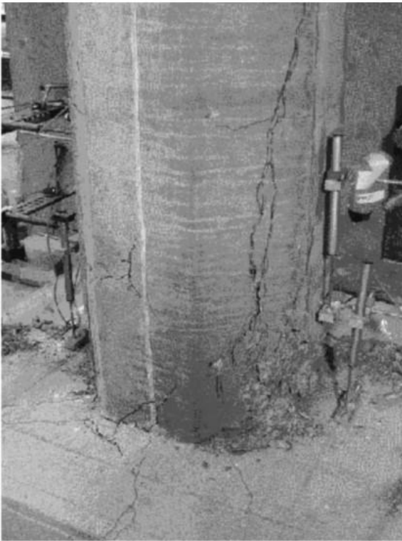
Damage State IV (4.5%)
