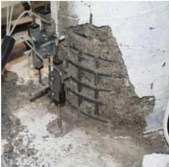
Damage State IV (8.89%)
