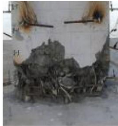
Damage State III
