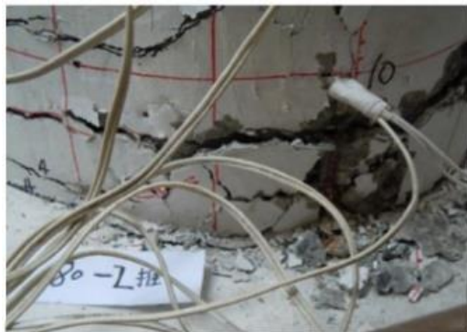
Damage State IV (5%)
