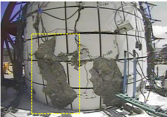
Full-Scale Column by Schoettler et al. (2015) Photo at Drift Ratio: 4.93% (EQ3) Column Height = 288 in. (324 with column head) Diameter = 48 in.
