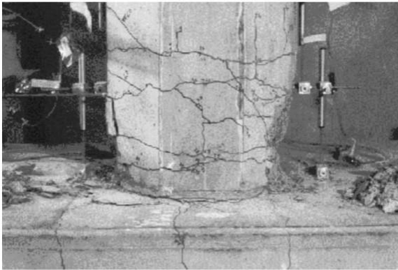
Damage State IV (4.5%)
