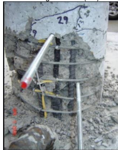
Damage State VI (10%)
