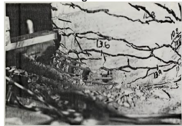
Damage State III
