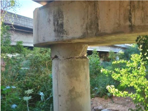
(m) Bridge 2417 Damage at Bent Top in the Jan. 2020 Puerto Rico EQ, Built in 1961 (Miranda et al., 2020)
