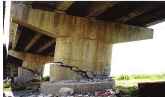
(h) Shear Failure of Pier Wall of the Wu-Shi Bridge in the Chi-Chi EQ (ACI 314.4R, 2016)
