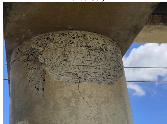
(f) Bridge 2401 Damage at Column Top in the March 2020 Puerto Rico EQ, Built in 1996 (Photo by Dr. Manuel Coll)
