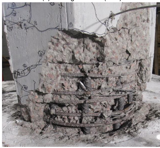
(f) Damage State 6 (DS6)
