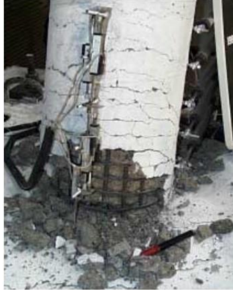
Damage State VI (23.61%)
