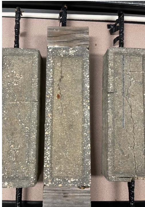
Figure 9. New set of reinforce concrete samples showing various levels of cracking due to corrosion. Note that each sample contains two rebars.
