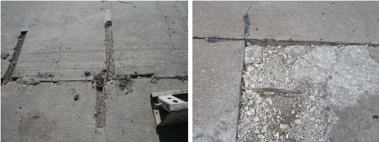
Figure 2.11- (a) Stapling failure due to slab expansion (left); (b) Failure of full-depth repair due to slab expansion (right)
