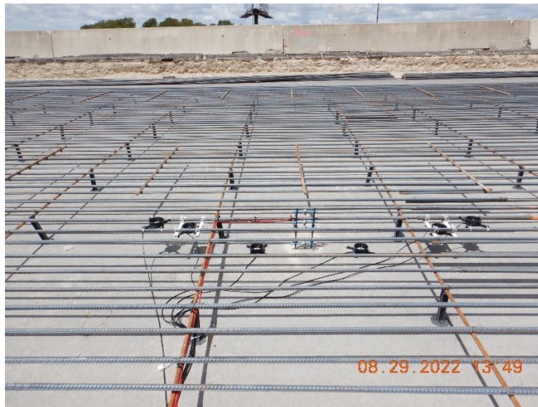
Figure 5.16 Actual gauge installation location at STA 212+00 in Hillsboro
