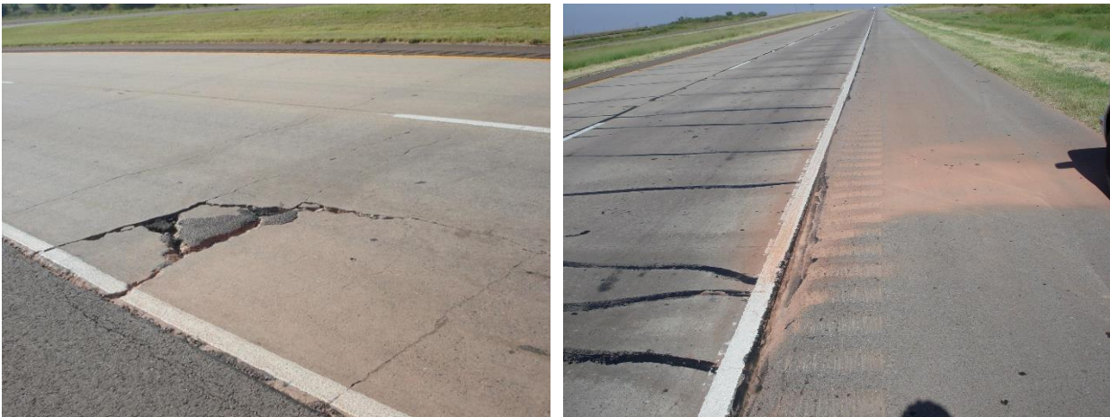
Figure 2.7-(a) Punchout distress on US 287 in Harrold (left); (b) Severe pumping on US 287 in Harrold (right)
