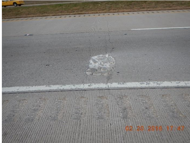
Figure 3.3 Distress caused by horizontal cracking on IH 20
