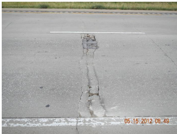
Figure 3.4 Distress caused by horizontal cracking on IH 35
