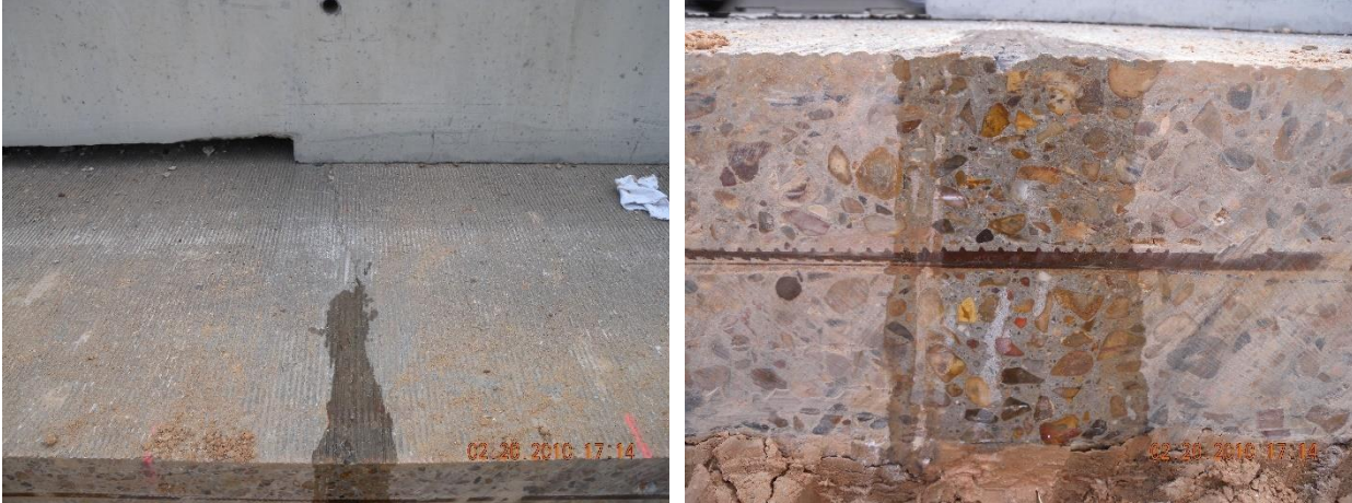
Figure 2.14- (a) Wide crack width on the slab surface (left); (b) Transverse crack profile through slab depth (right)
