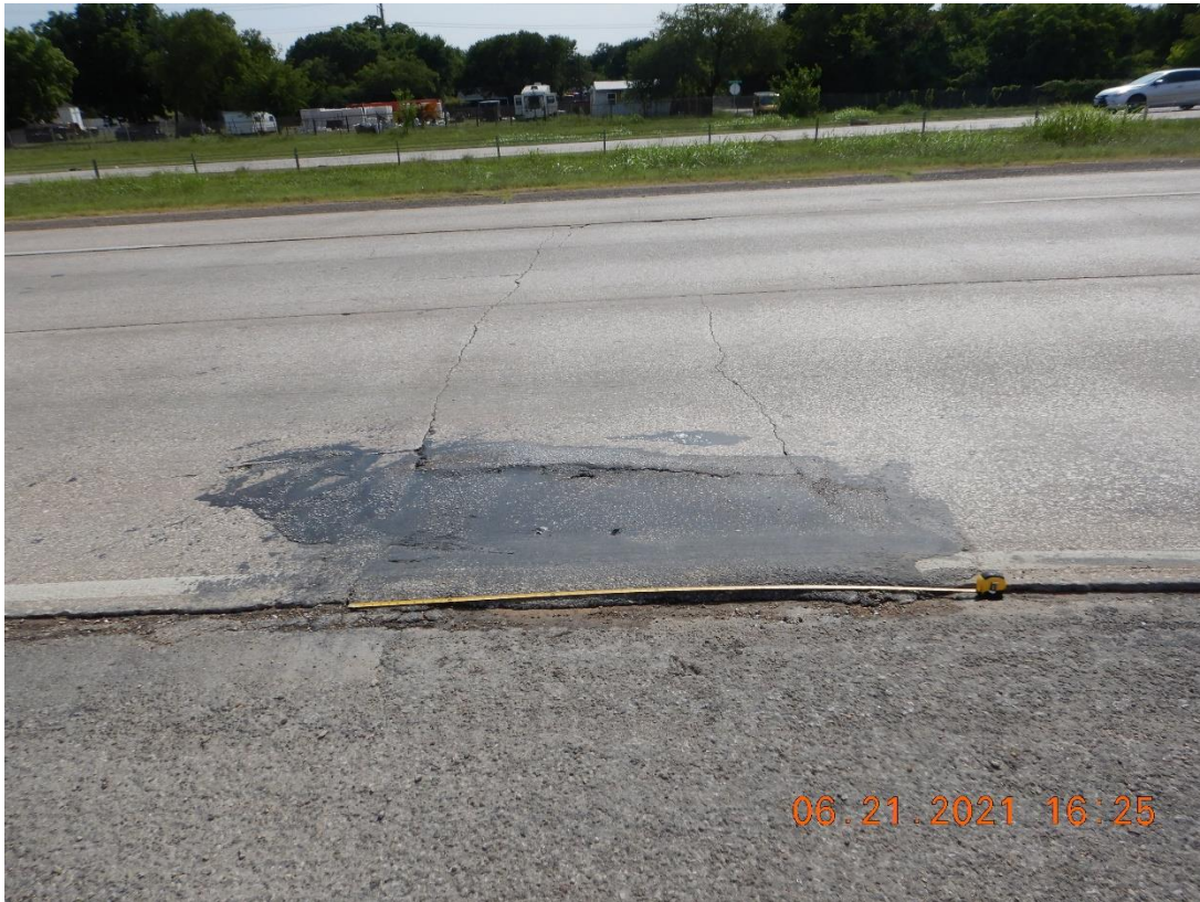
Figure 2.5 Punchout distress with a medium crack spacing
