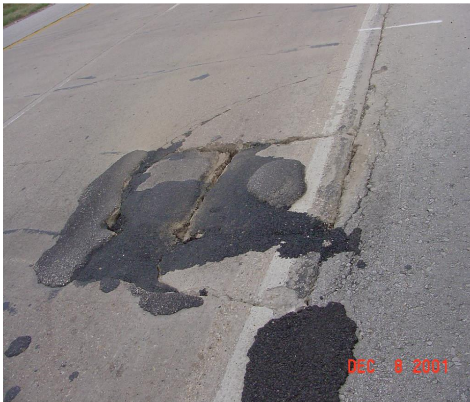
Figure 2.6 Punchout distress on IH-35W in Denton, Dallas District
