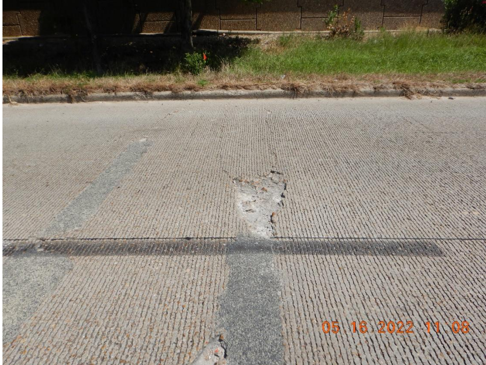
Figure 2.1 Typical spalling in CRCP observed in Texas
