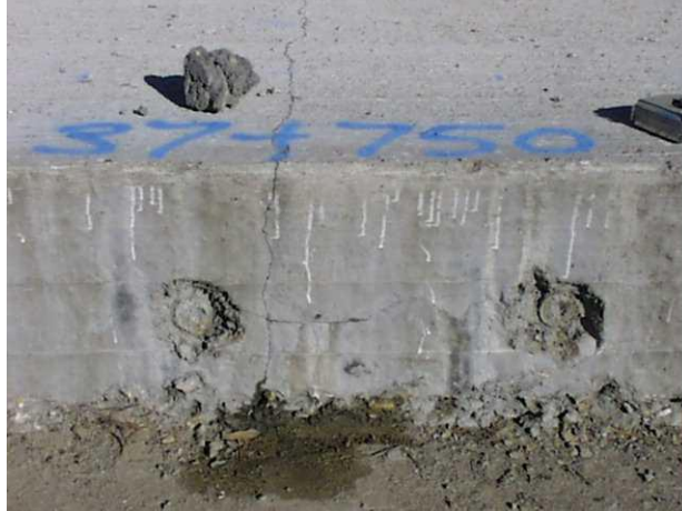
Figure 3.1 Horizontal cracking in new CRCP
