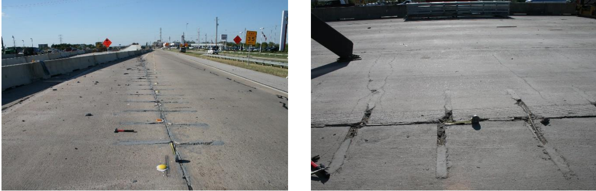
Figure 5.51 CRCP expansion and resulting stapling failure
