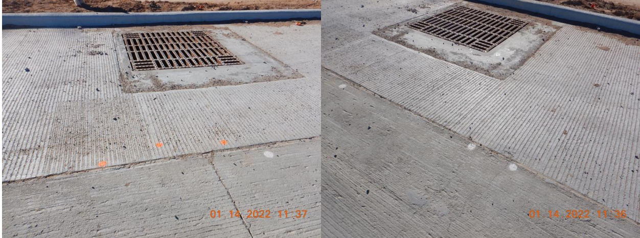
Figure 5.91 Development of reflection cracking at SC #1 from the drainage manhole
