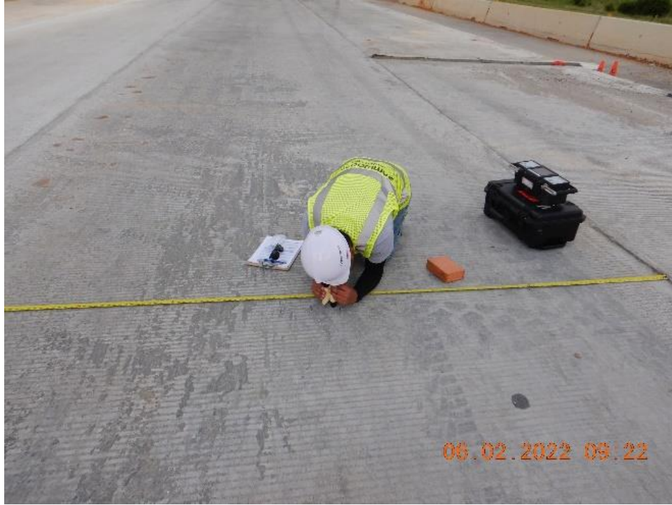
Figure 5.93 Investigation of crack widths in mid-depth and upper depth section in IH10 San Antonio
