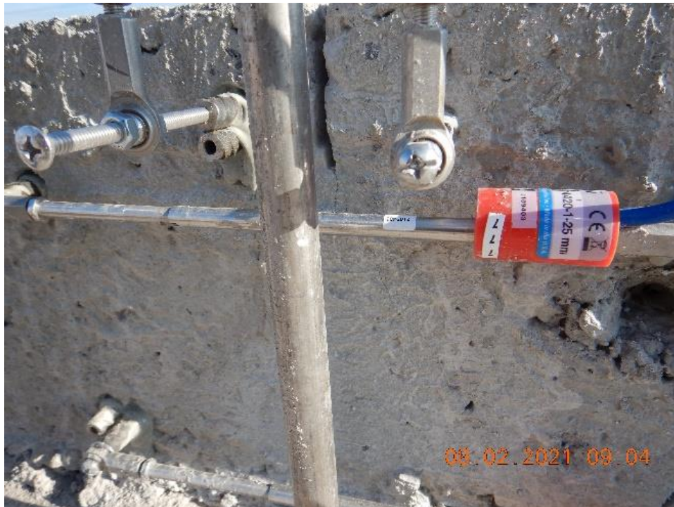
Figure 5.25 Crack propagation at the upper-depth section (2-2) in US62/180 El Paso
