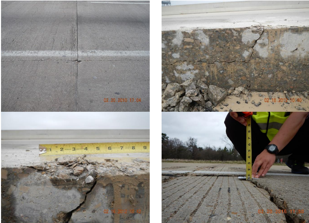
Figure 5.56 CRCP horizontal cracking observed in IH45 Dallas
