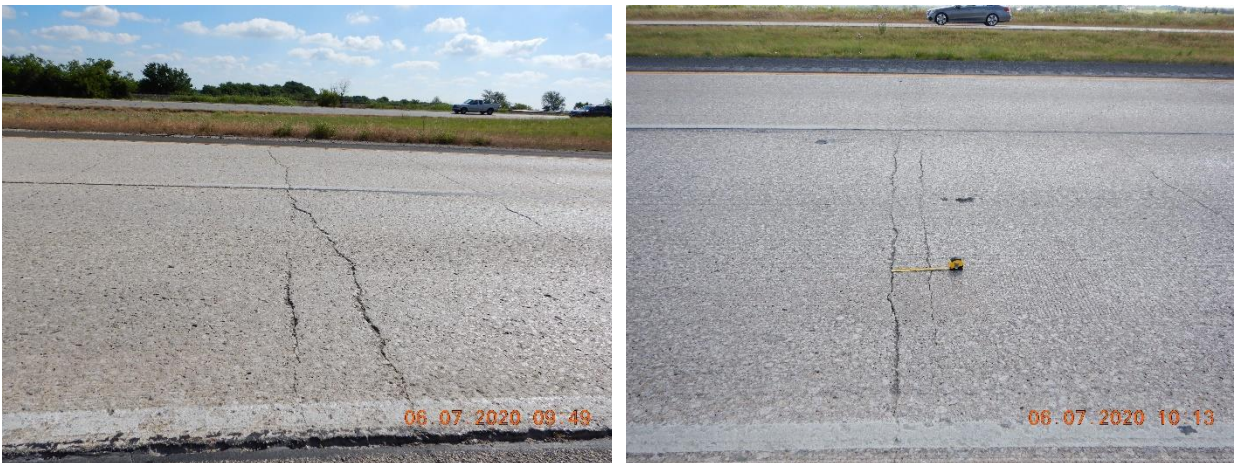
Figure 2.4- (a) Y-crack with no distress (left); (b) Short crack spacing (right)
