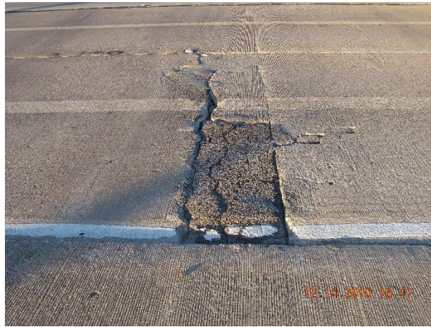
Figure 2.17 Typical distress at TCJ
