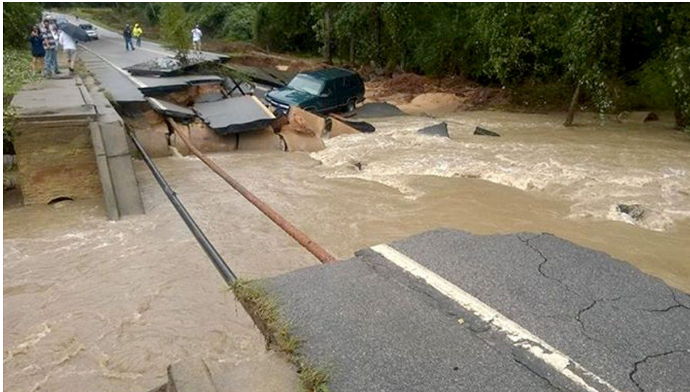
Figure 1.1 On October 4, 2015, flooding occurred on Caughman Road in Richland County [3]
