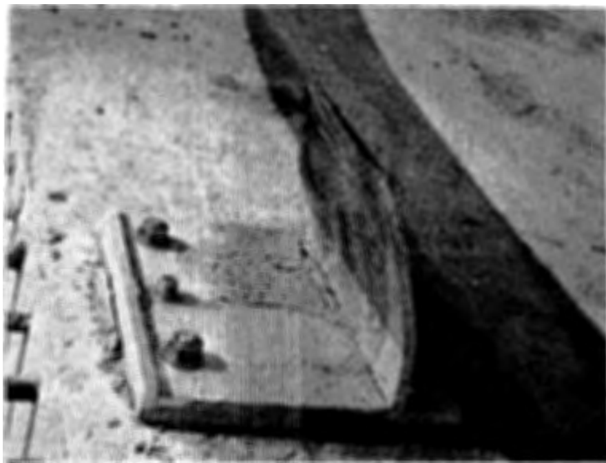
Figure 58. Sheared Rivets on Post Mountings After Test 4182-2 (Ref. 15).
