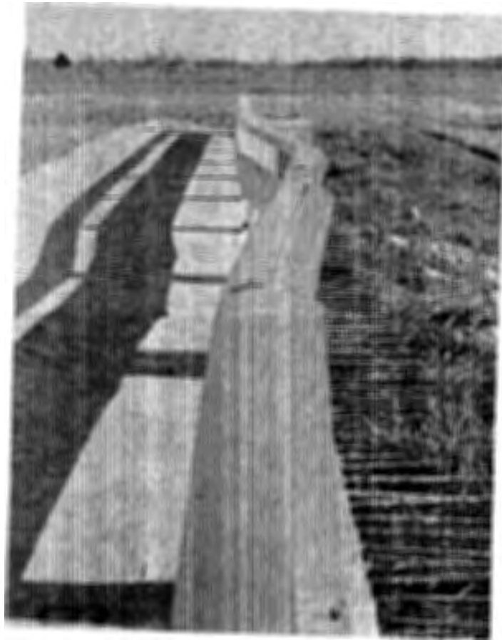
Figure 60. Damage to Railing After Test 4182-3 (Ref. 15).
