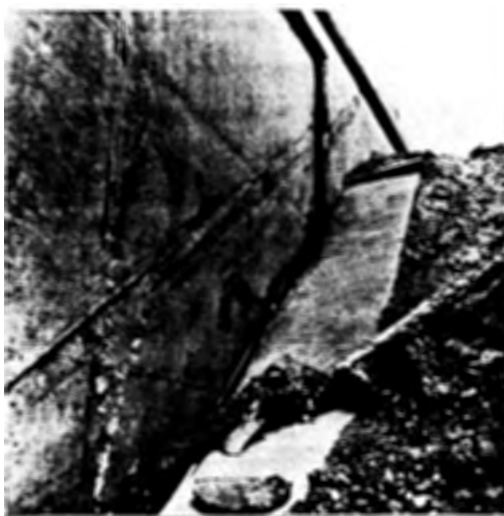
FIGURE 18. ABUTMENT AND APPROACH FILL SETTLEMENT— SAN FERNANDO EARTHQUAKE, 1971
