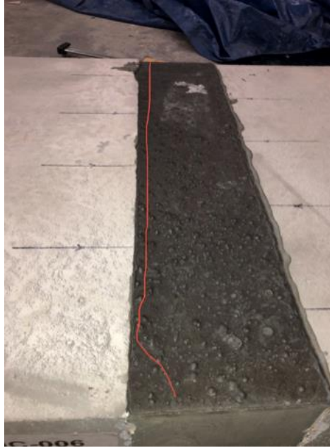
Figure 168. Photo. Location of shrinkage crack in specimen G-9-5.0-B.
