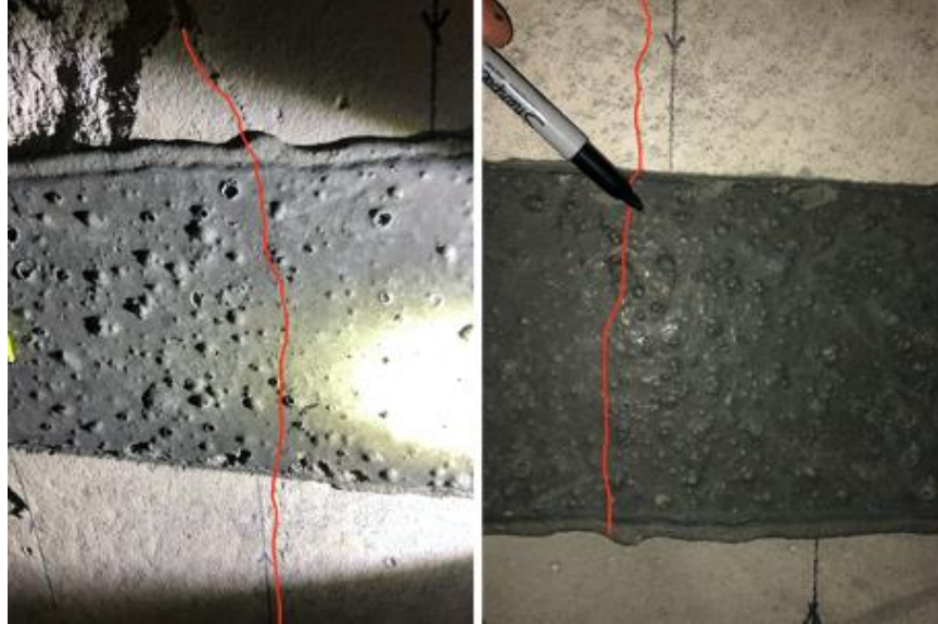
Figure 178. Photo. Thin cracking in UHPC joints propagation from precast panels.
