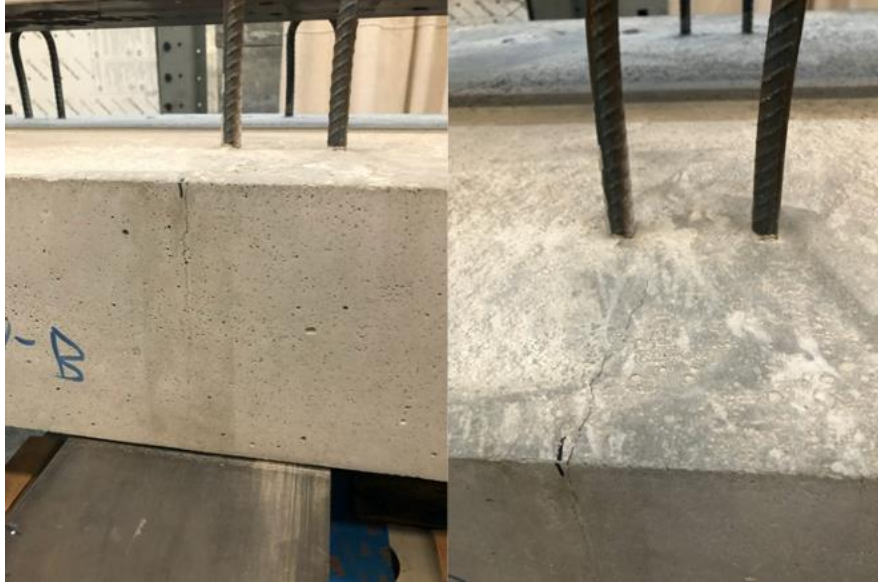
Figure 113. Photo. Cracks near supports in the precast panels at load P_{cr} .
