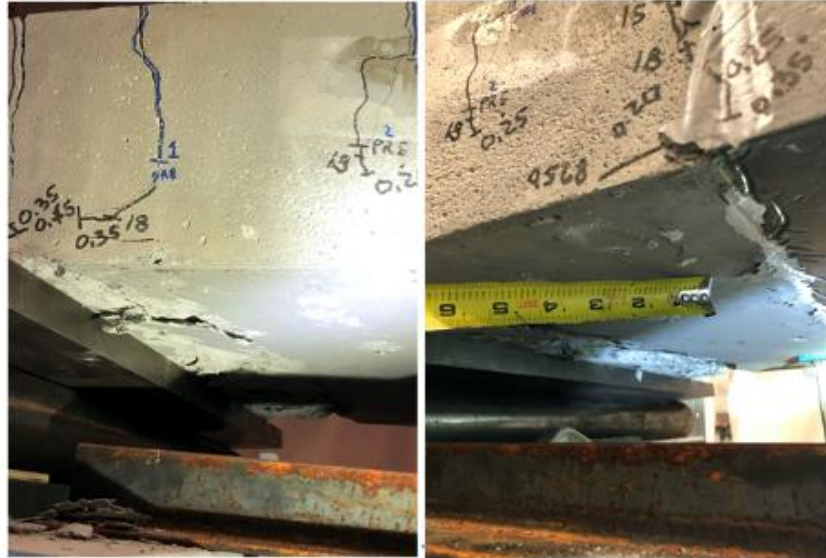
Figure 141. Photo. Concrete from precast concrete crushing under supports and against UHPC joint.
