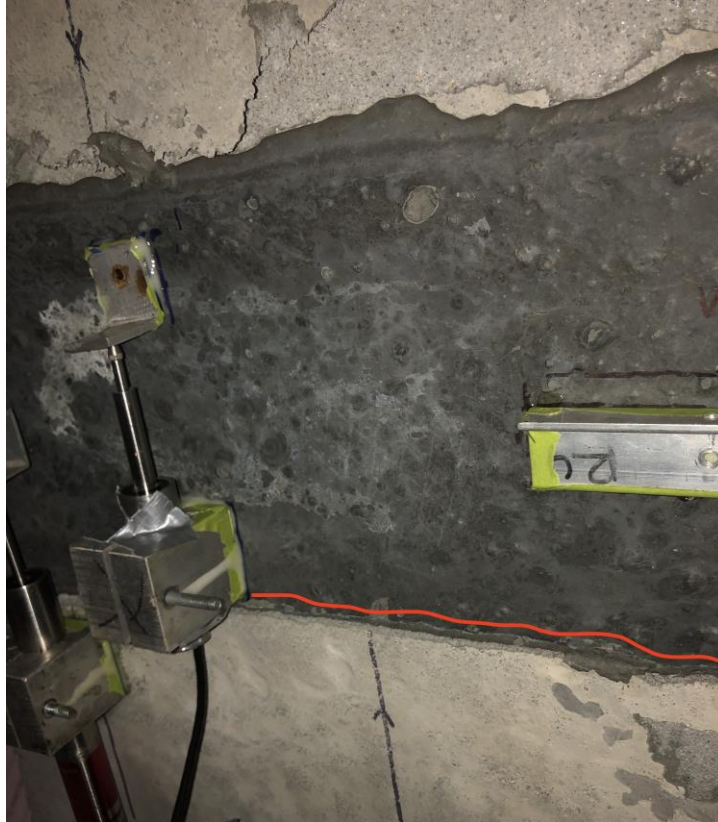
Figure 180. Photo. Shrinkage crack during loading.
