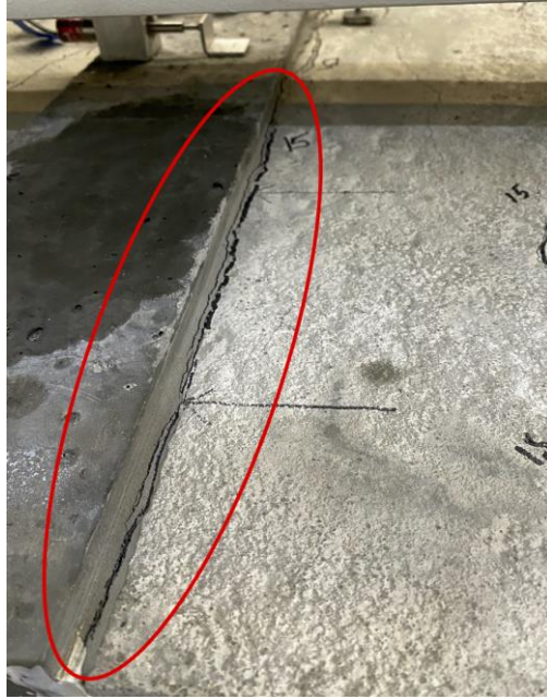
Figure 103. Photo. Wider crack observed at the interface at M_u .
