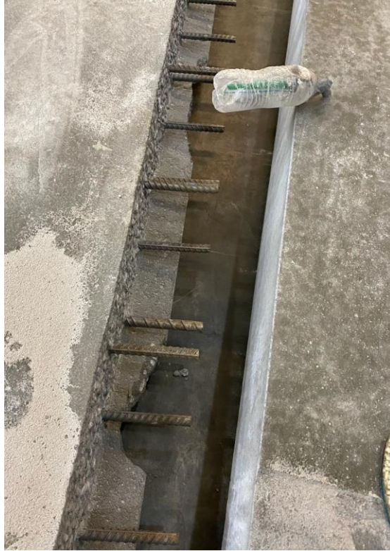
Figure 89. Photo. Damage to GDOT specified joint detail during transport.
