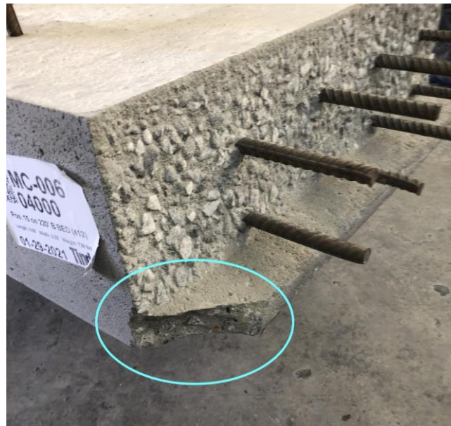
Figure 147. Photo. Damage caused to shear key during shipping of panels.
