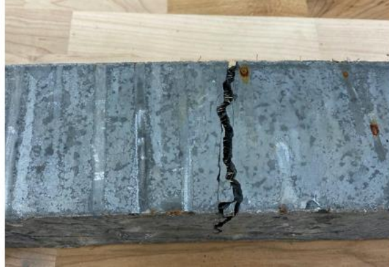
Figure 68. Photo. Close-up of the major crack in the 3 in. by 3 in. beam.
