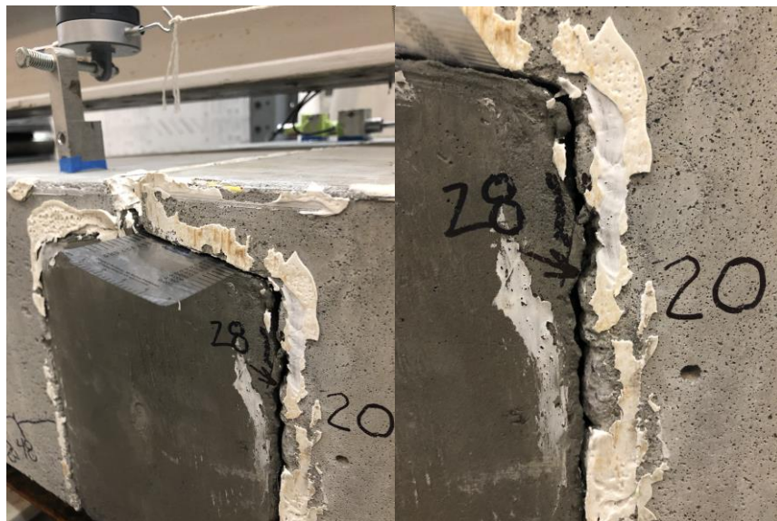
Figure 162. Photo. Close-ups of large gap between shear key and UHPC joint caused by cold joint.
