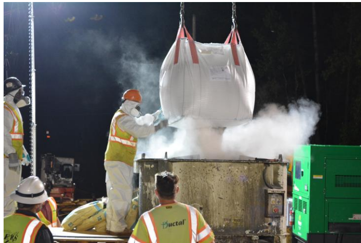
Figure 34. Photo. UHPC being mixed in a high-shear pan mixer in the field.
