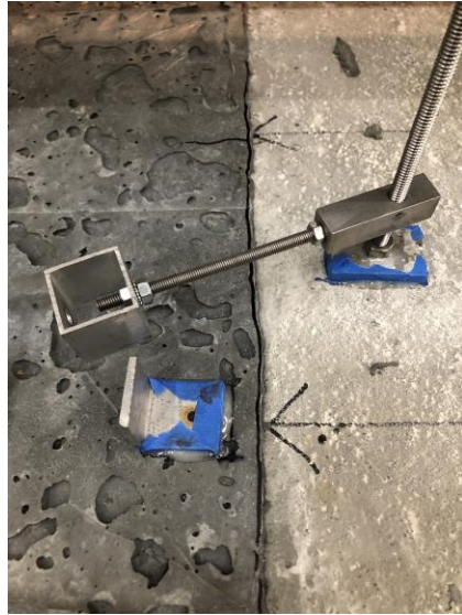
Figure 132. Photo. Pre-test crack at UHPC and precast concrete interface.
