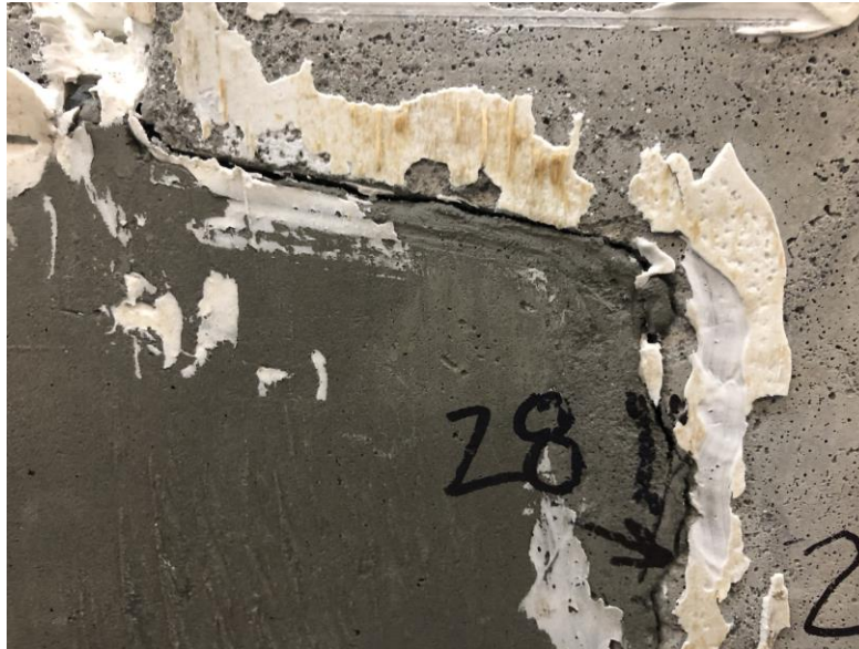
Figure 155. Photo. Gap formation between precast concrete panel shear key and UHPC joint at 38 kips.
