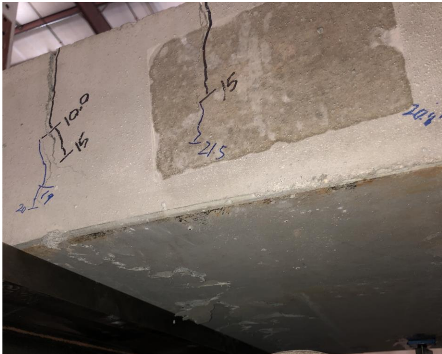
Figure 122. Photo. Crushing of precast concrete under west support.
