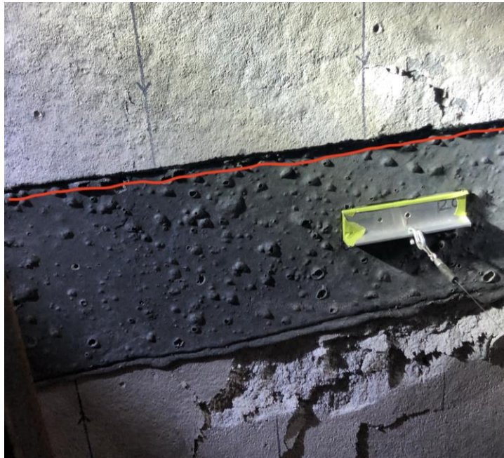
Figure 181. Photo. Concrete crushing on side opposite shrinkage crack.
