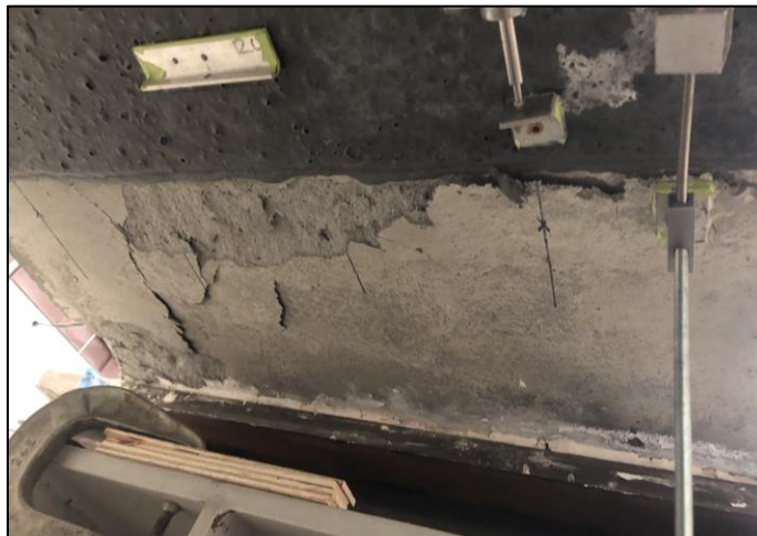
Figure 175. Photo. Crushing on precast panel at failure.
