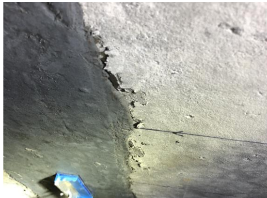
Figure 160. Photo. Crushing of precast concrete panel against UHPC.
