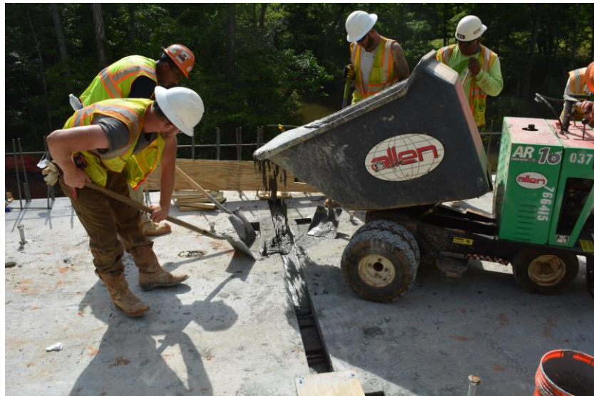
Figure 22. Photo. Workers fill a transverse joint on the County Road 131 Bridge with UHPC.
