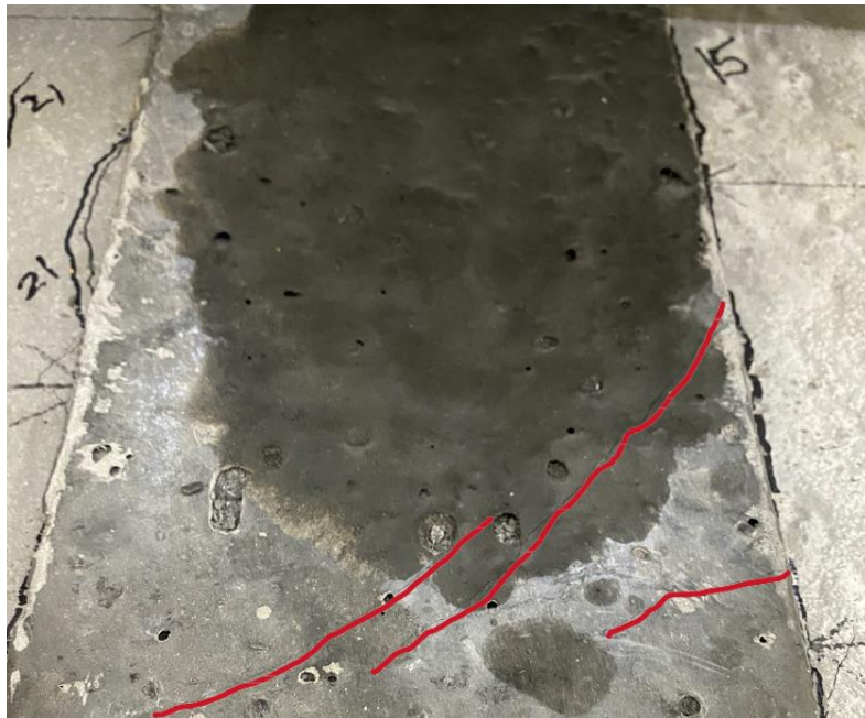
Figure 105. Photo. Top surface crack in UHPC at 1.3M_n .
