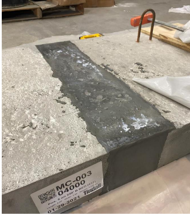
Figure 95. Photo. UHPC joint after 3 days of curing time and removal of formwork.
