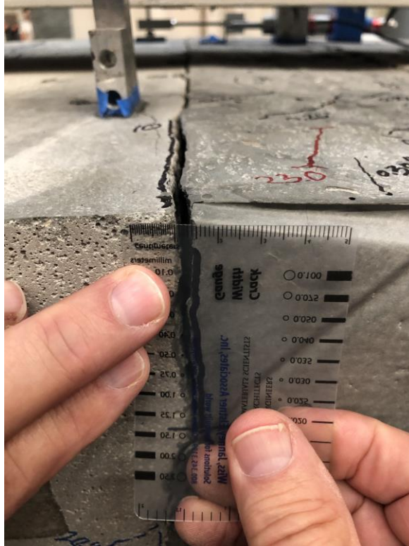
Figure 123. Photo. Measured crack width of crack at UHPC and precast concrete interface.
