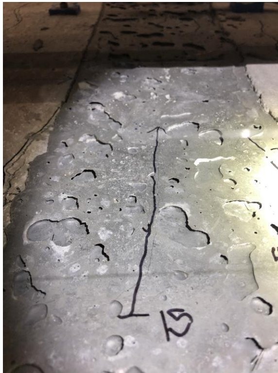
Figure 139. Photo. Close-up of tension crack in UHPC at a load of 17.6 kips.
