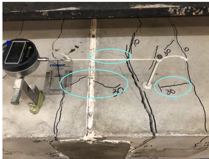
Figure 174. Photo. Horizontal cracking at 30 kips.
