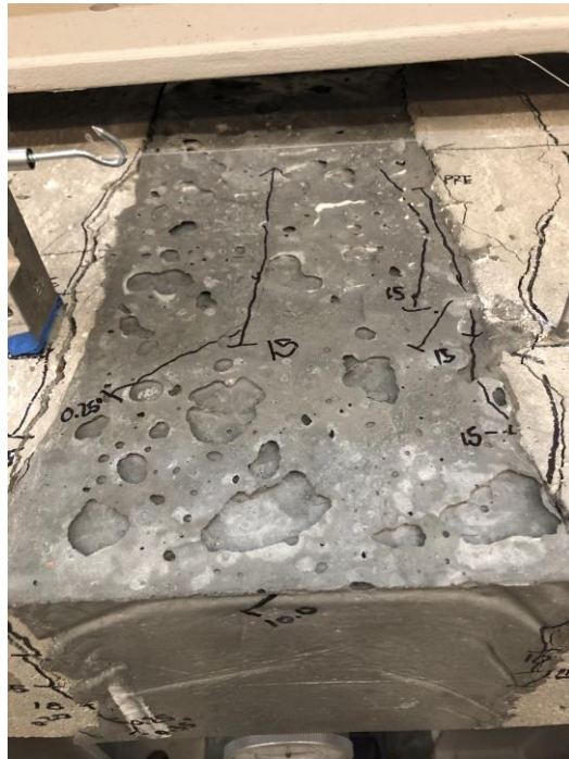
Figure 143. Photo. Cracking in UHPC region at failure.
