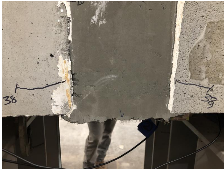
Figure 156. Photo. Horizontal cracking in precast concrete panels unmatched by the UHPC joint at 38 kips of applied load.
