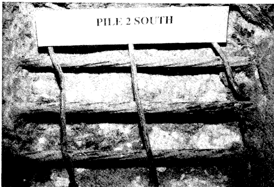
Figure 60. Appearance of uncovered tendons and reinforcing steel in south repair area, pile 2, after 215 weeks of tidal cycling.
