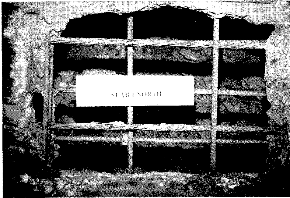
Figure 23. Appearance of uncovered tendons and reinforcing steel in north repair area, slab 1, after 100 exposure cycles.
