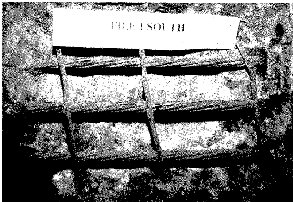
Figure 56. Appearance of uncovered tendons and reinforcing steel in south repair area, pile 1, after 215 weeks of tidal cycling.
