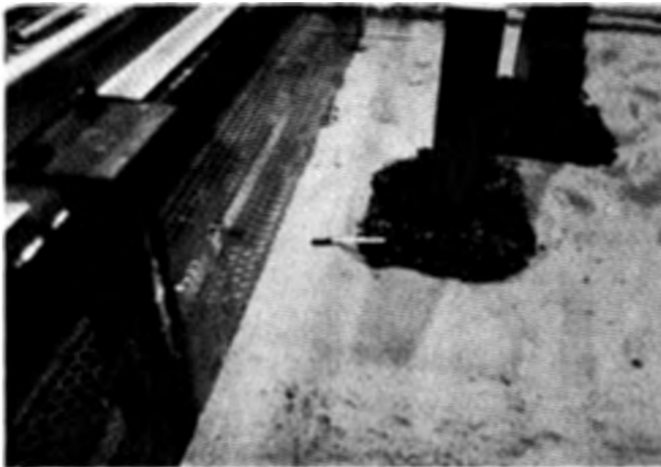
Figure 19. Scour around riprap.
