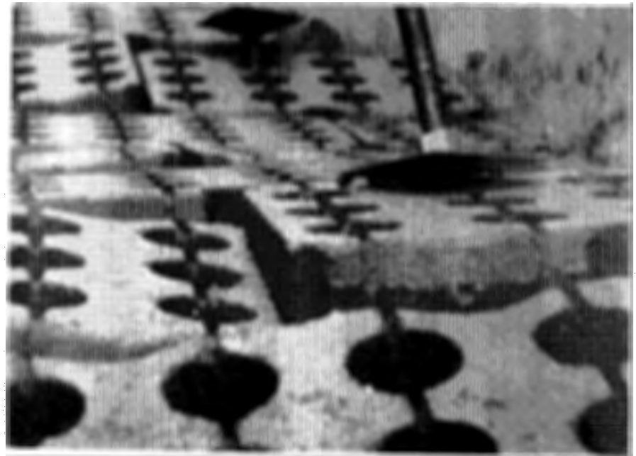
b. Block displacement due to uplift forces.
