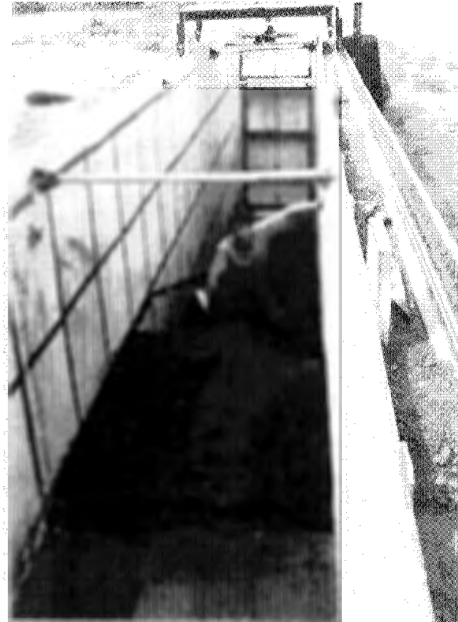
b. Looking downstream at the embankment crest. Note deformation of system near right wall.
