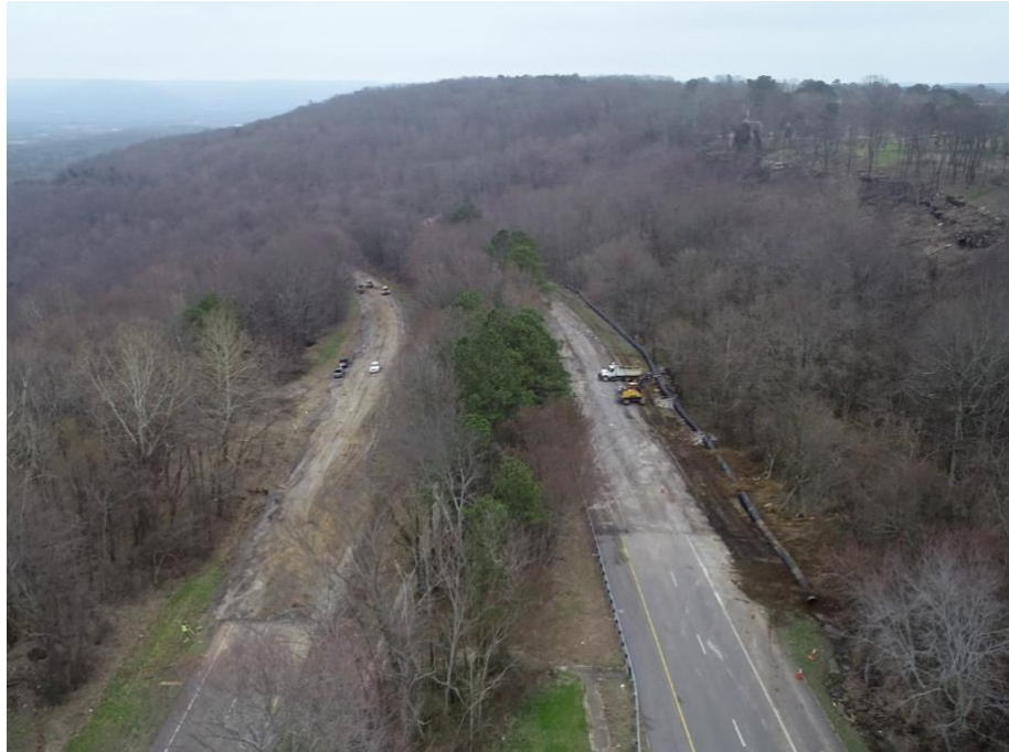
Figure 5-5: View of the slide area along US-231 after removal of the pavement. The geophysical survey team can be seen along the SB shoulder on the left side of the figure.
