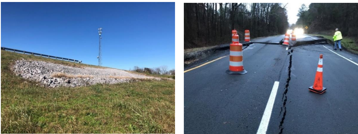
Figure 2-1: (Left) A repaired slope failure in an embankment section of SR-5 in Perry County and (right) cracking in the southbound lanes of US-231 near Laceys Spring following a large landslide in 2020.
