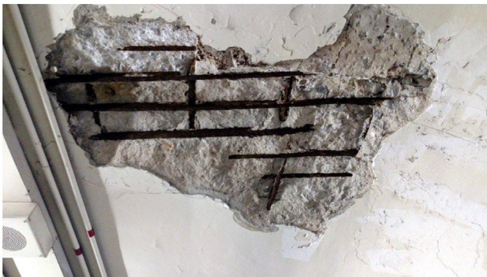
Figure 2-3 Example of spalling concrete from tunnel ceiling
