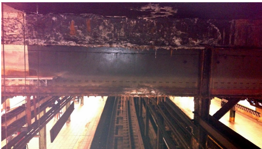
Figure 2-2 Example of leakage and corrosion on a beam (view from station)
