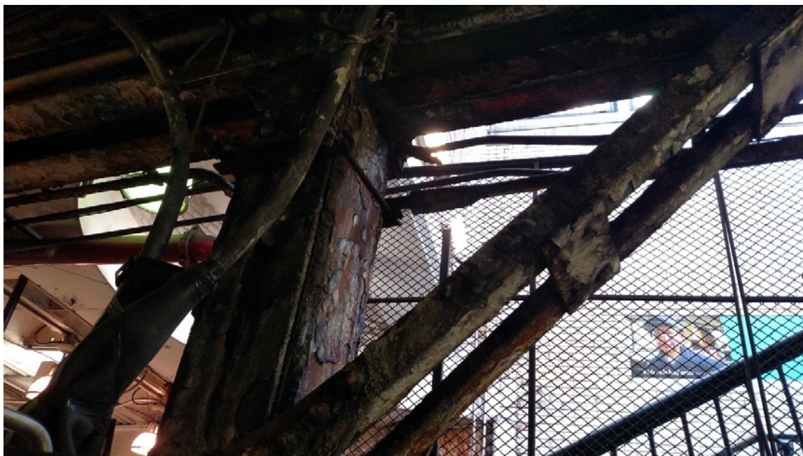
Figure 2-4 Example of deteriorated steel columns
